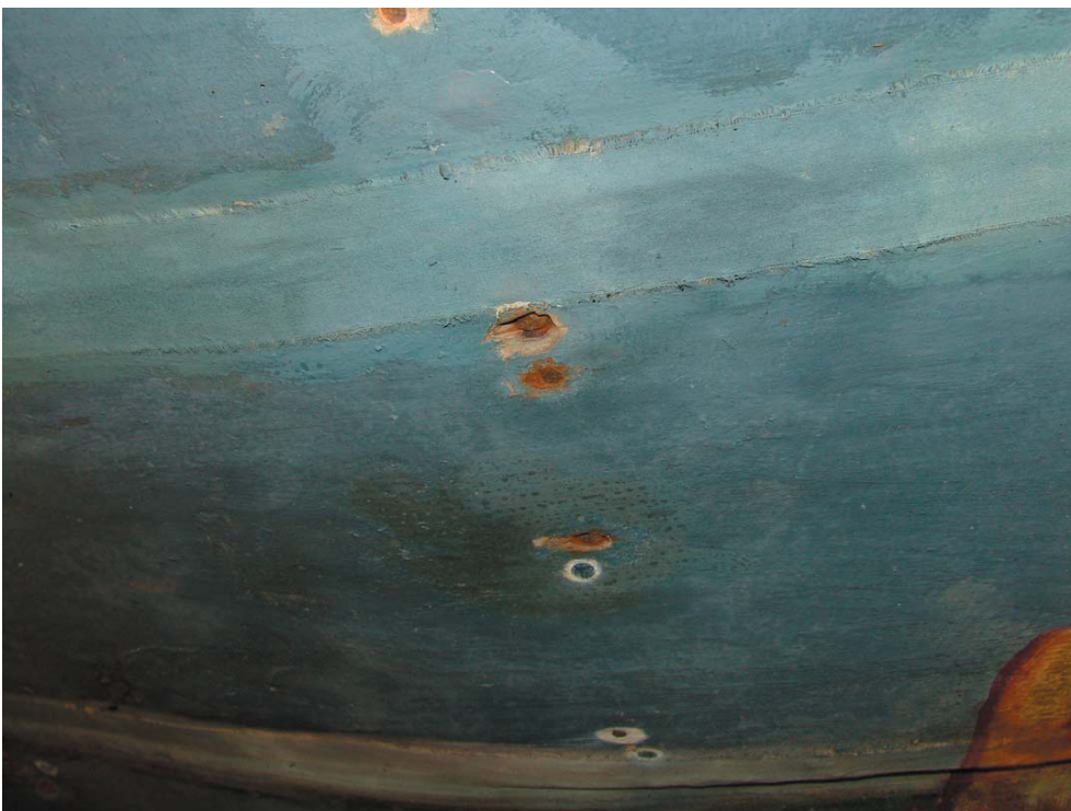
Plate 27 (below). Throughout the ceiling there were over 3500 rusting nails that required treatment. (Photo: Paine and Stewart 2006)
