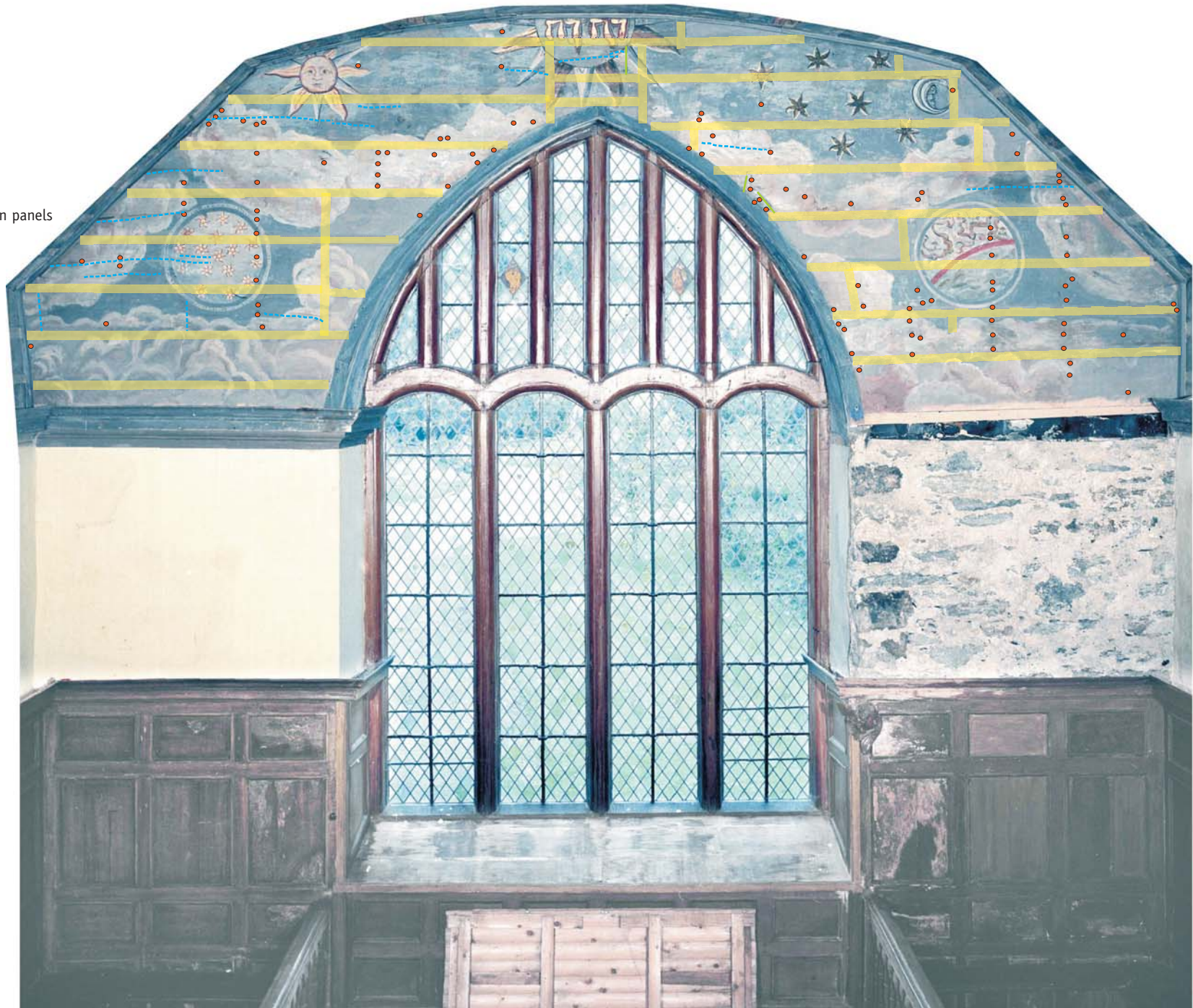
Figure 2: overall photograph of the east wall decoration, showing aspects of condition
