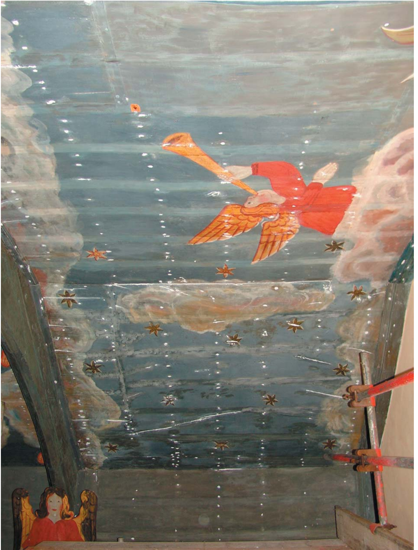
Plate 28 (above). General view of the western end of the ceiling, showing work in progress, with multiple nail heads treated, filled and awaiting final retouching, (Photo: Paine and Stewart 2006)
