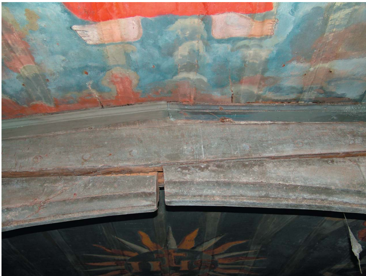
Plate 34 (above). The trusses displayed significant areas of blanching (probably resulting from previous coatings applied in the 1950s) and other unidentified disfiguring runnels, seen here prior to treatment.
