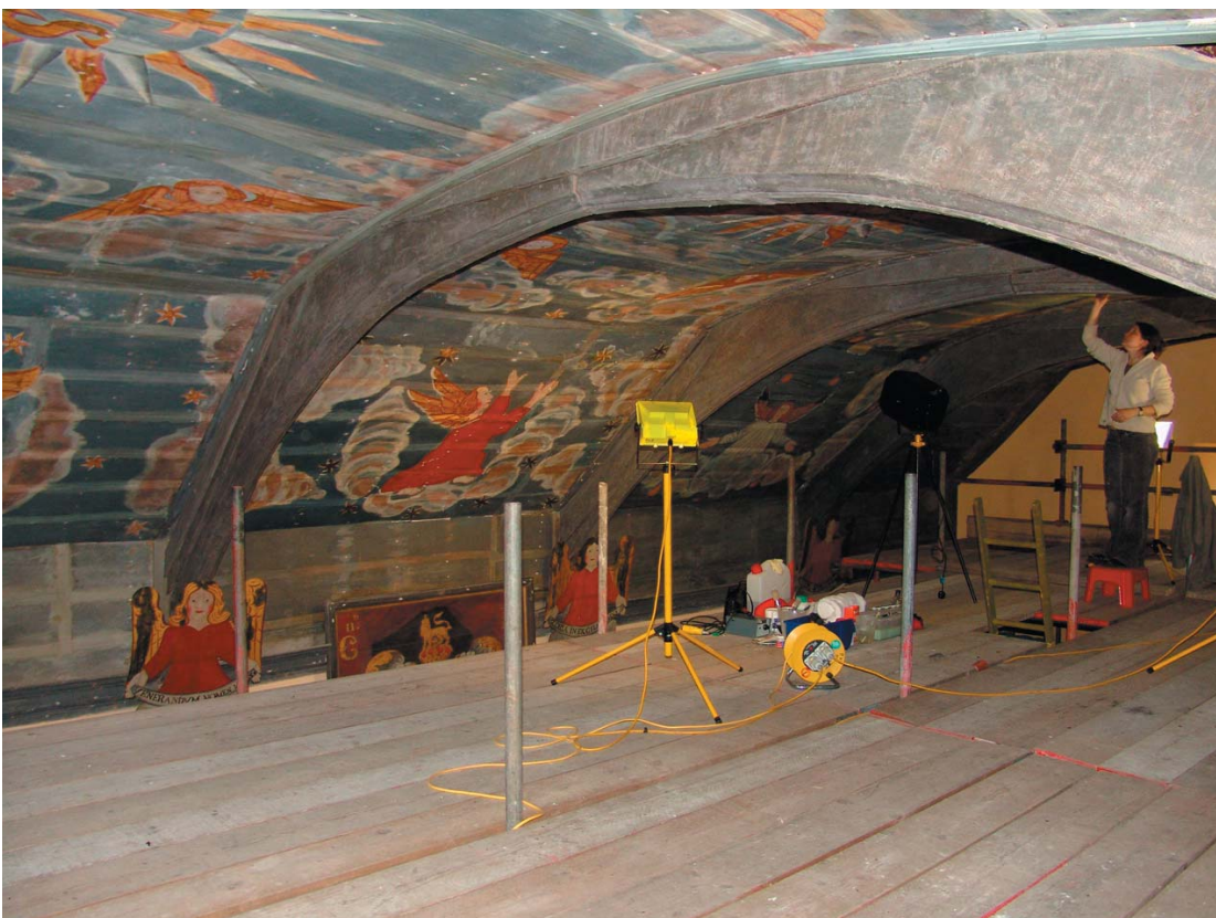
Plate 33 (below). Work in progress during the reintegration phase. (Photo: Paine and Stewart 2006)
