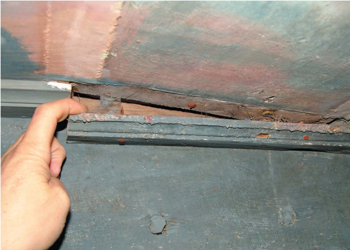
Plate 24 (above). While many of these edging strips (between ceiling planks and trusses) are replacements, the principal for such elements is probably an original one, since the decoration does not appear to extend beneath them. (Photo: Paine and Stewart 2006)
