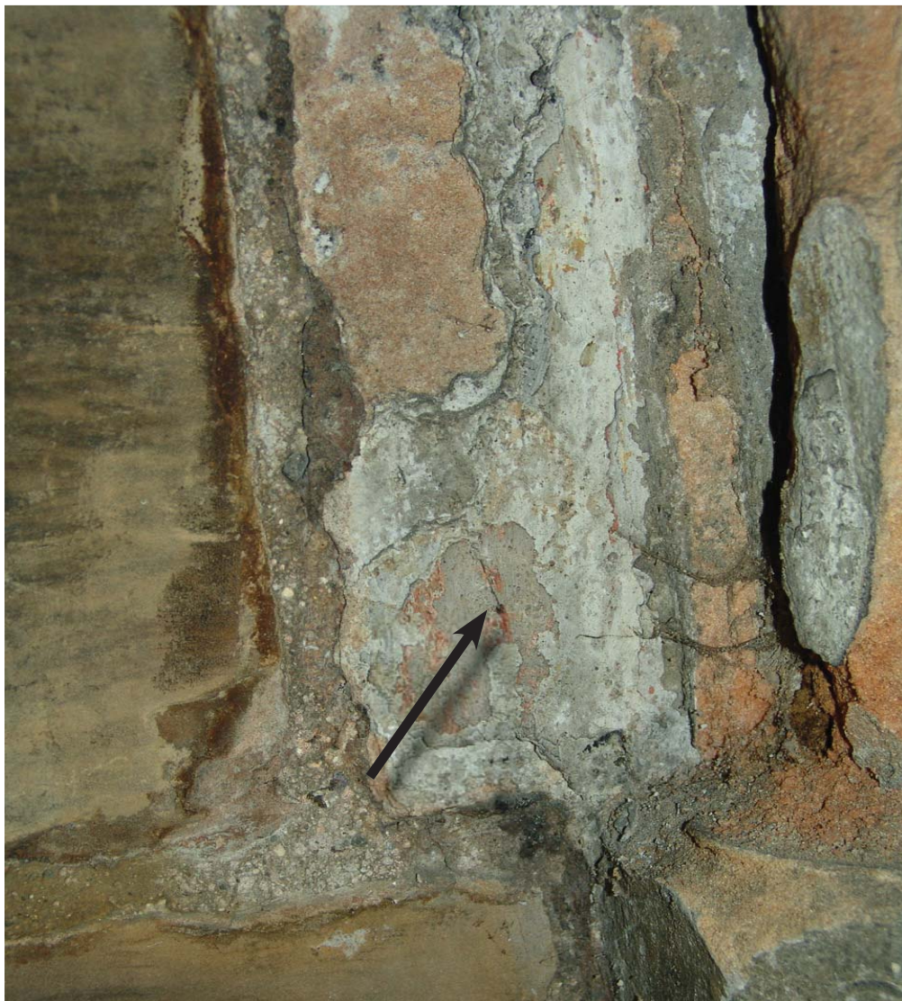
Figure 6. Sample site 3. South east corner springing of vault. Fragments of red pigment underlying later limewash layers can be noted. No discernible design could be noted, which is typical for the entire space.
