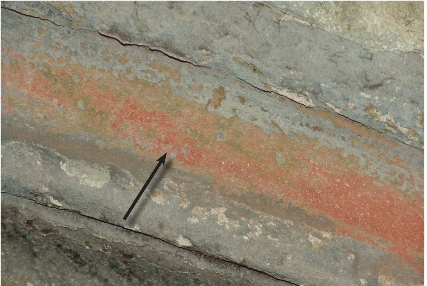
Figure 8. Sample site 4. West side of the central entry arch. Red and green colouration can be noted within the mouldings of the arch ribs.
