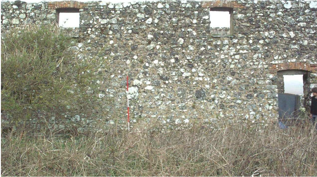
Skomer Island Farm outbuilding range: south wall exterior (east end), from south
