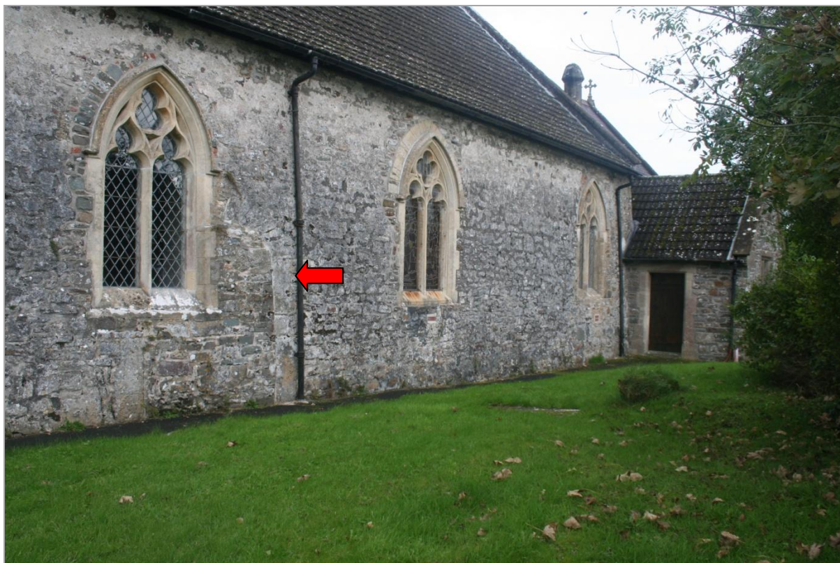
Looking northeast at the blocked doorway in the south wall of the nave of St Clears priory church. This doorway is believed to be the exit from the church into the claustral buildings.
