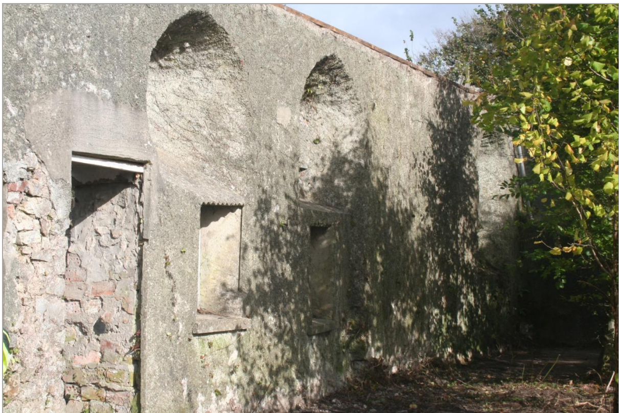
Looking north at the former internal face of the north wall of a medieval chapel, showing the three original blocked lancet windows.
