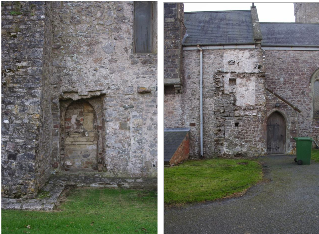
Photograph of the north side of Monkton Priory church showing the blocked doorway (left) and broken masonry (right) of where the nave and the northeast chapel respectively were attached to the former priory buildings.
