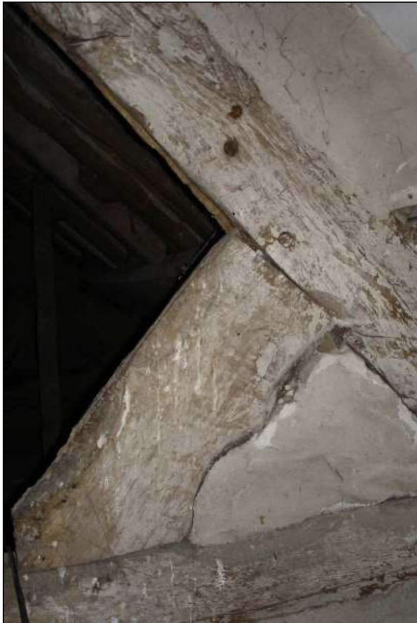
Figure 3: Detail of western side of reused cusped truss T2 showing ill-fitting joint to principal rafter
