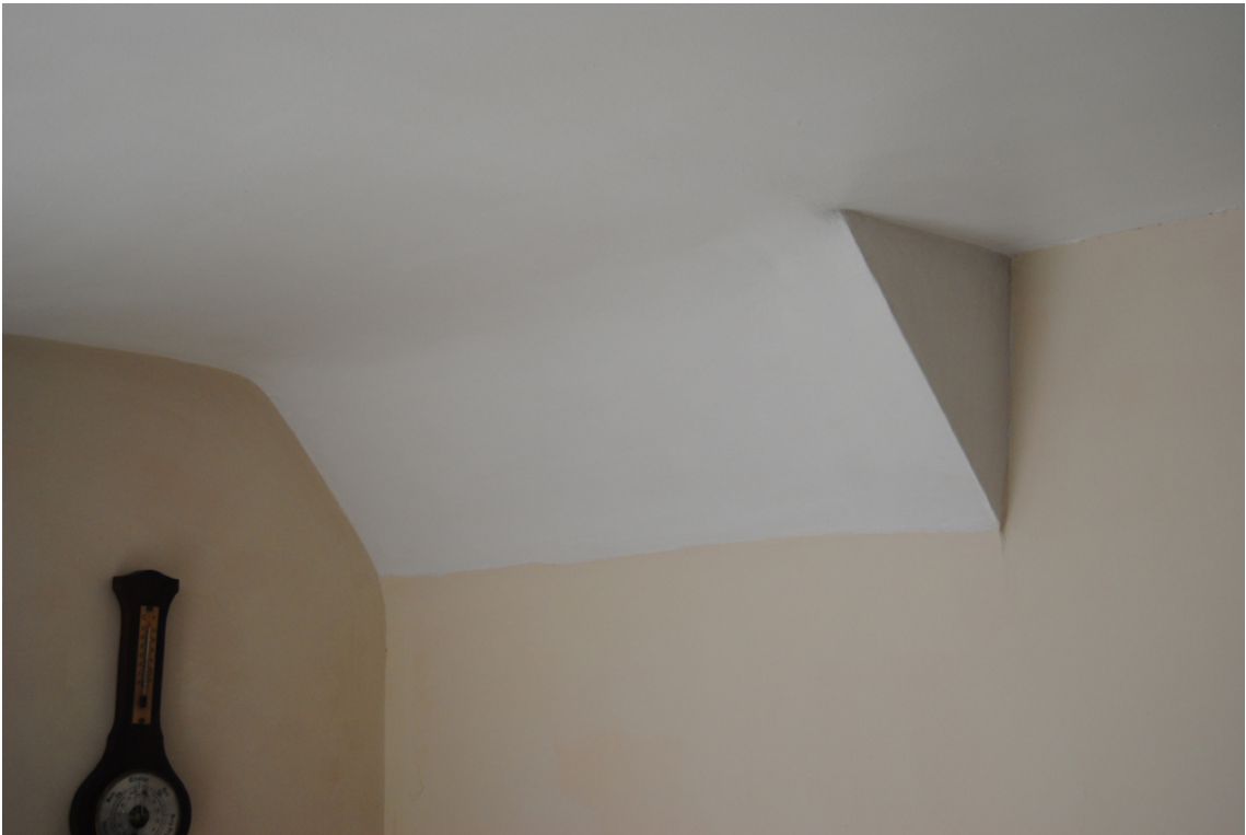
Plate 25: Sloping section of ceiling at south-east corner of [GF04] suggestive of former stair.
