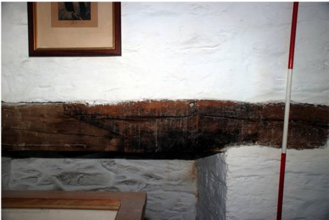
Plate 20: Detail of the repair to the bressumer over the fireplace in the northern gable.
