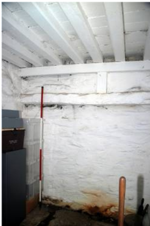
Plate 8: Timber across the northern gable end.
