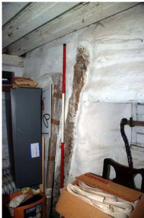
Plate 6: Timber embedded in the wall of the north east ground floor room
