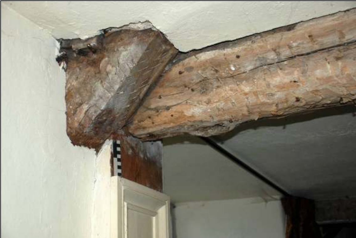
Plate 39: Relationship between the foot of Truss 5 and the tie beam, looking north
