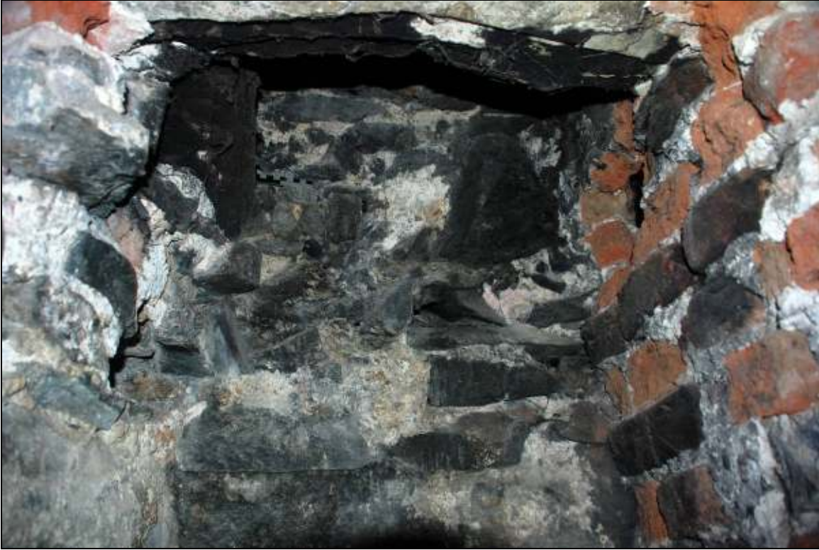
Plate 31: Sooting in stone lined channel on first floor tower room, looking up
