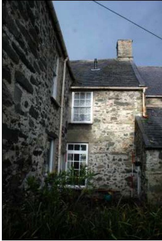
Plate 12: Possible blocked opening at northern end of the rear wall of the central range, looking NW
