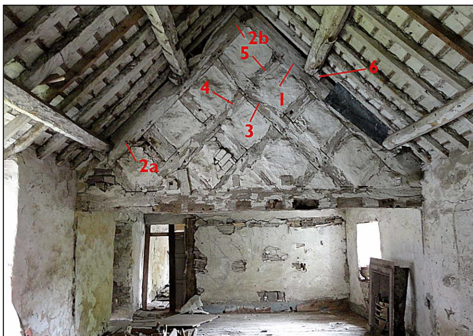
Figure 1: Photograph of the lattice truss (DM) showing the timbers sampled for dendrochronology, the samples were taken from the other face of this truss.
