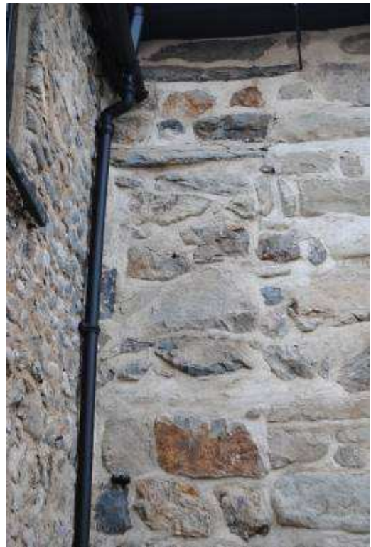
Plate 7: Blocked window at 1F level (infill abutted by west wall of porch).
