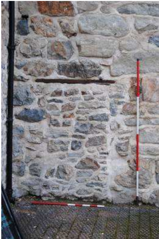
Plate 6: Blocked doorway to west of porch.
