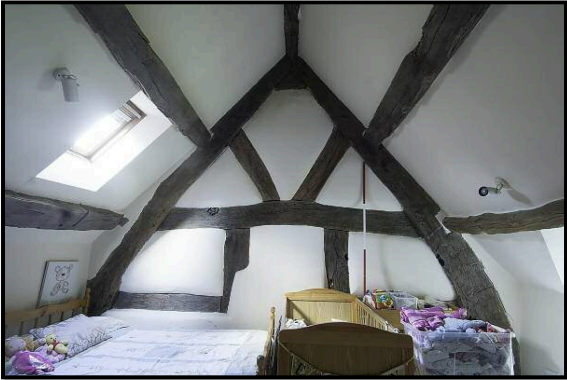
Figure 23: Fine timber framed gable Truss 3. Pegged from other, external, face. 3 Replaced purlins. Central panel not pegged on internal edge so possibly a window or even a door.
