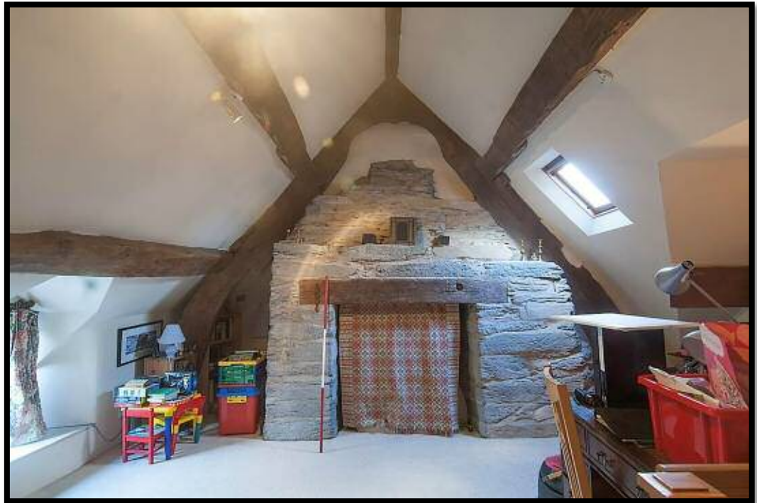
Figure 19: Truss 1. Remnant of truss sitting over the later inserted chimney stack. Encroachment of masonry enforced the removal of all the lateral timbers of the truss.
