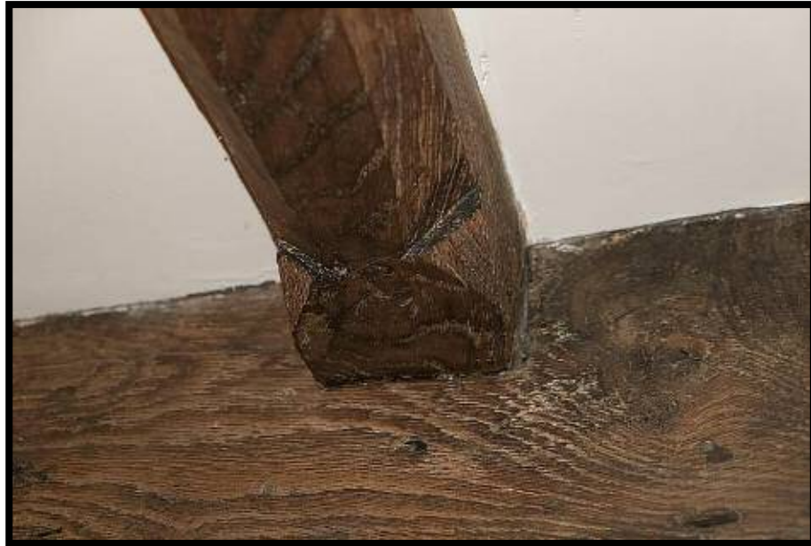
Figure 11: Joist from inserted floor showing deep chamfer and stopped and run out stop.
