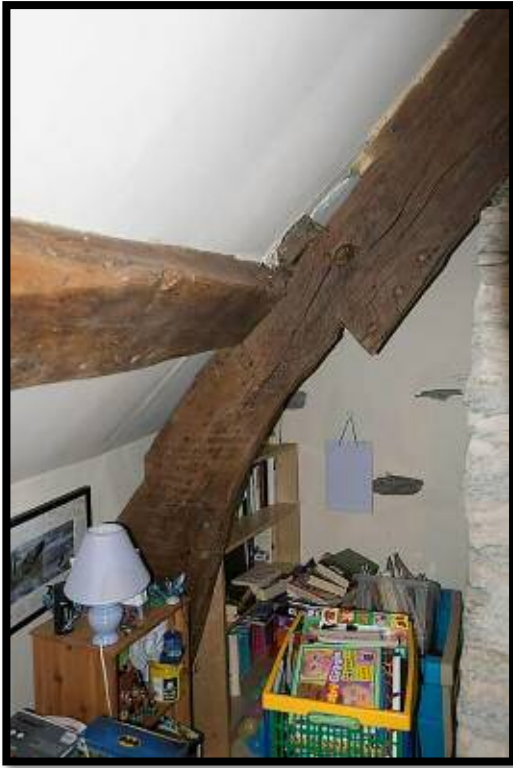
Figure 21: Left cruck blade T1. Three pegs for a collar. Evidence of several wind braces at this point, one heading beyond the purlin to a further bay now gone.
