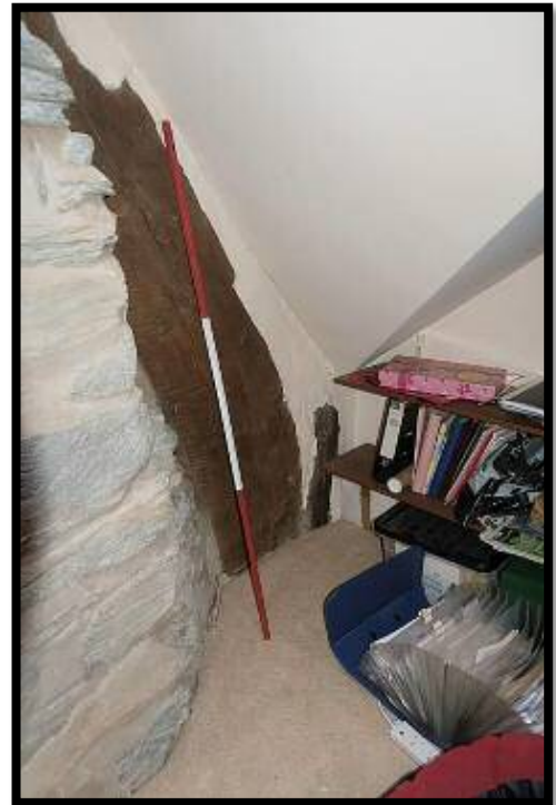
Figure 22: Right cruck blade Truss 1. Remnant of wall post signifying an alternative roof structure, probably timber framed.
