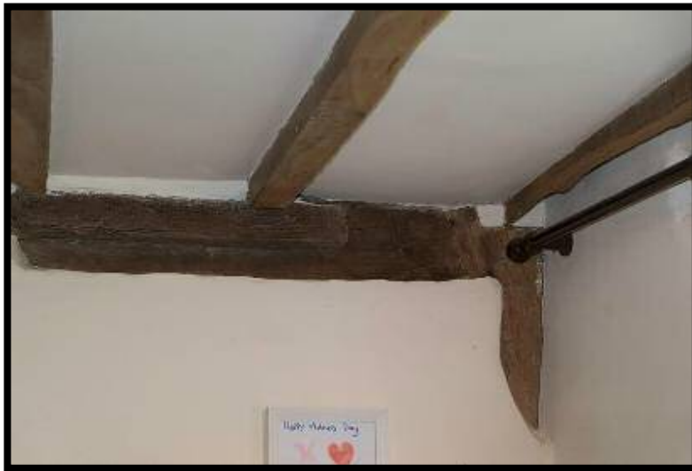
Figure 14: Gable of inner room. Cruck t right with jointed tie beam. Planted joist 'hanger' onto tie beam.
