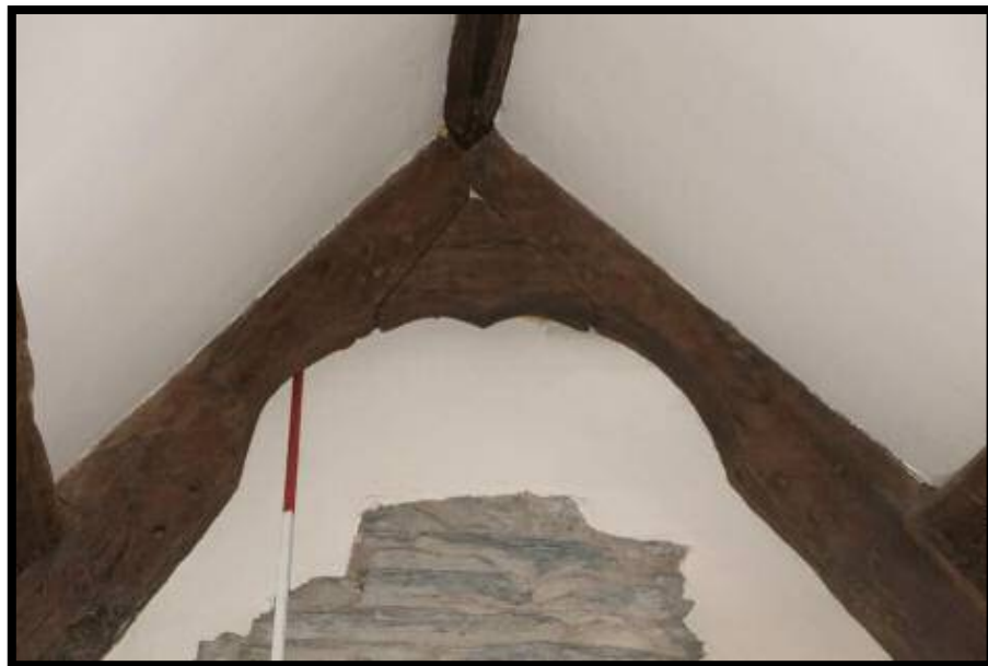
Figure 20: Detail of the apex of open truss. note triangular block at apex, a common feature in this area. In this case cusped to complement similar treatment on timbers.
