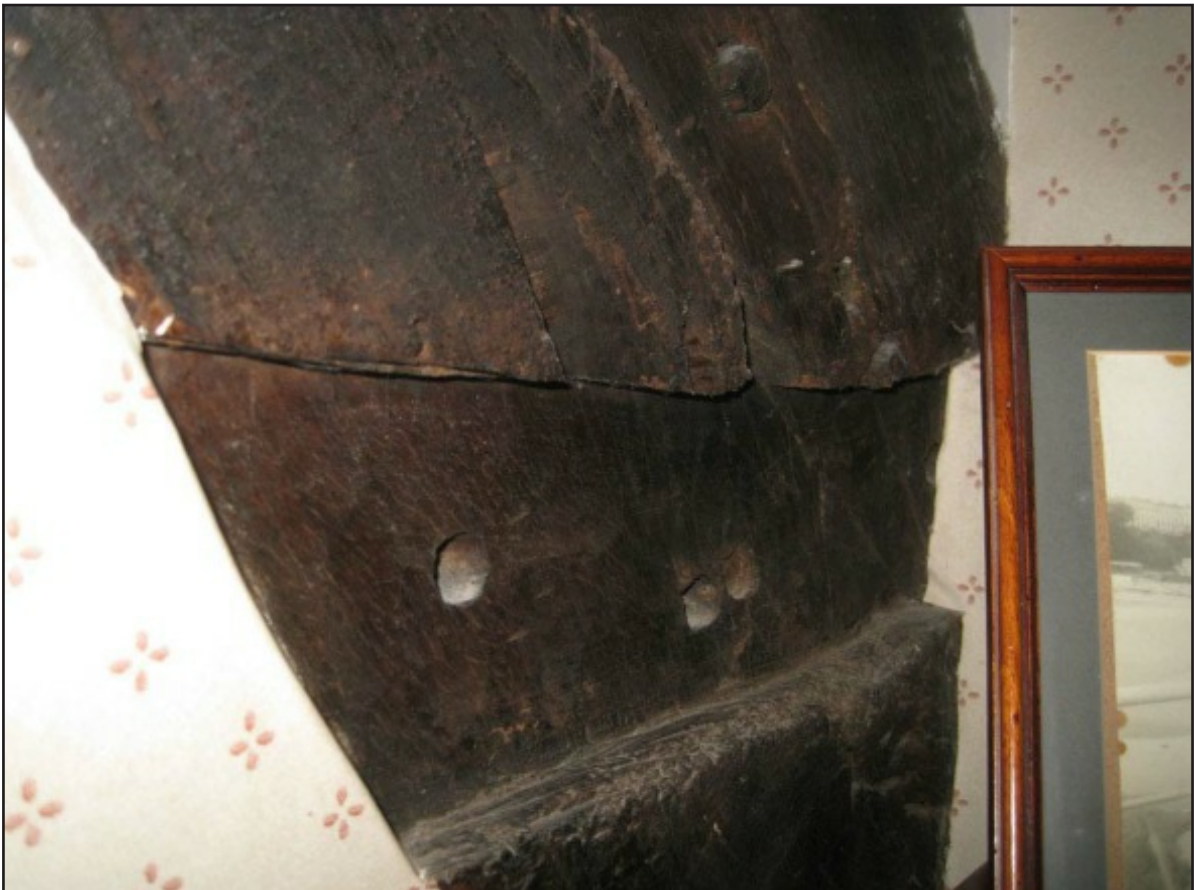
Plate 12: Close up of the housing for a tie beam on the eastern side of the southern face of the northern cruck, which forms the southside of the screens passage; view from the south.
