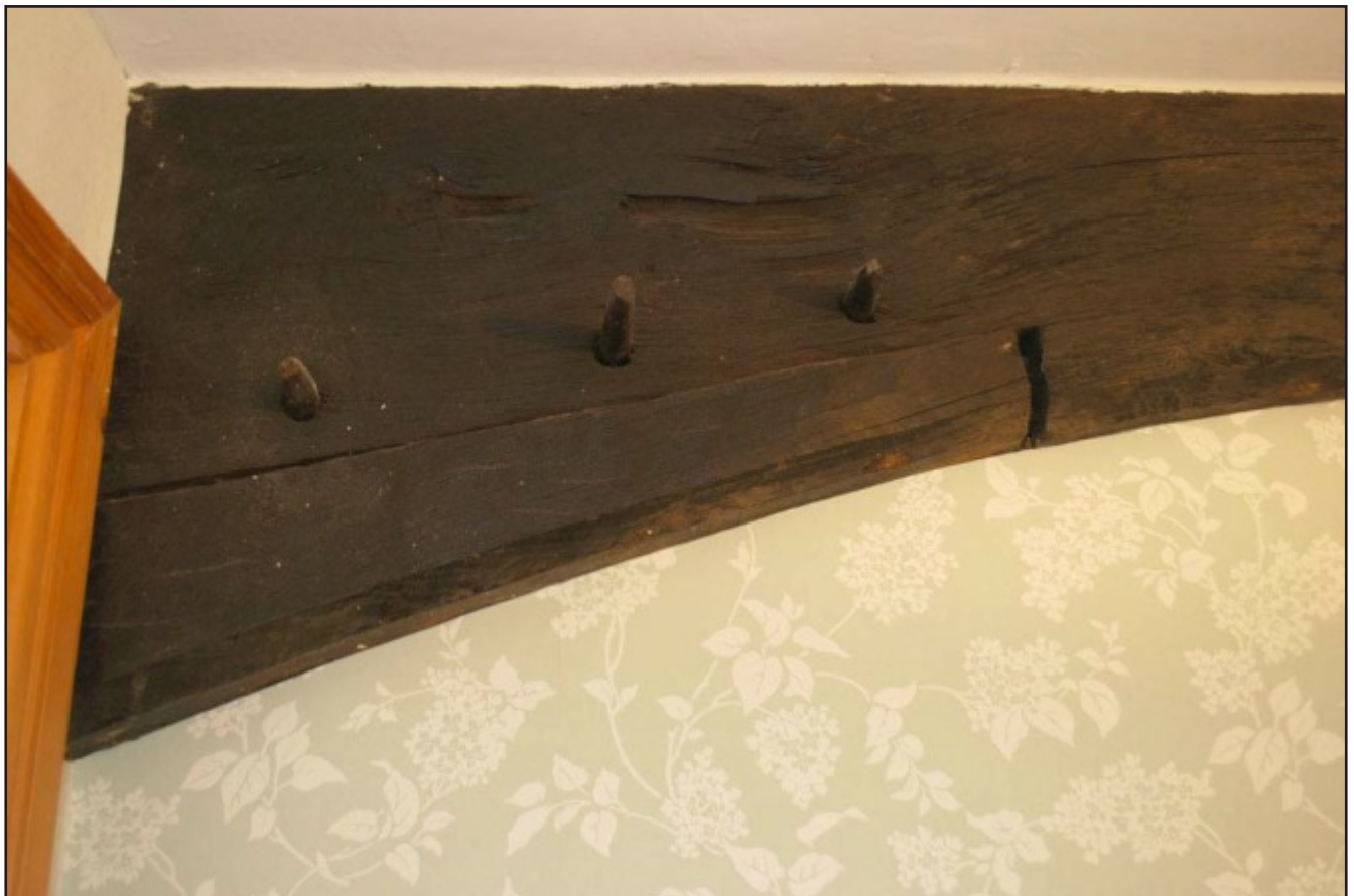
Plate 4: Close up of the pegs which join the jointed vertical post with the principal to form the bend of the southern cruck. This is the western side of the southern face; view from the south.
