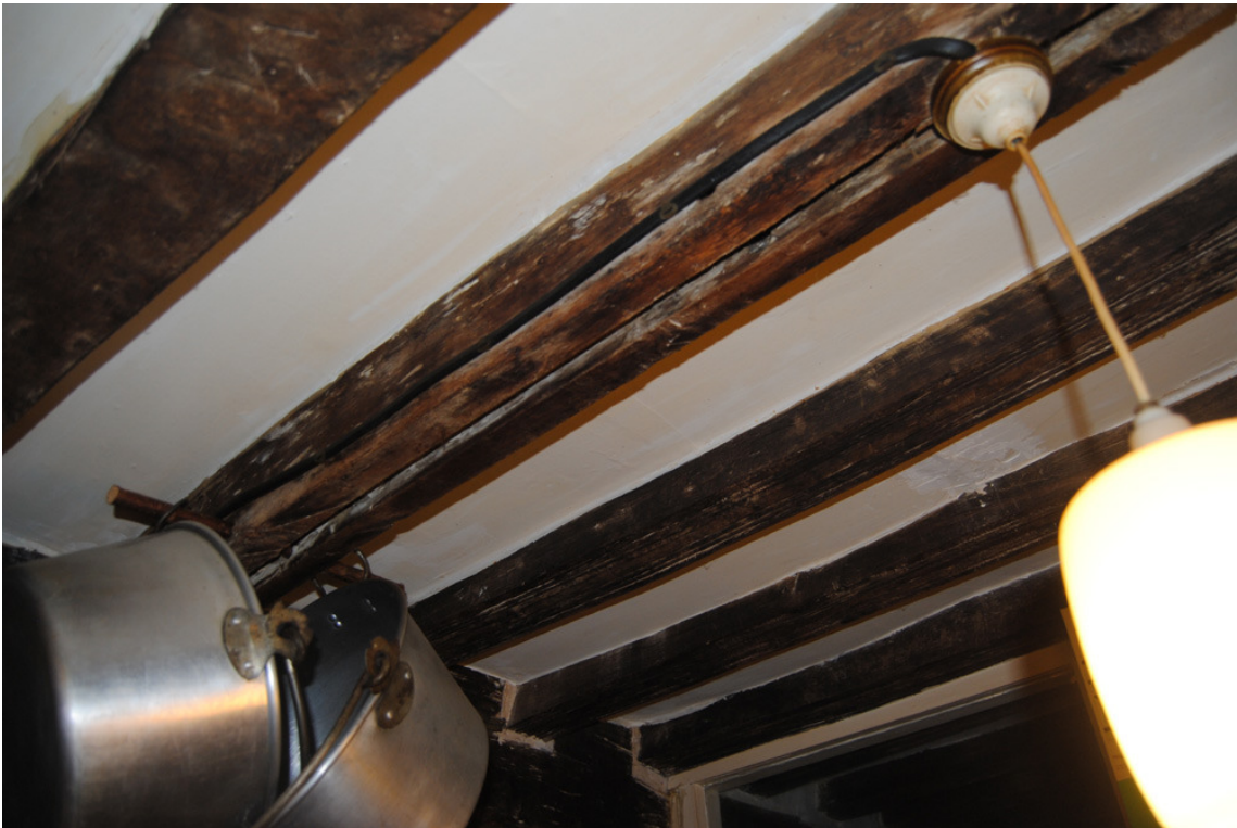
Plate 21: Ceiling structure of [GF03] with redundant mortices and groove indicating former lateral partition; NB: common joists to east are moulded, those to west are plain.
