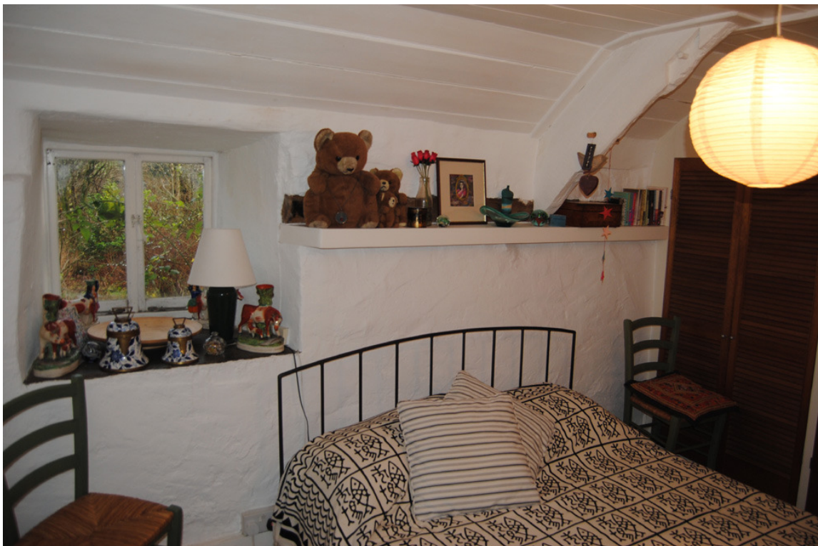
Plate 30: Room [1F03] looking east; note east principal of truss T2 with lap joints for former vertical studs.
