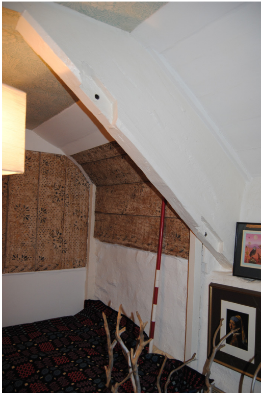
Plate 31: [1F04], west principal of T2 displaying lap joints for former vertical studs.
