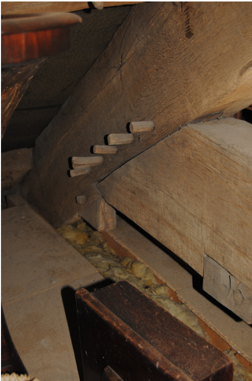
Plate 36: Truss T2; collar joint, NB. cut off studs.
