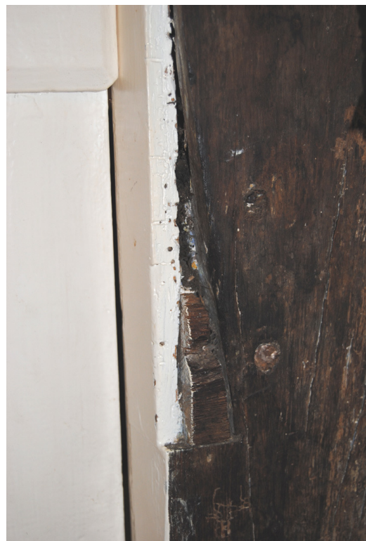
Plate 23: Notched joint evidences original door head location (see Figure 6).
