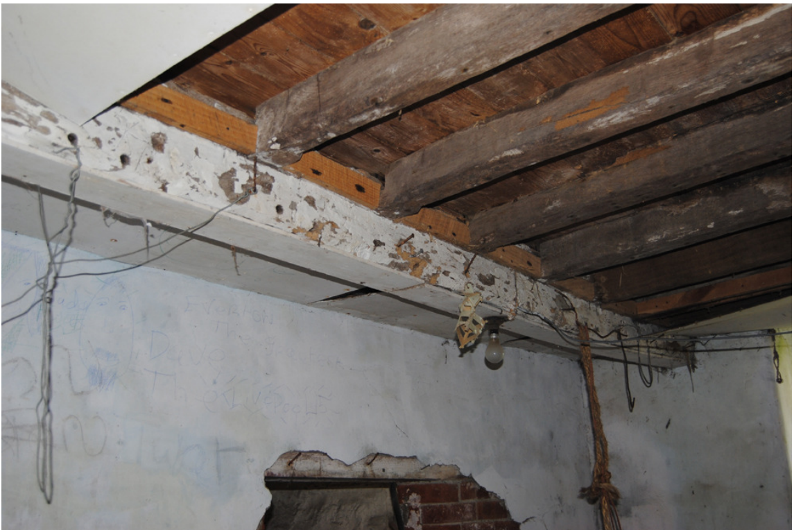
Plate 15: Primary ceiling beam within [GF02]; NB: regular paired peg-holes evidence primary partition.
