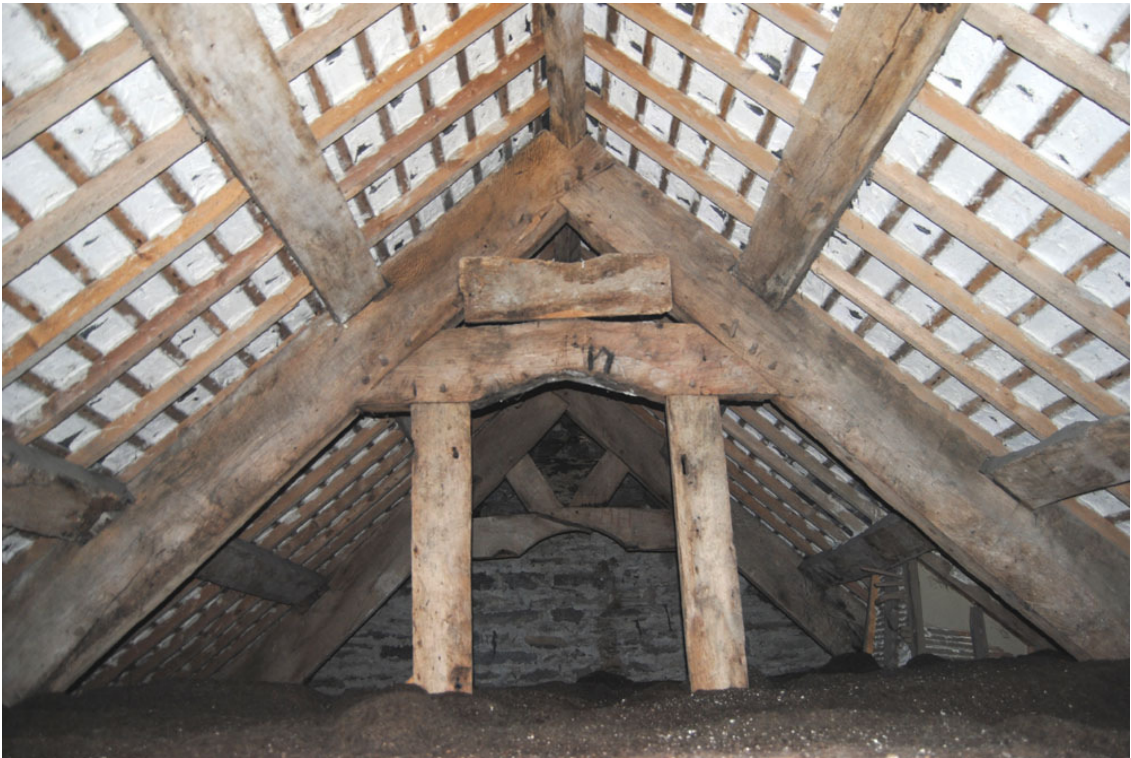
Plate 42: Roof over north-west range looking west, T2 in foreground, T1 with upper v-strutting beyond
