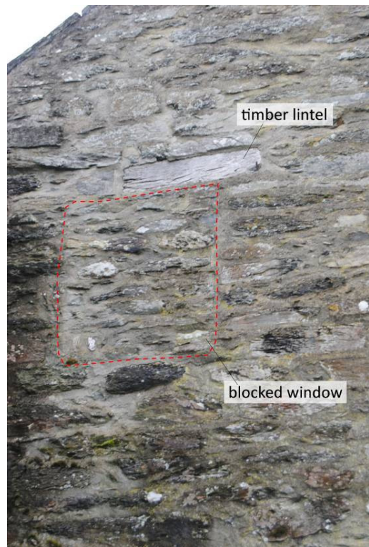
Plate 29: Blocked window at 1F (S).
