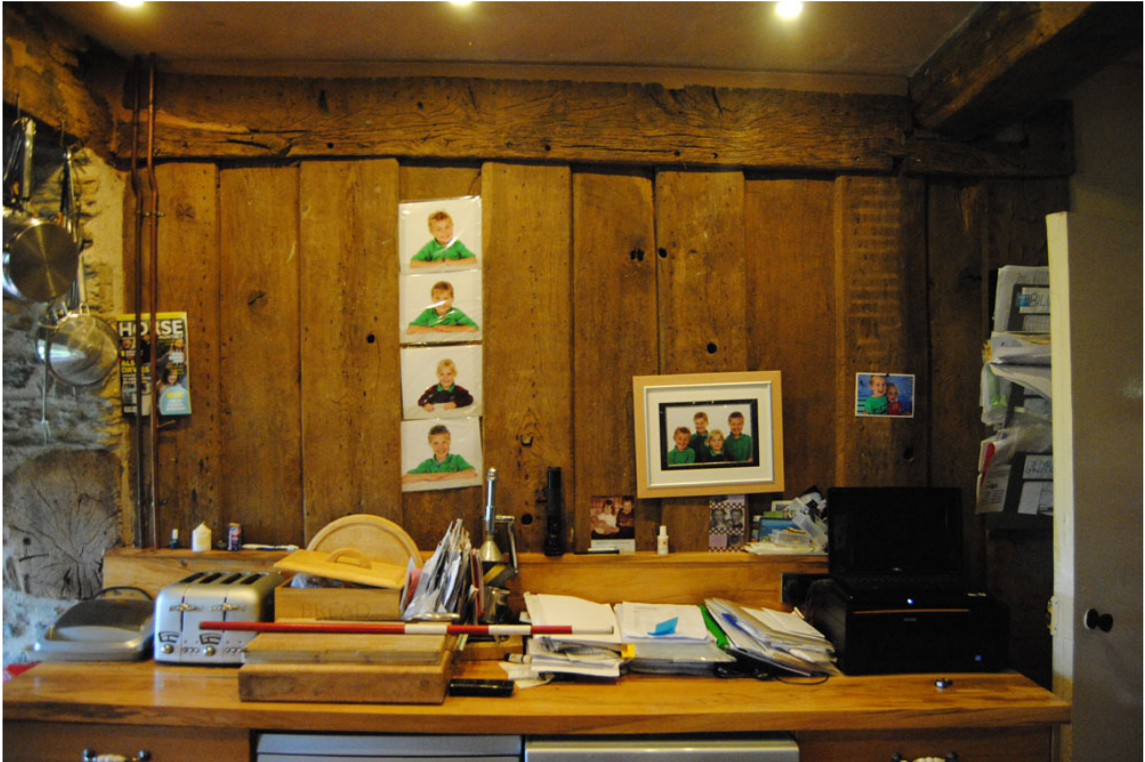
Plate 36: Plank and muntin partition forming south wall of [GF04], though situated within NW range.
