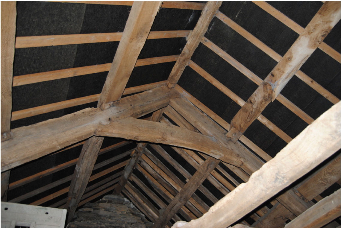
Plate 23: South-east range roof structure; central collar beam truss looking north (from 1F level).
