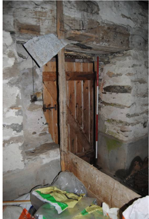
Plate 17: Doorway in west wall of [1F01] (NB: former window embrasure to left)
