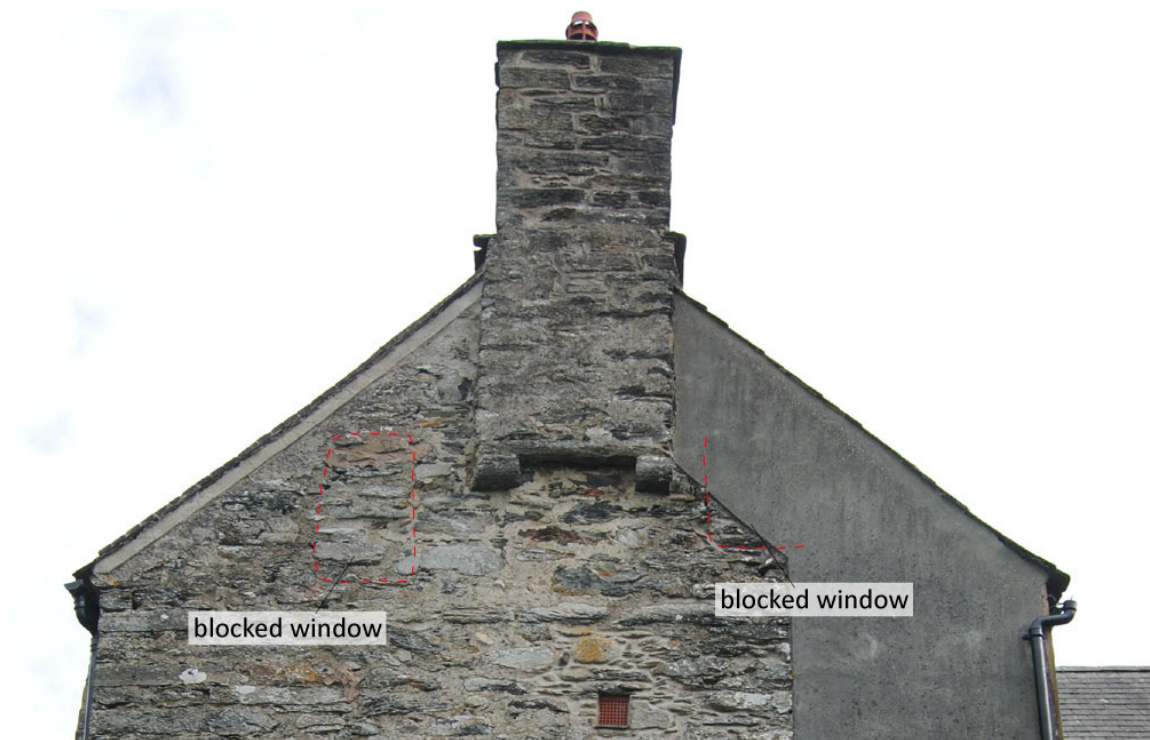
Plate 48: Blocked attic windows within north gable of kitchen extension.
