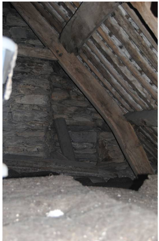
Plate 63: Truss T5, cruck-like east principal, note SJ of blocked window in gable wall beyond.
