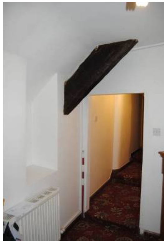
Plate 29: Landing [1F04] looking south, passageway to south range adjacent to stack; NB:E principal T2.
