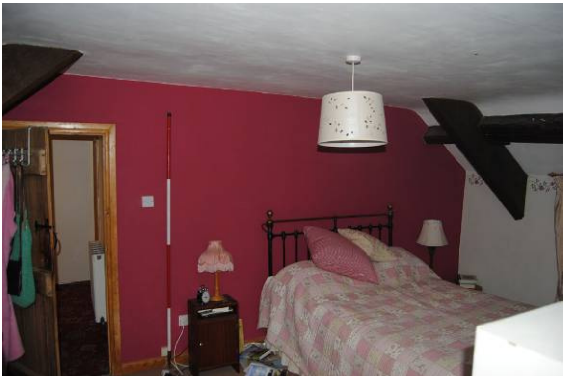
Plate 14: South range, Room [1F01] looking east with exposed principals and lower side purlins of T1.
