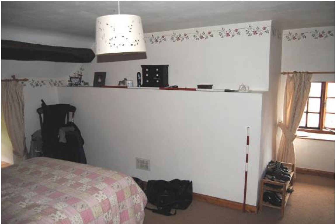
Plate 13: South range, Room [1F01]; stack at SW angle (fireplace blocked; note vent).
