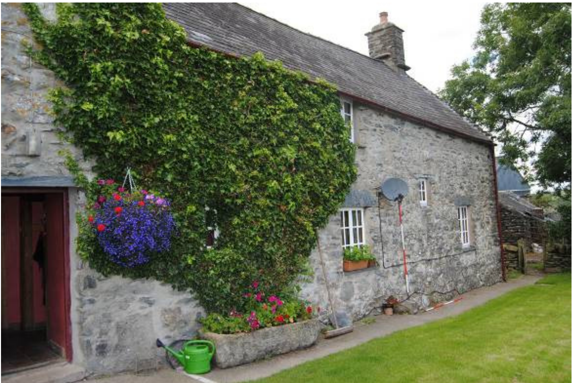
Plate 19: North range, east elevation oblique, looking north-west, note straight joint to right of door.
