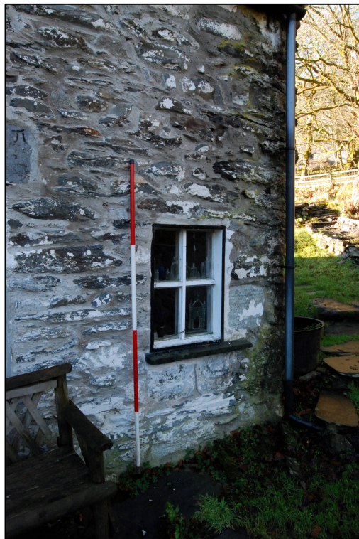
Plate 6: Partially blocked opening at the northern end of the eastern elevation
