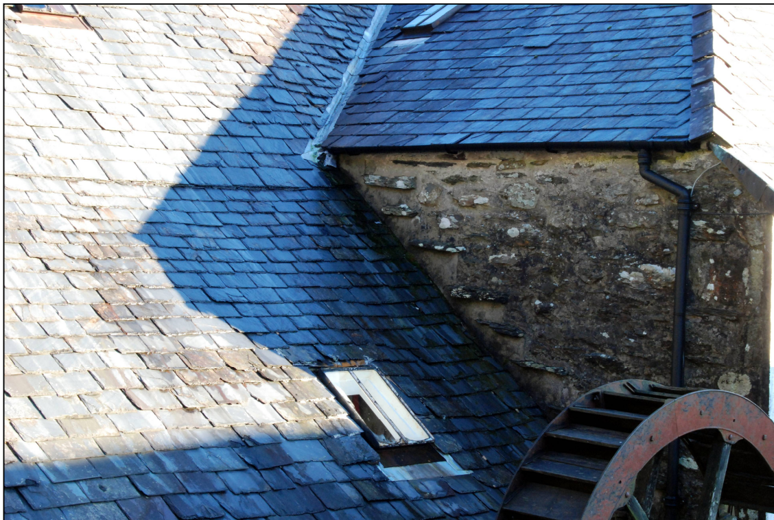
Plate 10: Water tabling above the "dairy range"
