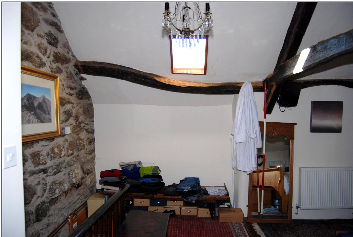
Plate 28: Warped purlin in the northern range
