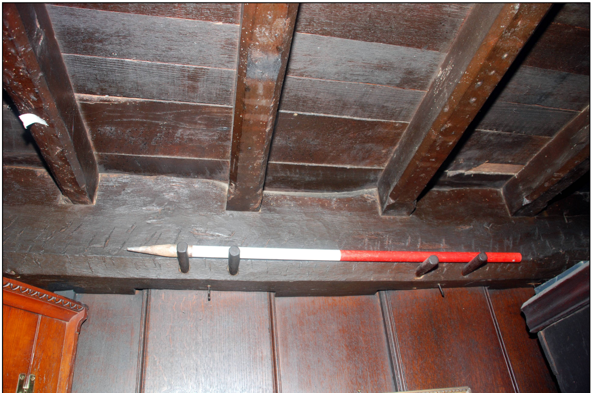
Plate 30: The joists in the southern, ground floor, room of the cross wing
