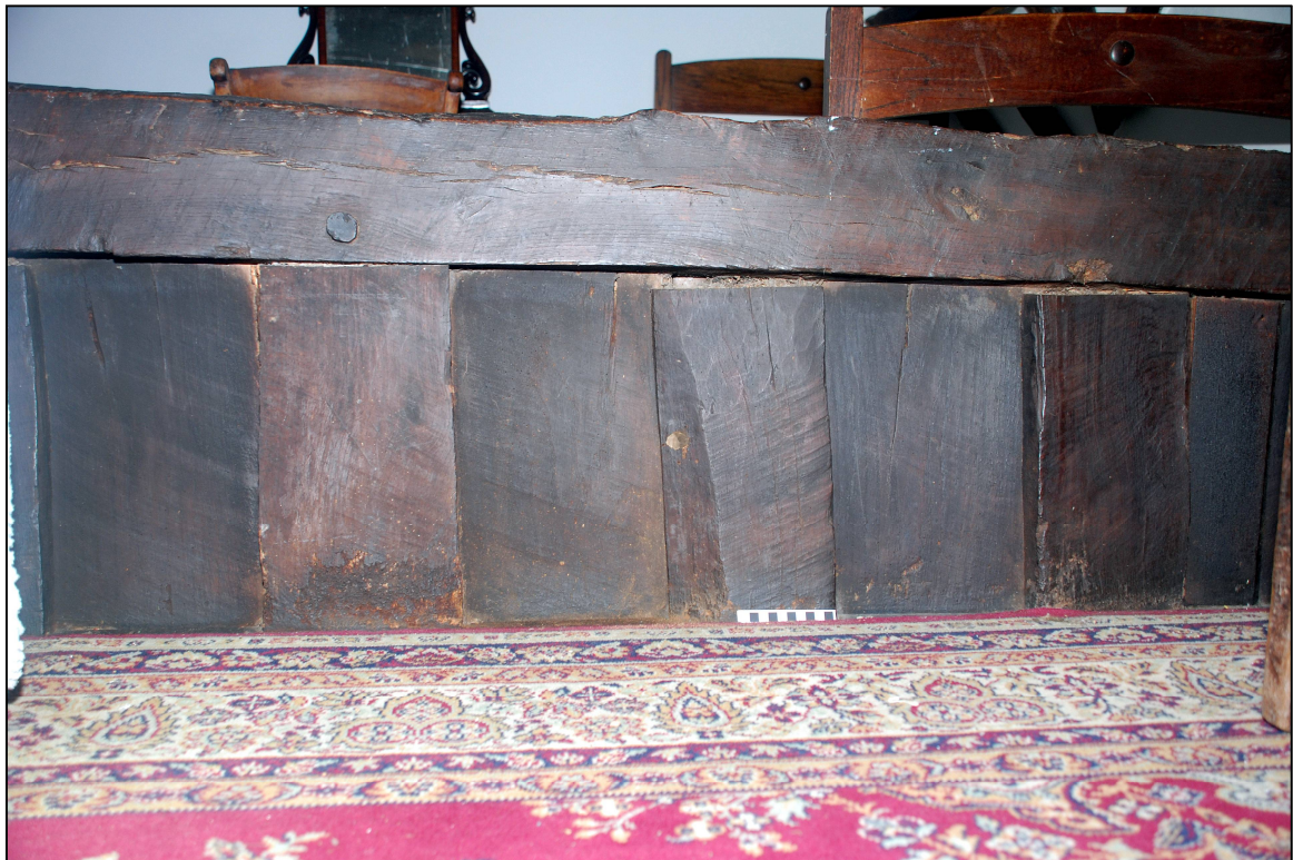
Plate 12: Detail of the partition between the pantry and the cross passage in the first floor room above
