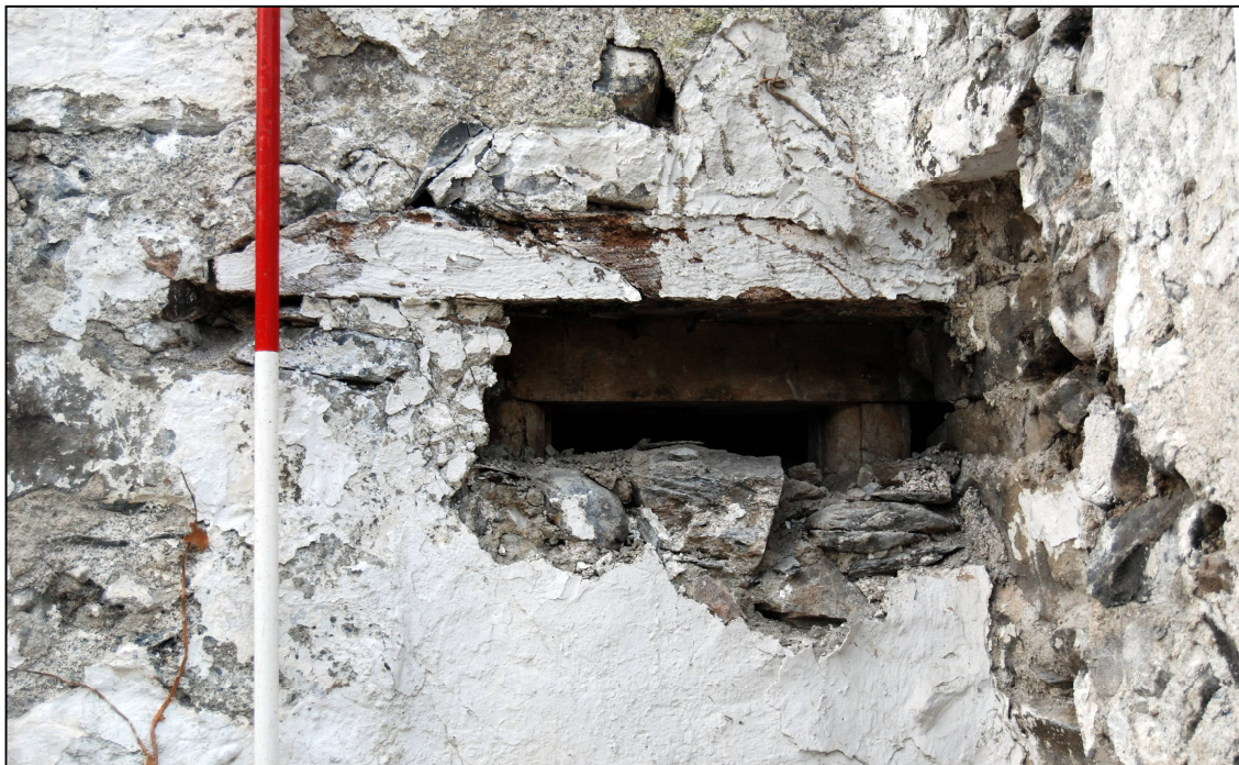
Plate 10: Detail of the window frame in the blocked window in the gable end of the southern range
