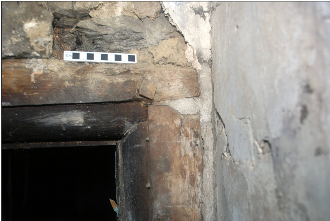
Plate 21: Detail of the ovolo moulding of the doorway between the kitchen and the hall
