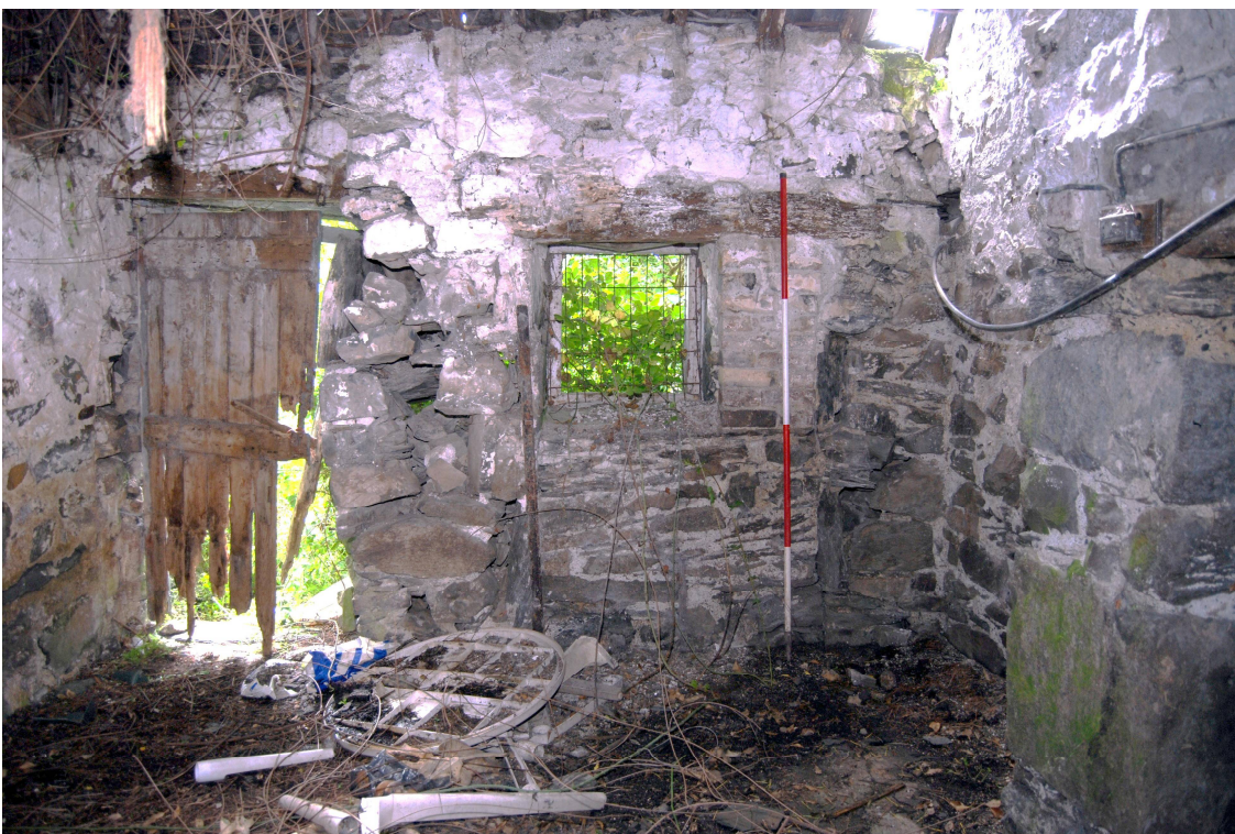
Plate 8: Window in blocked opening in the south eastern end of the building
