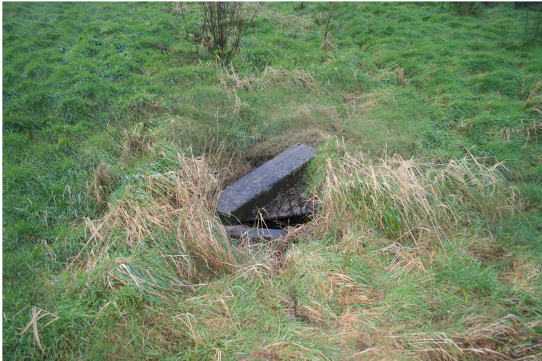
Plate 3: Damaged section of the culvert.
