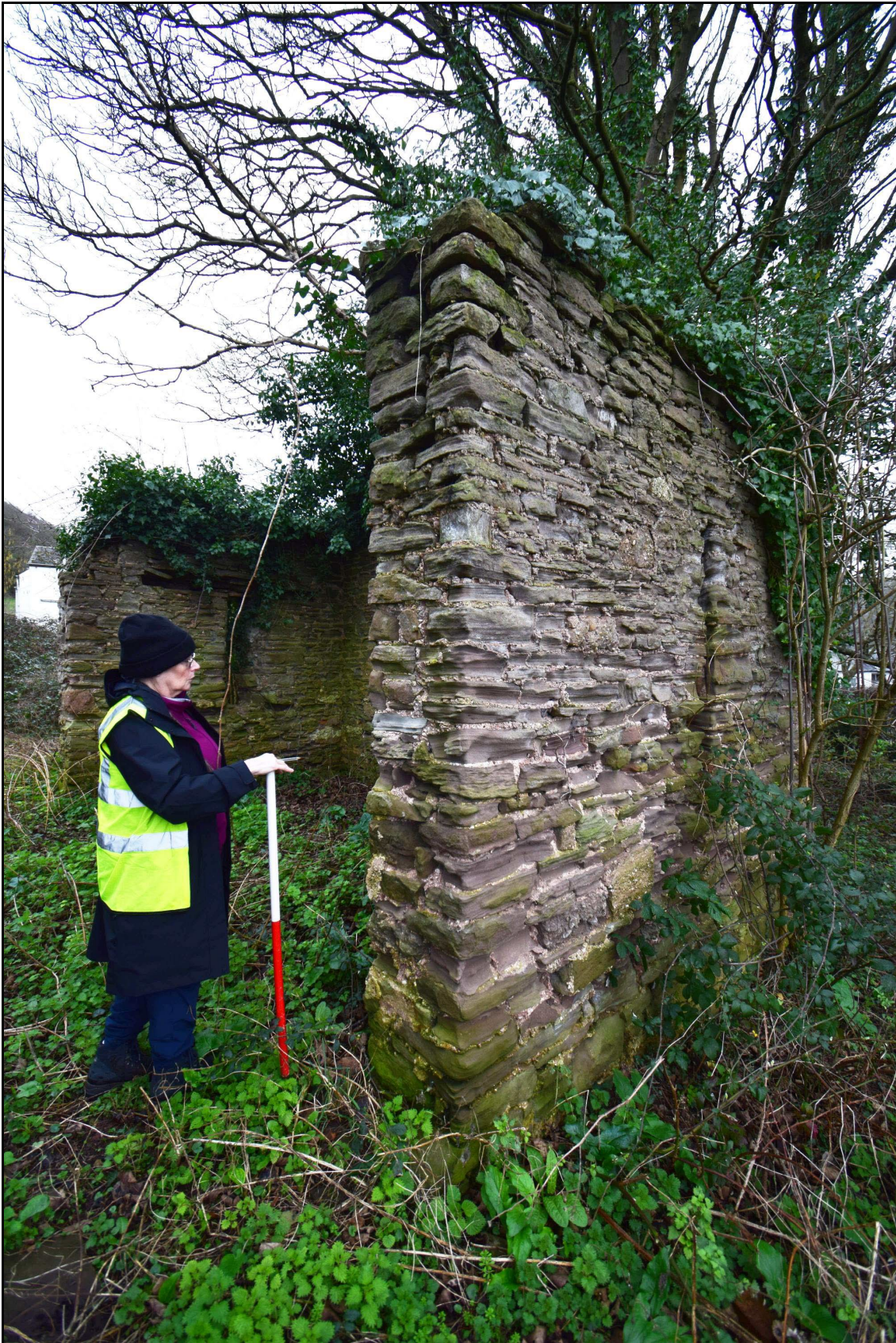
Plate 8 - TRW2024_008: A view of the lateral wall to the south of the west-facing doorway of the barn (ID number 22). Note the white lime mortar bonding the now heavily eroded sandstone masonry. Looking southeast.
