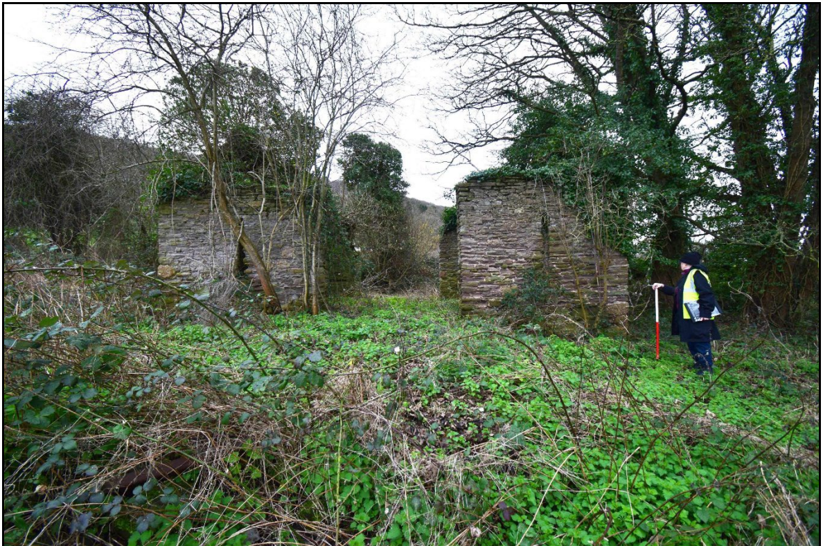
Plate 7 - TRW2024_007: A closer view of the now derelict barn (ID number 22) which once belonged to Tudor House. Note the wide, opposed doorways, suggesting it may have been used for threshing originally. There are narrow ventilation openings in the walls either side of the doorways. Looking east.
