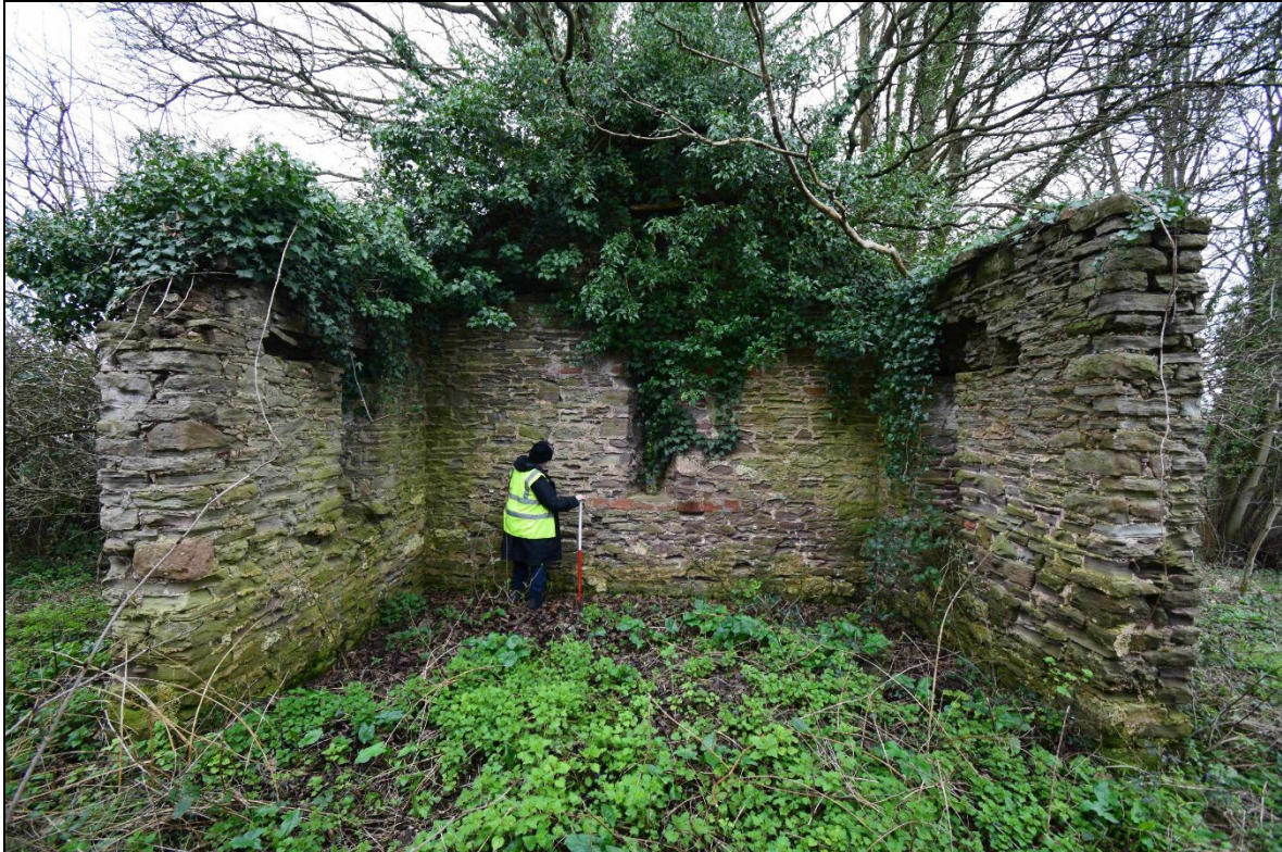
Plate 9 - TRW2024_009: A view inside the barn (ID number 22), showing a ventilation opening in the southwest gable end. The gable is fairly complete to ridge height and the lateral walls are largely intact to wallplate level. Looking south.
