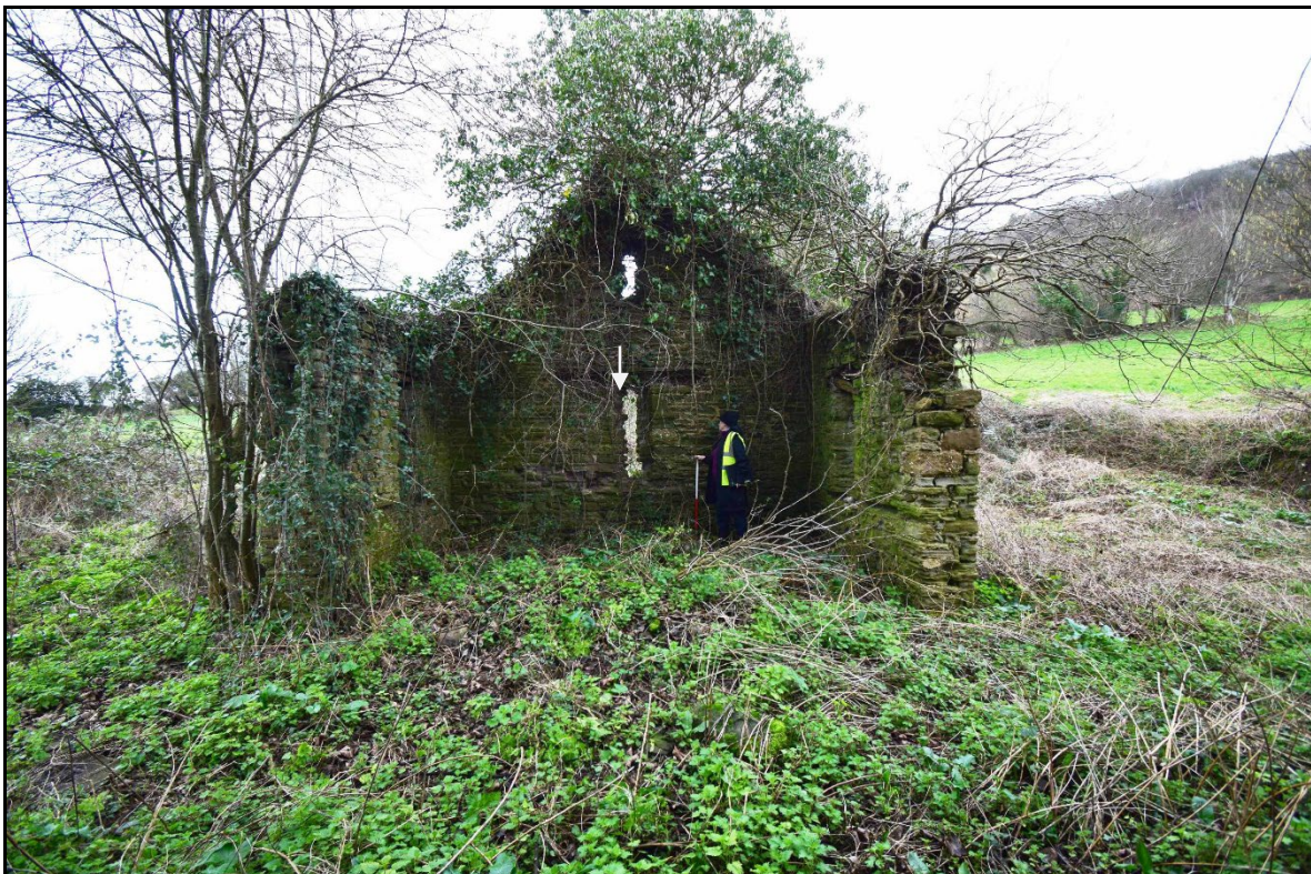
Plate 10 - TRW2024_010: A view inside the barn, showing the ventilation openings in the northeast gable end. This gable is also fairly complete to ridge height and the lateral walls are largely intact to wallplate level. Looking north.
