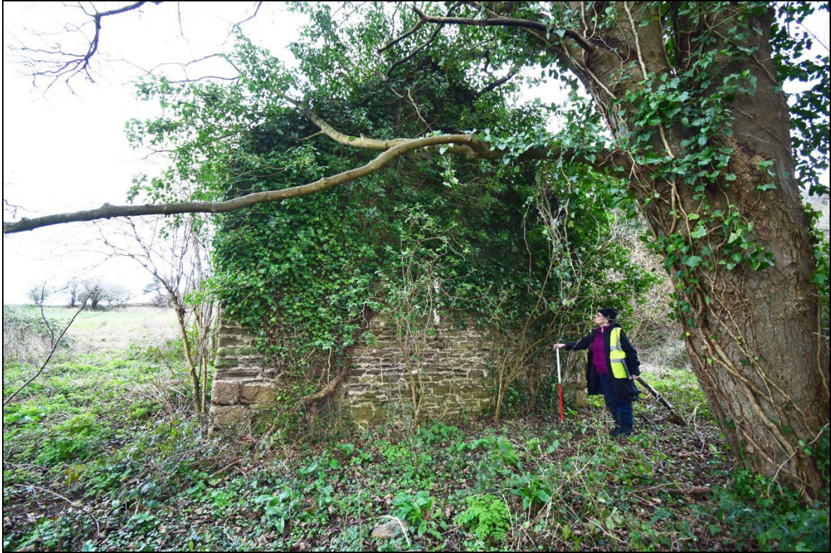
Plate 13 - TRW2024_013: A view of the southern gable wall of the now derelict barn (ID number 22). Looking north.
