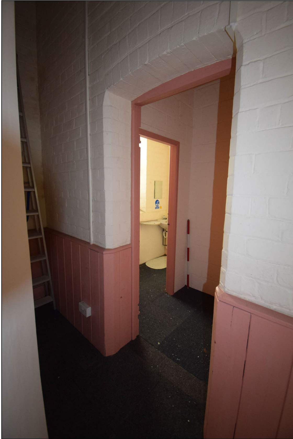
Plate 14: PSC2023_014, A view from the main hall of the schoolroom into the southeast extension where the toilet block is located. Looking south.
