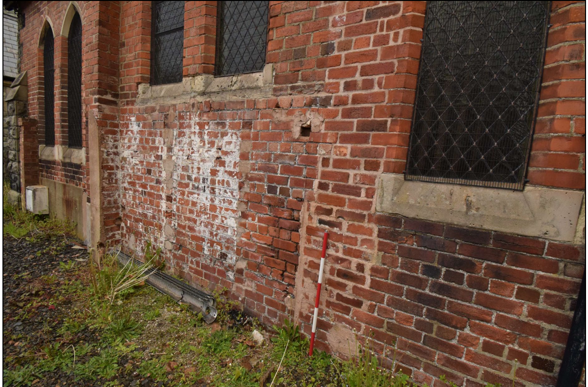
Plate 6: PSC2023_006, An external view of the southwest wall showing the brickwork of the schoolroom and a scar where a small structure once stood against the wall, and some repairs to the brickwork. Looking north-northwest.
