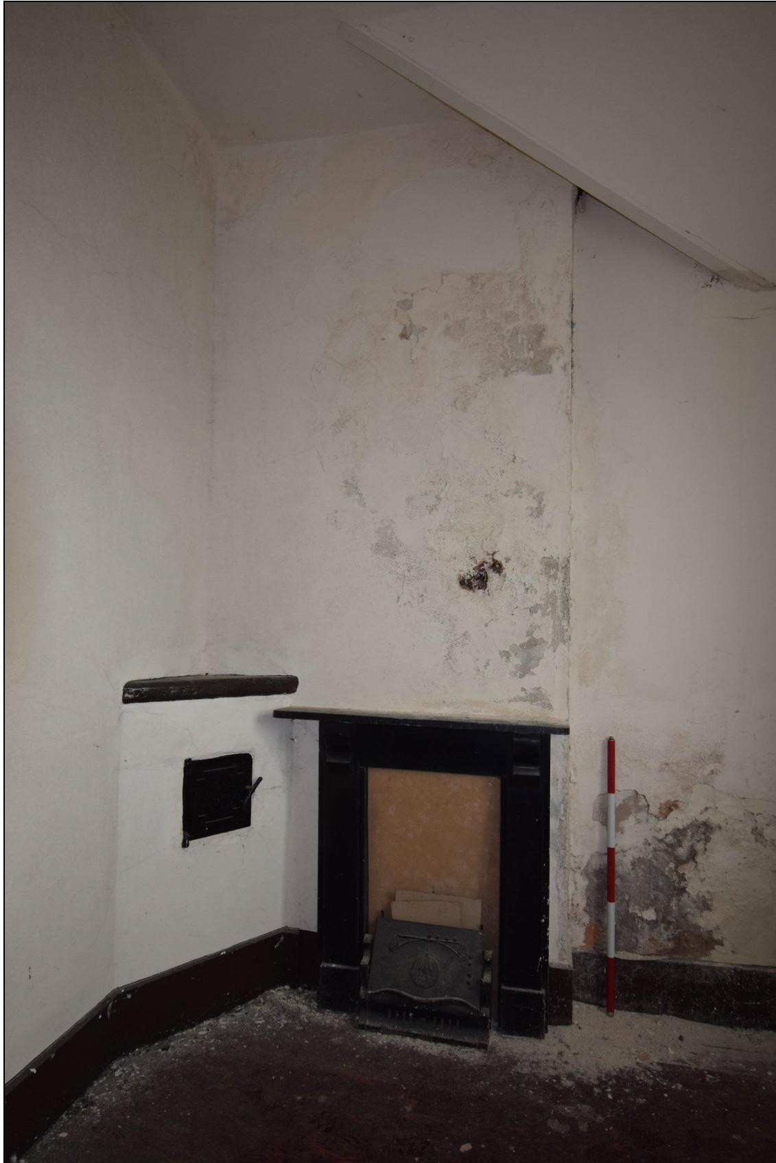
Plate 38: PSC2023_038, A view inside the vestry at the south corner of the chapel, showing the fireplace. Looking west-northwest.
