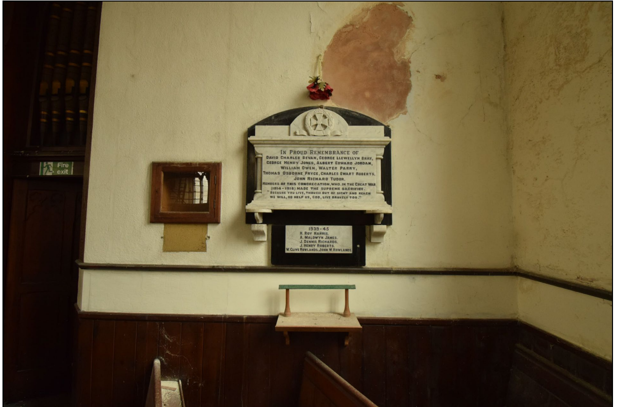
Plate 35: PSC2023_035, A view of a memorial plaque to the southwest of the pipe organ. Looking southeast.
