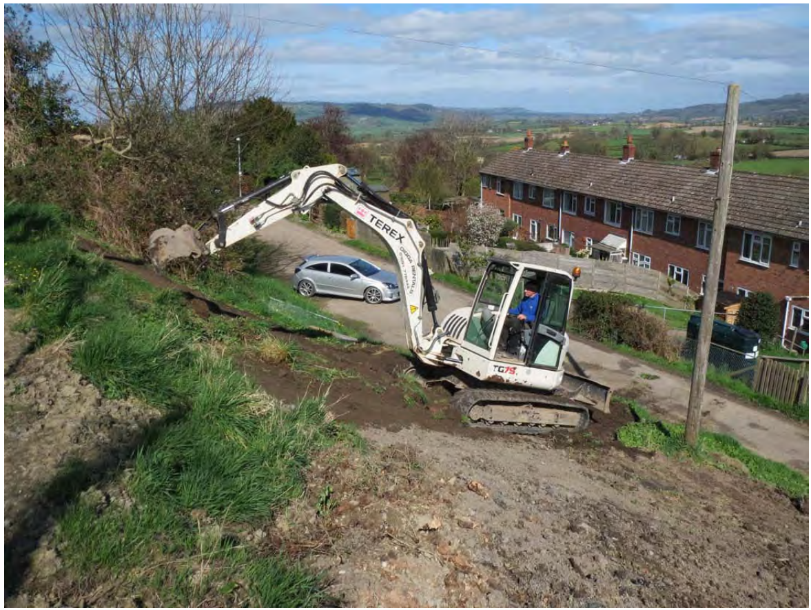
Plate 27. Working shot of the soil strip to the north of the former garages. Looking North-North-East.
