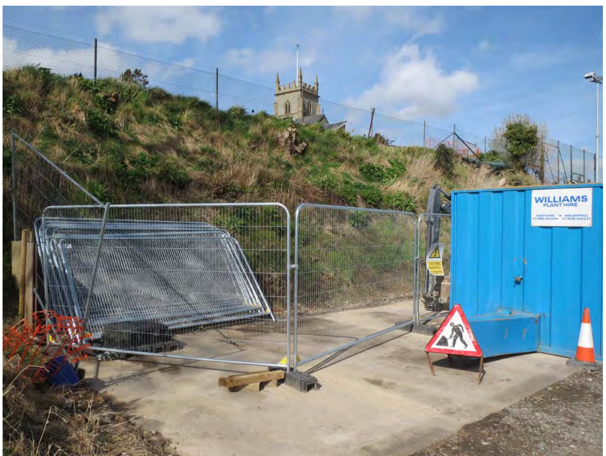
Plate 2: View of cutting into medieval bank for garages (demolished). Looking north north west
