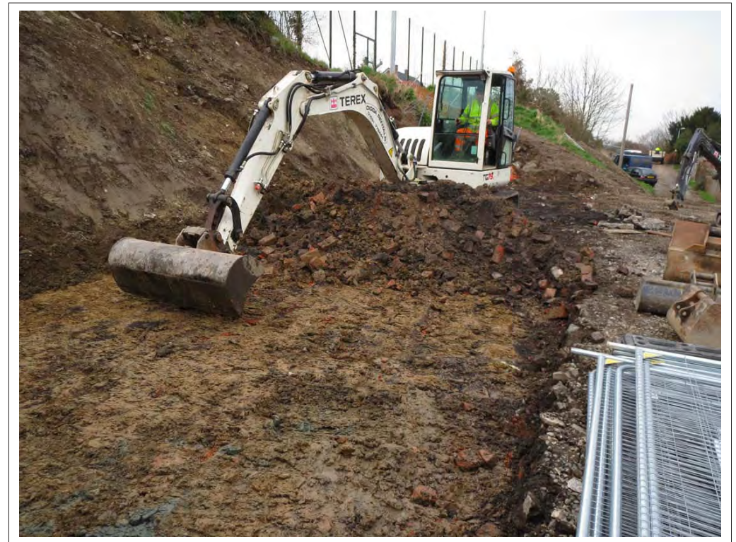
Plate 20. Working shot of soil strip within area of former garages. Looking North-North-West.
