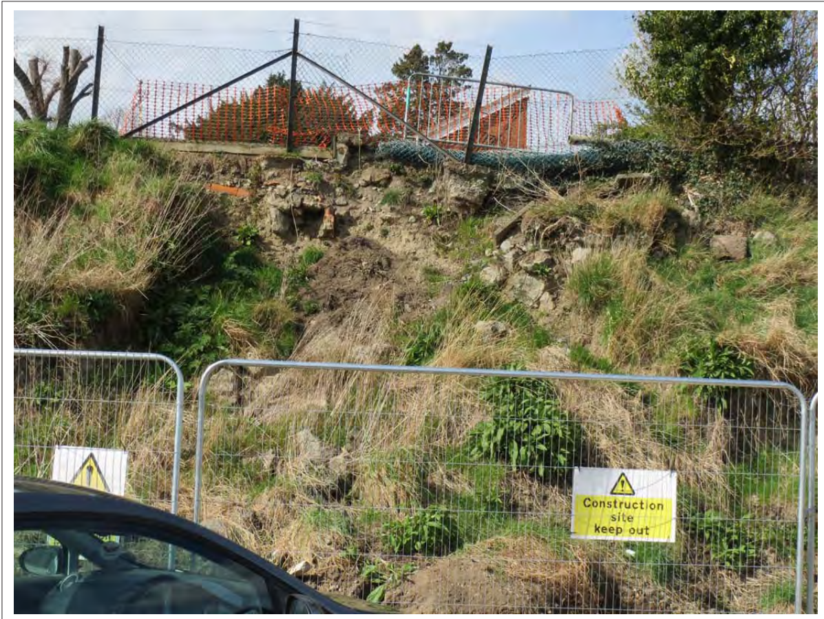
Plate 3: Area of landslip/slumping at the top of the bank, below the eastern edge of the bowling green. Looking west
