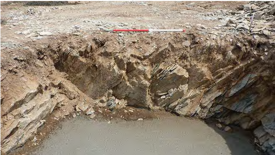
Photo 14: South facing shot of one of the foundation pads for the crane showing the thin deposit of topsoil (102) overlying the bedrock (104). 1m scale.
