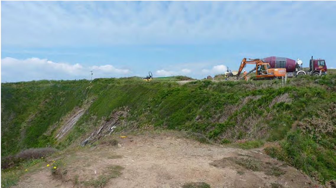
Photo 2: View northeast from beyond the site boundary, looking back at the site during foundation works for the crane pad.
