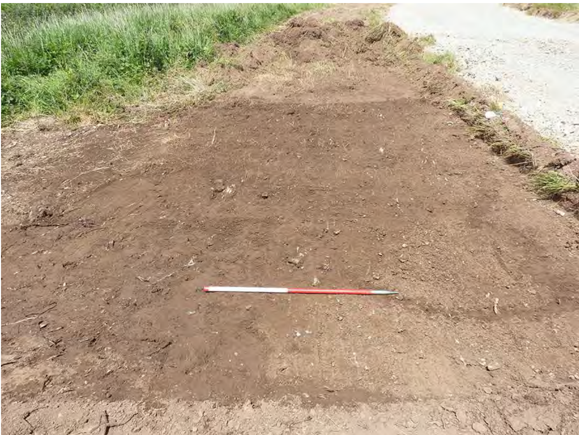
Photo 4: Looking north at area stripped alongside the main access track for the temporary site welfare units, showing topsoil deposit 100. 1m scale.
