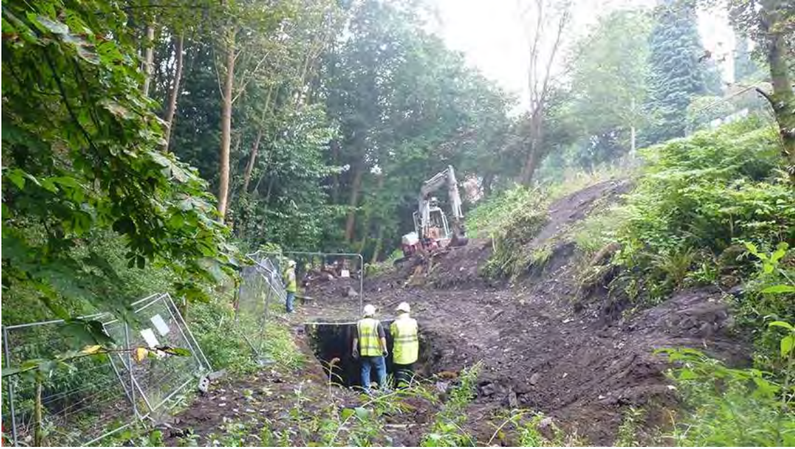
Photo 1: View south down the small valley along which the culvert runs. Showing the area of collapse and the extent of the scoured area at the valley bottom.
