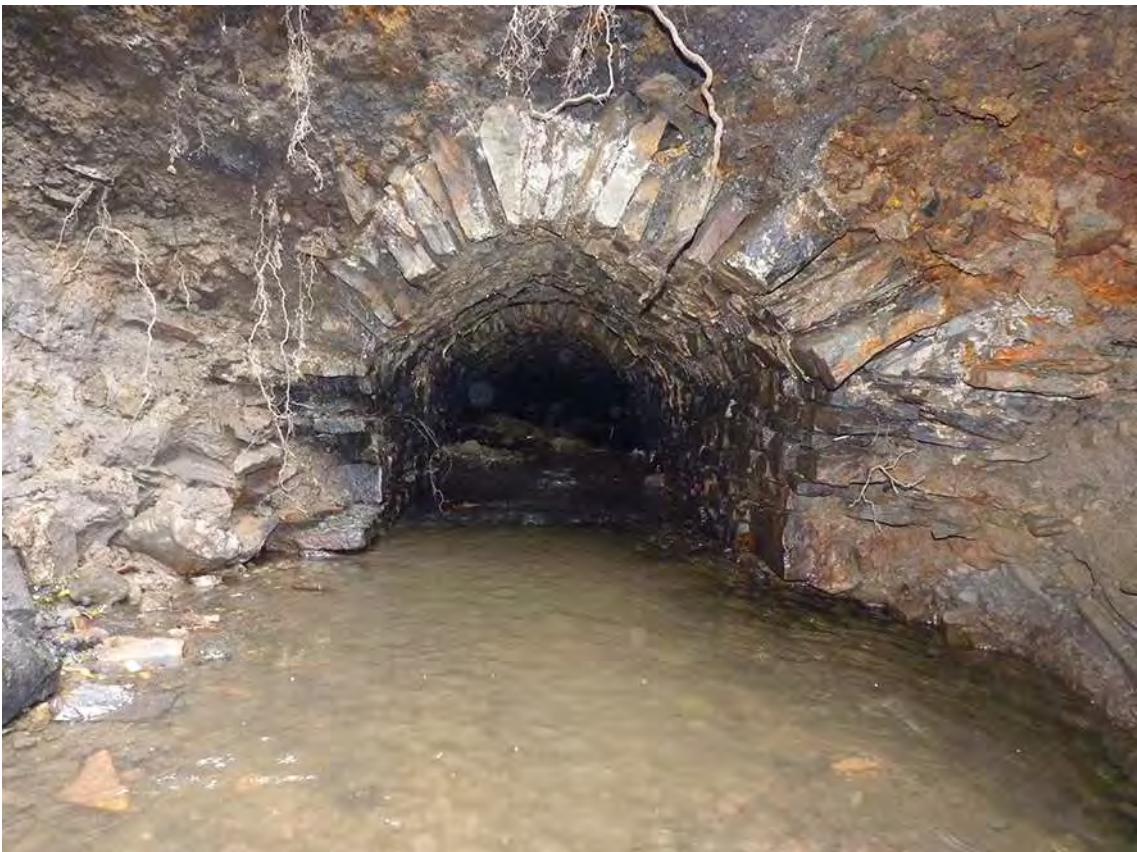
Photo 16: South facing view down the surviving section of culvert. The opening for the manhole is visible in the roof of the culvert a short distance in.
