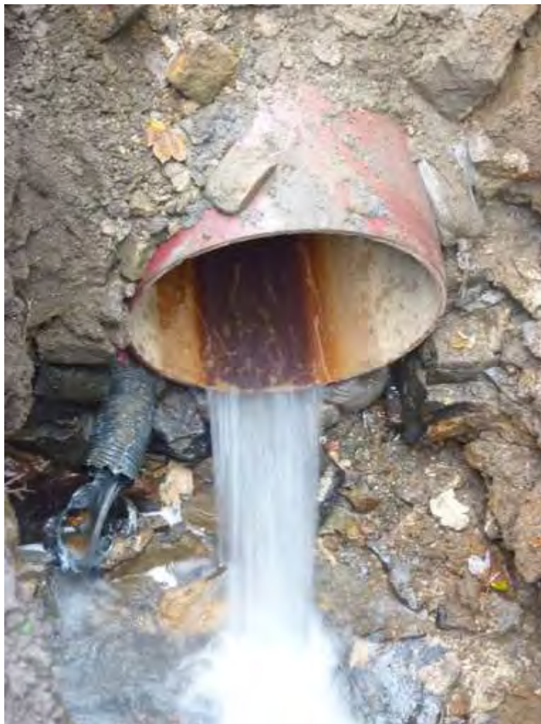
Photo 10: Close-up of the inserted pipe. The remains of the stone culvert is visible on either side of the pipe.
