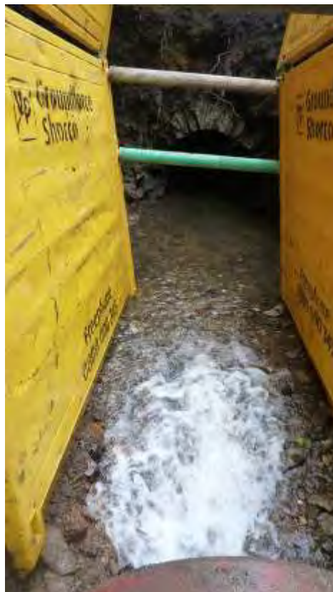
Photo 12: Facing south, showing the surviving section of culvert and the extent of the shoring within the collapsed area, demonstrating the difficulties of getting a detailed recording of the surviving culvert.
