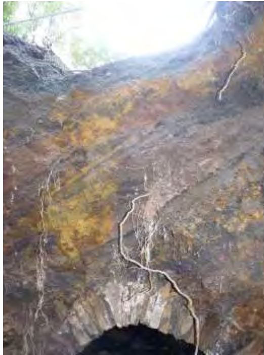
Photo 21: Backfill deposit visible in section above the culvert. Shows tip lines coming in from the west, and iron staining suggesting these deposit derive largely from waste material from the iron working processes.
