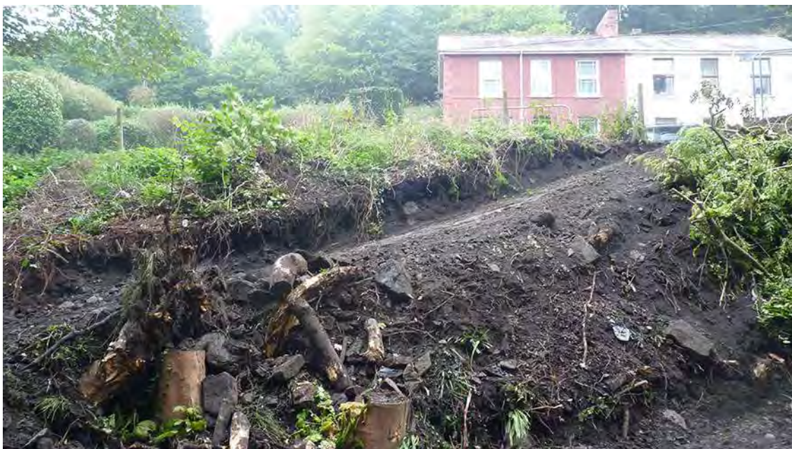
Photo 4: West facing shot of the ramp created to gain access to the valley bottom.
