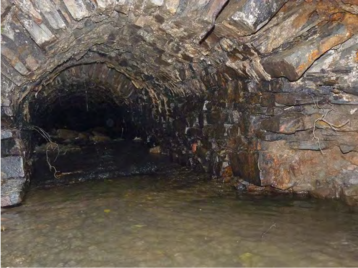
Photo 17: Oblique shot showing more detail for the western wall and arched roof of the culvert. Again the manhole opening is visible in the roof of the culvert.
