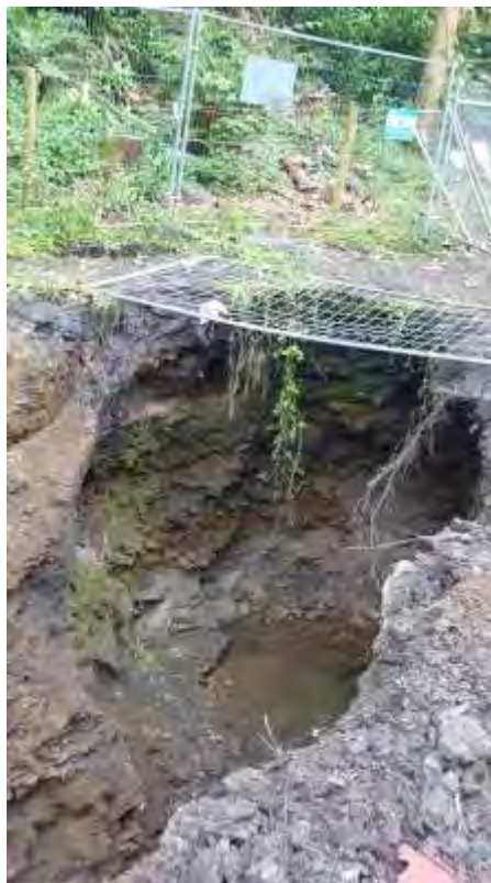
Photo 8: View of the collapsed area, facing southeast.
