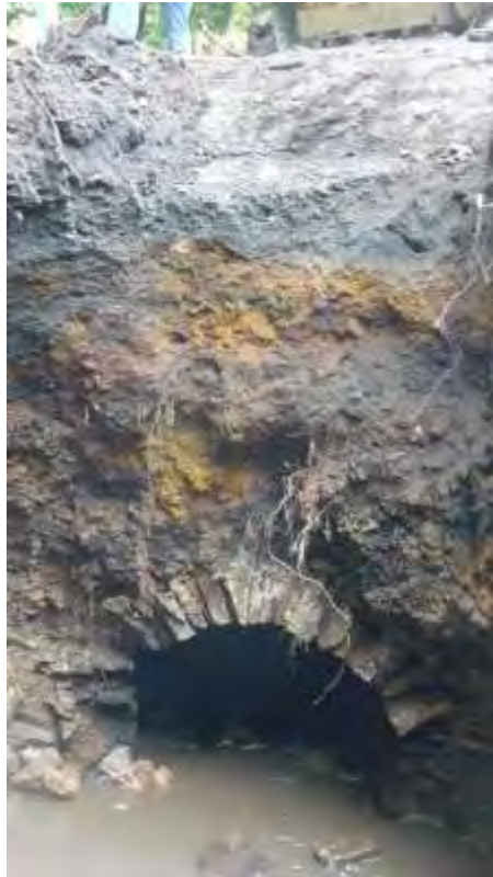
Photo 11: South facing shot of the surviving section of culvert showing the depth of material above it.
