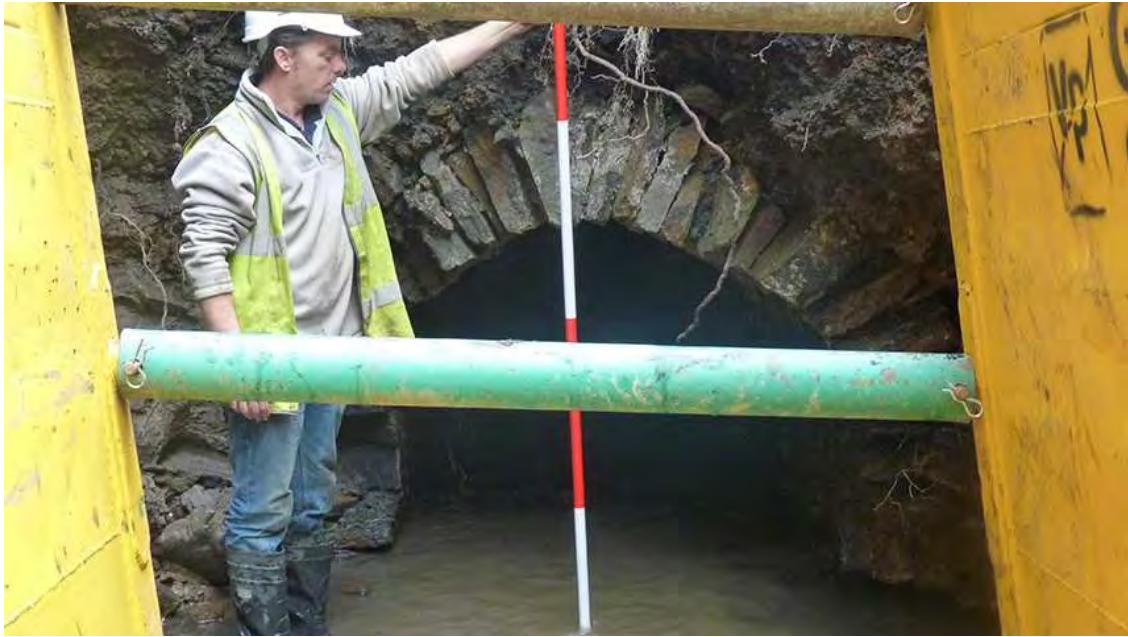
Photo 13: Facing south, surviving section of culvert with 2m scale. Taking scale photos was not feasible due to overhanging deposits.
