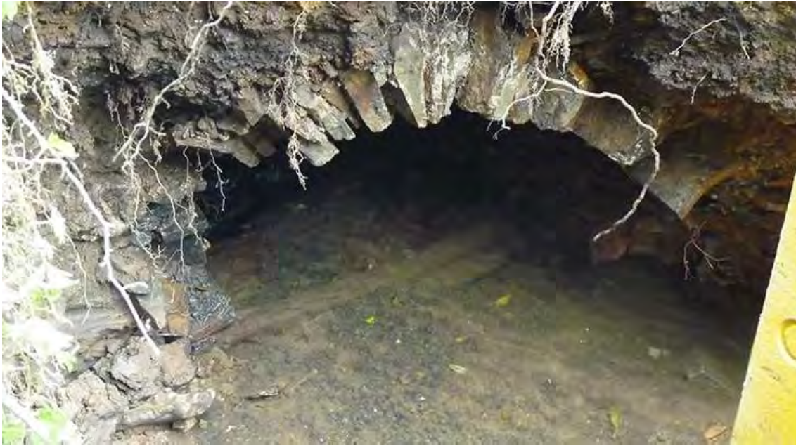
Photo 19: Southwest facing shot showing the wooden beams along the base of the culvert
