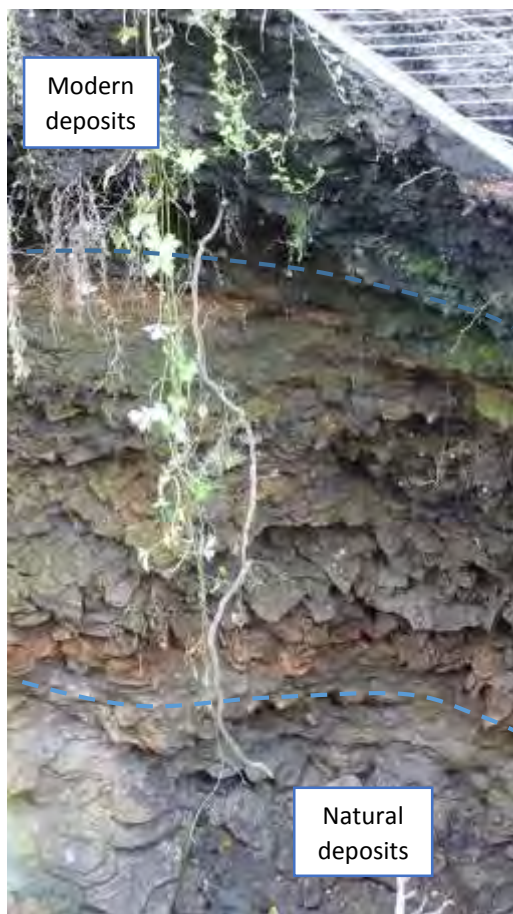
Photo 24: East facing, and slightly downward view of the deposits revealed in the side of the collapsed area. Showing natural stone and clays at the base, overlaid by large amounts of presumed 19 th century material that appeared to cover the line of the culvert. The dark deposit of modern disturbance and overburden is visible at the top.
