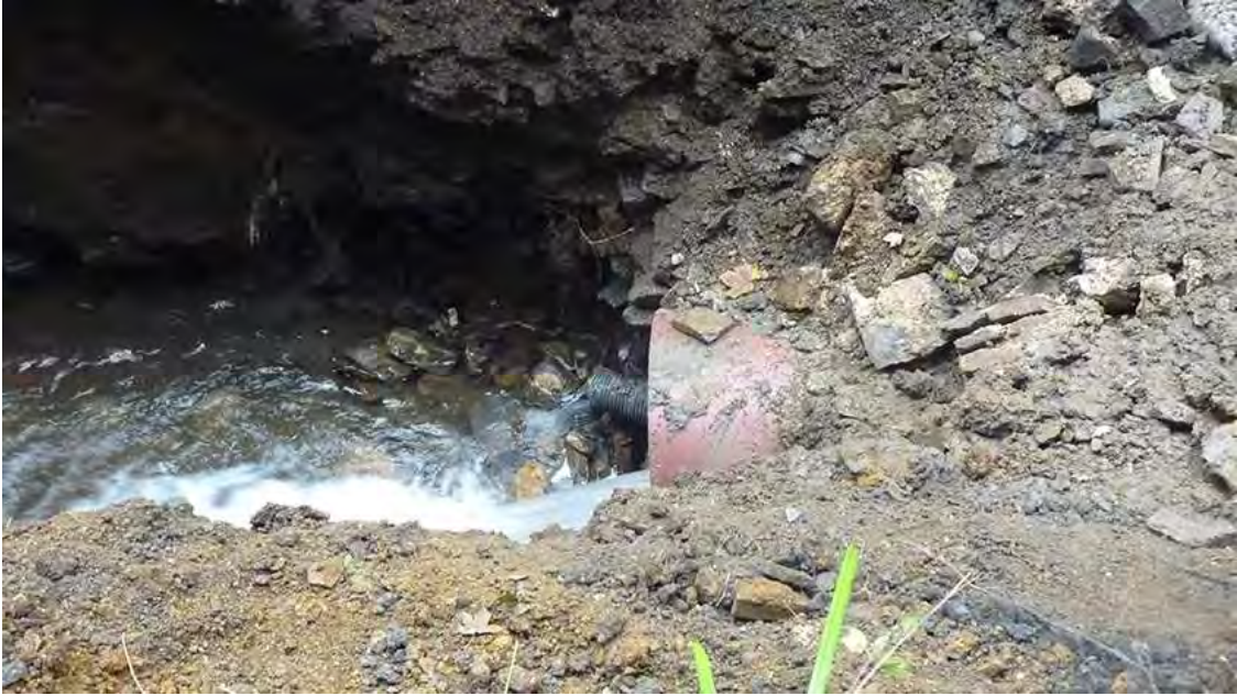
Photo 9: West facing shot of the northern end of the collapsed area, showing the pipe inserted through the culvert in the previous stage of repair work.
