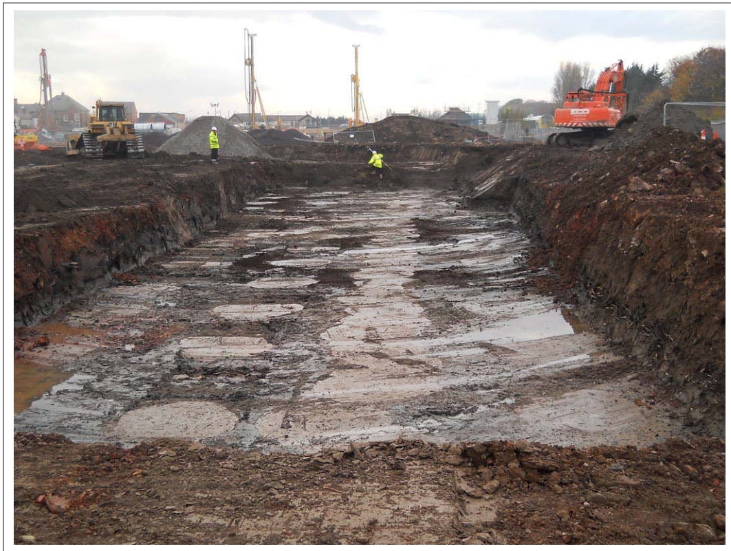
Plate 4: Post excavation view of Area 2, Note more consistent peat deposits within sections
