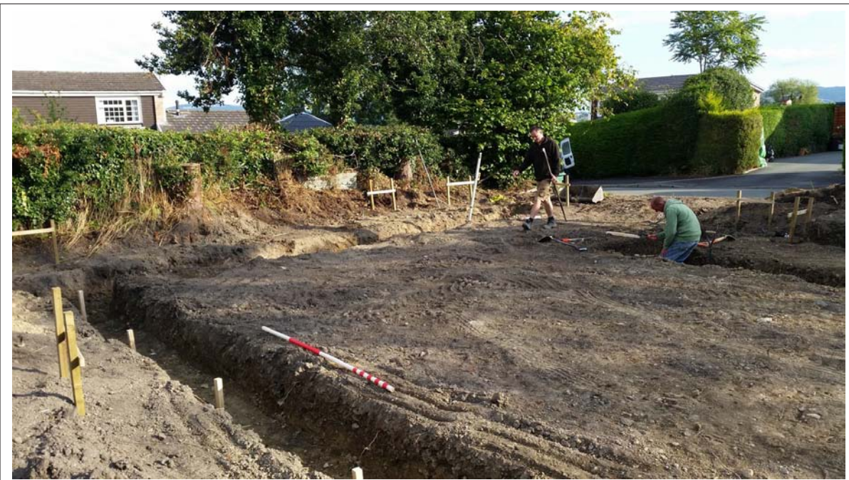
Plate 6: View north west across assessment area after cutting of foundation trenches Scale 1x2m
