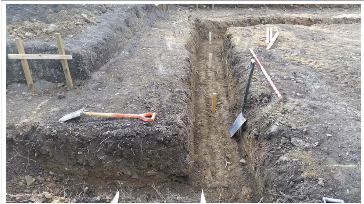
Plate 7: Example view of foundation trench showing dimensions/depth, Looking north west. Scale 1x2m
