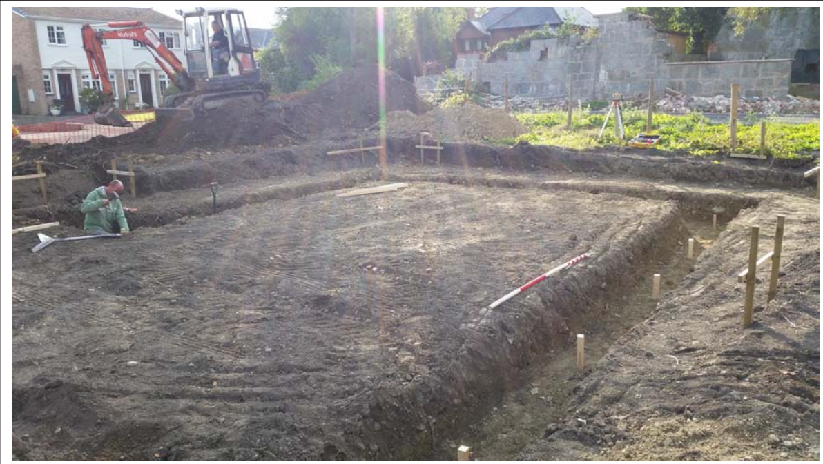
Plate 5: View north east across assessment area after cutting of foundation trenches Scale 1x2m
