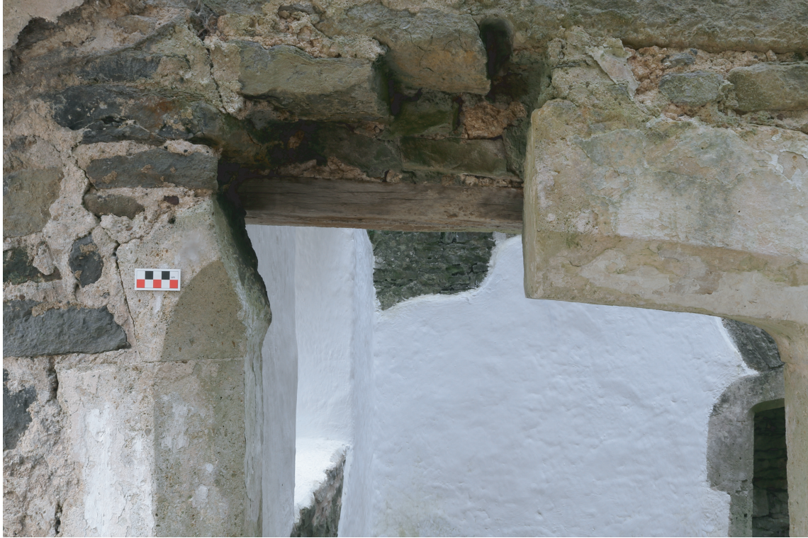
Plate 08. Old Beaupre - View of missing header stone in doorway into western room of Gatehouse. Looking W.
