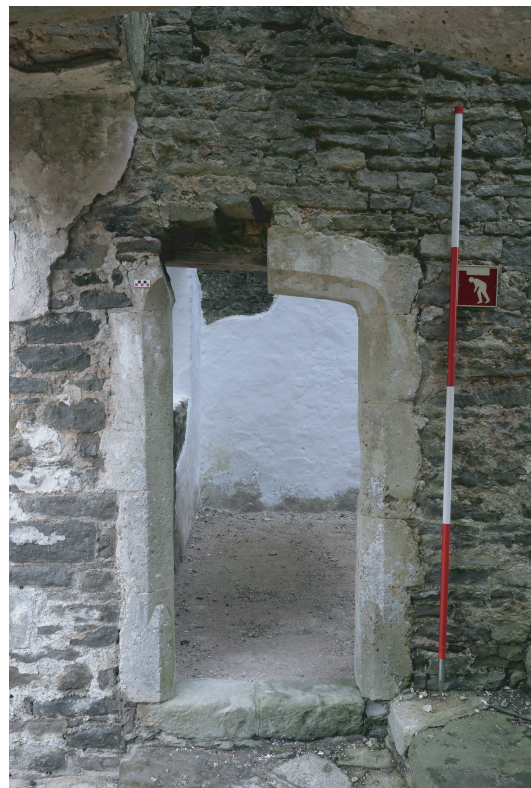
Plate 07. Old Beaupre - View of doorway into western room of Gatehouse. Looking W.
