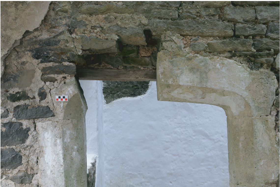
Plate 09. Old Beaupre - View of missing header stone in doorway into western room of Gatehouse. Looking W.
