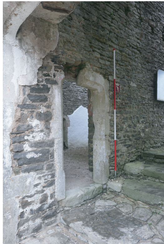
Plate 03. Old Beaupre - View of doorway into western room of Gatehouse. Looking NW.
