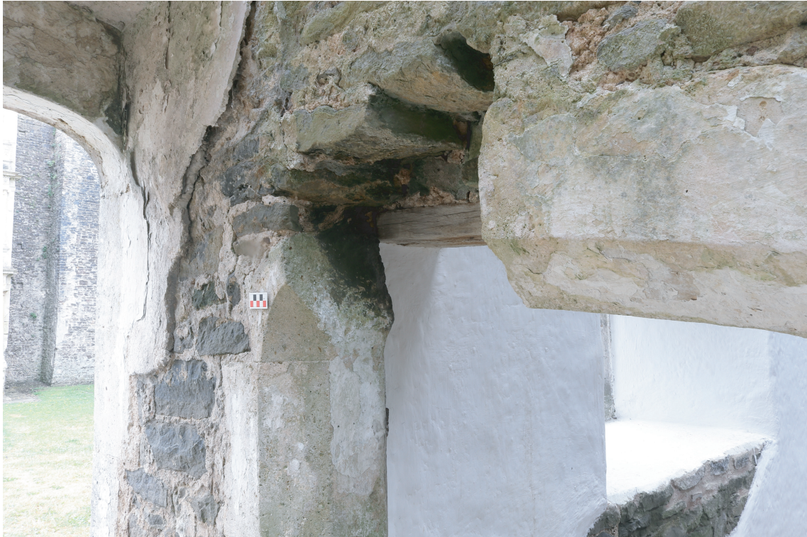
Plate 10. Old Beaupre - View of missing header stone in doorway into western room of Gatehouse. Looking SW.
