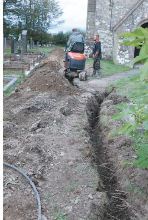
Plate 19. St. David's Church, Blaenporth - Working shot during initial cutting of water service trench at entrance of cemetery. Looking N.
