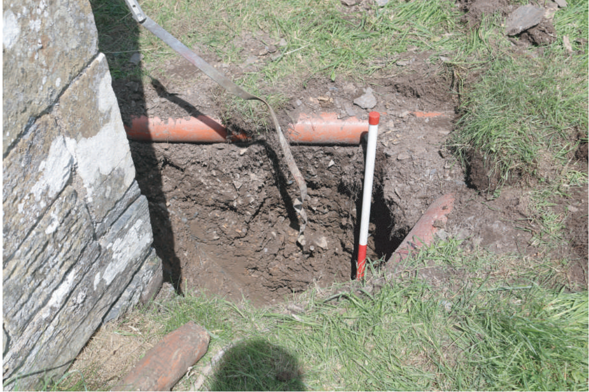
Plate 30. St. David's Church, Blaenporth - Completed Trench for Lightning Conductor Plate 2 at eastern corner of church. Looking N.
