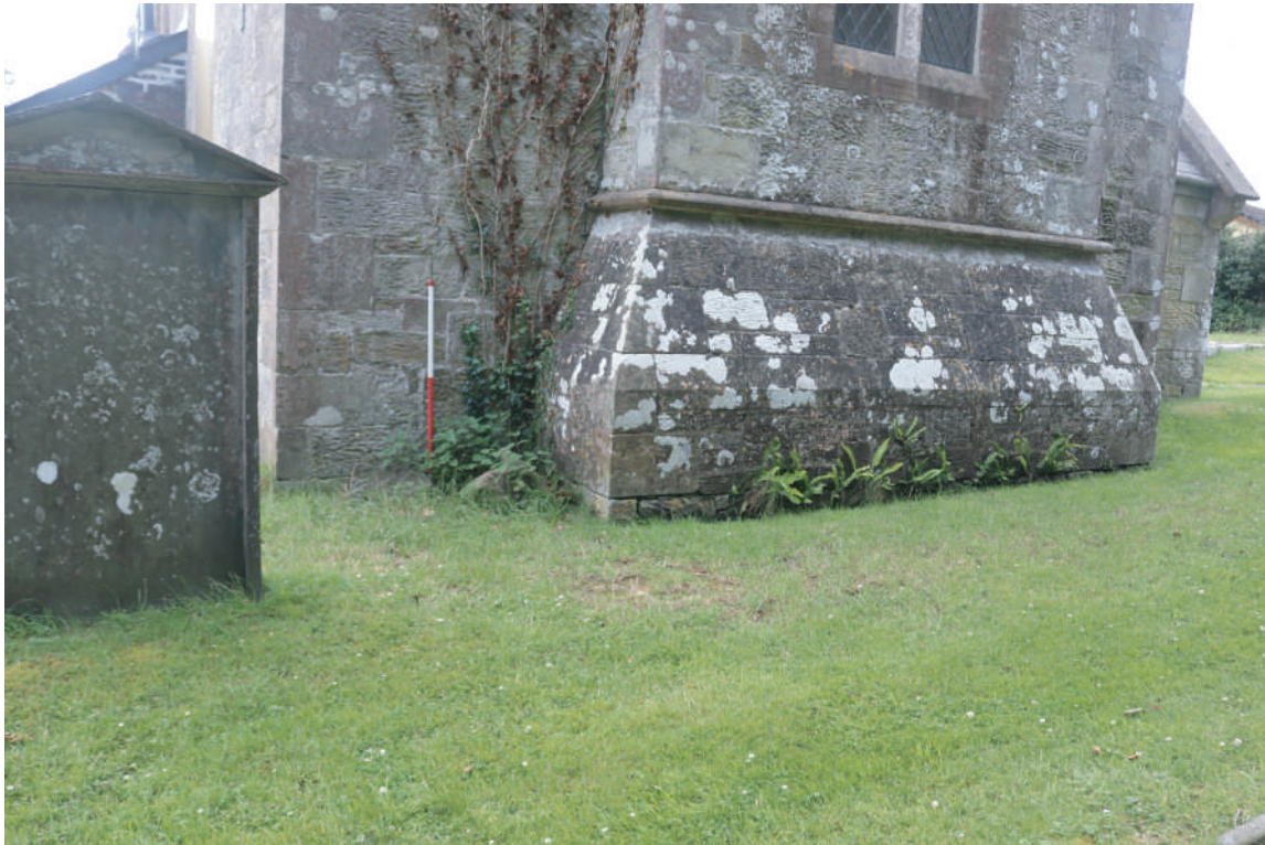
Plate 25. St. David's Church, Blaenporth - Position of proposed Lightning Conductor Plate 1. Looking E.
