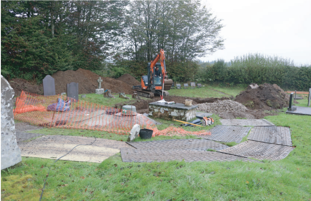
Plate 10. St. David's Church, Blaenporth - Working shot during ground work for drainage trench north of septic tank. Looking NE.
