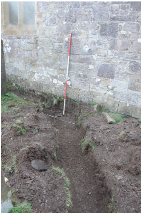
Plate 15. St. David's Church, Blaenporth - View of cut drainage trench alongside west end of church. Looking SE.
