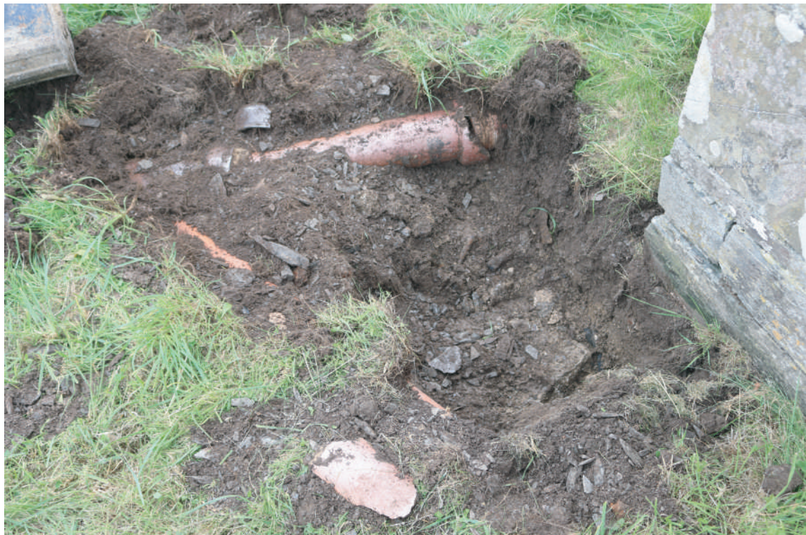
Plate 29. St. David's Church, Blaenporth - Working shot during cutting for Lightning Conductor Plate 2. Note 1930s/50s stone drainage pipe. Looking E.
