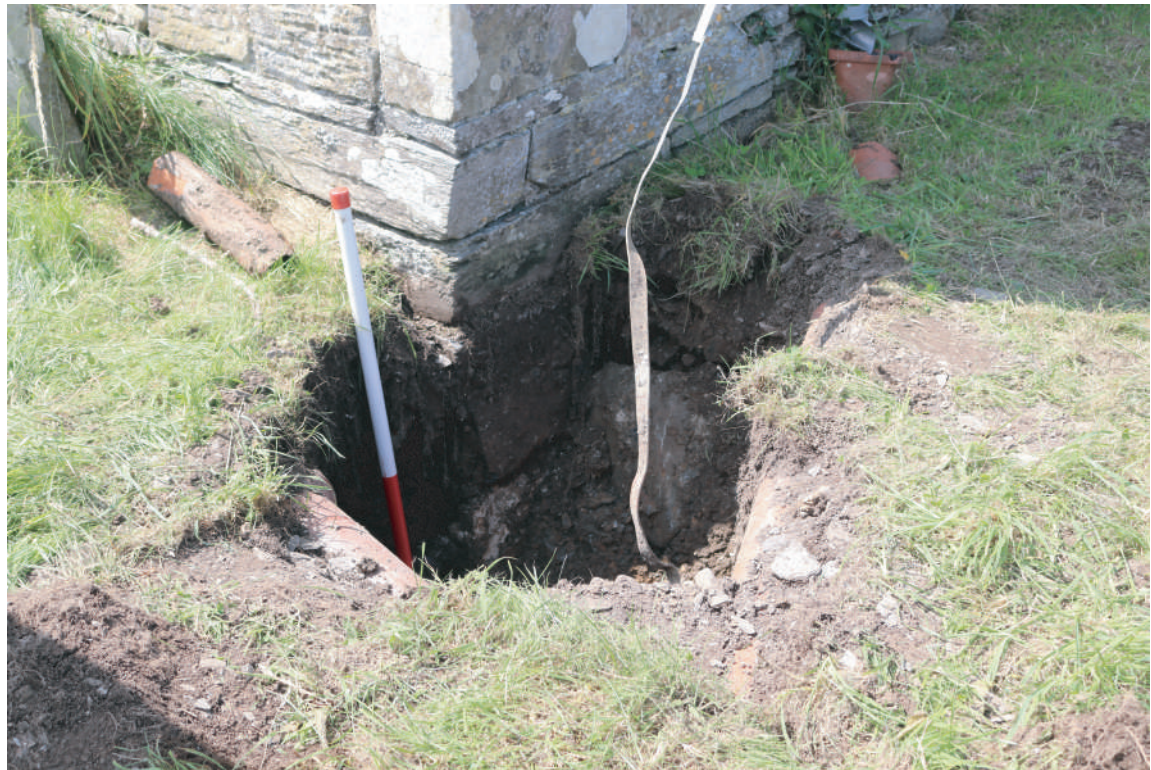
Plate 31. St. David's Church, Blaenporth - Completed Trench for Lightning Conductor Plate 2 at eastern corner of church. Looking SW.
