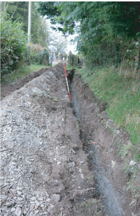
Plate 22. St. David's Church, Blaenporth - View of completed cut trench for proposed water pipe outside of cemetery entrance. Looking N.
