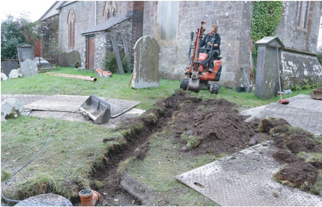
Plate 14. St. David's Church, Blaenporth - View of cut drainage trench from septic tank toward west end of church. Looking SE.
