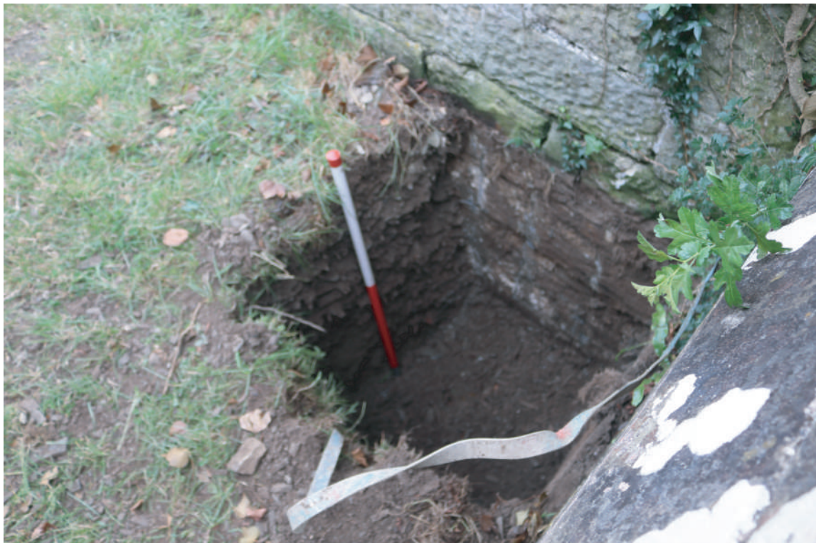
Plate 27. St. David's Church, Blaenporth - Completed Trench for Lightning Conductor Plate 1. Looking S.
