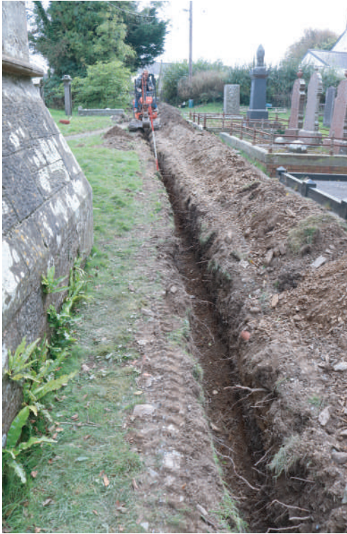
Plate 20. St. David's Church, Blaenporth - Working shot during cutting of water service trench from entrance of cemetery. Looking S.
