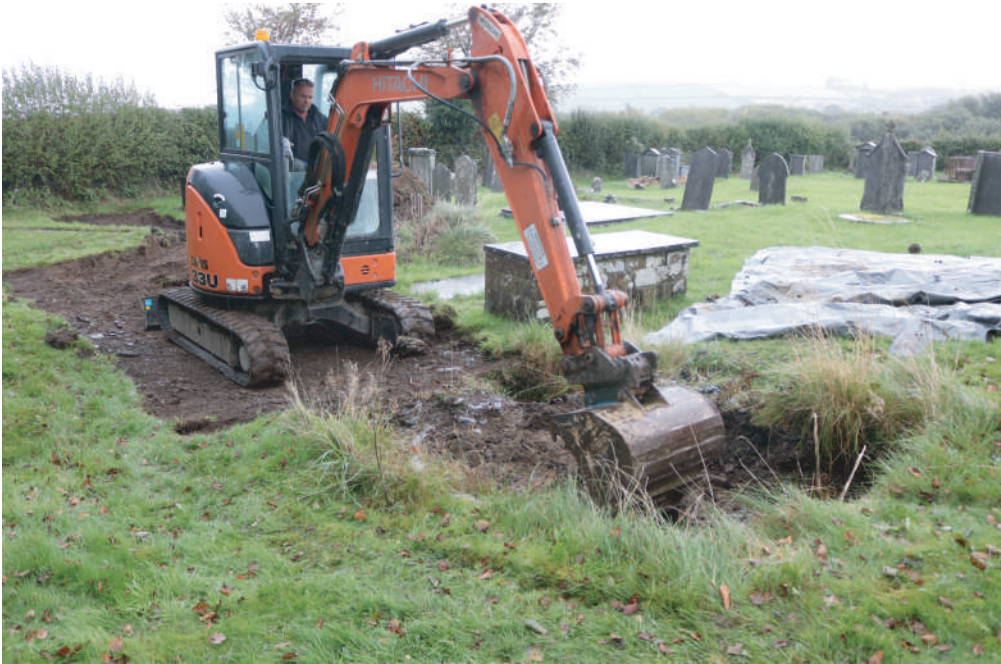
Plate 05. St. David's Church, Blaenporth - Ground work during excavation of area for septic tank. Looking NE.
