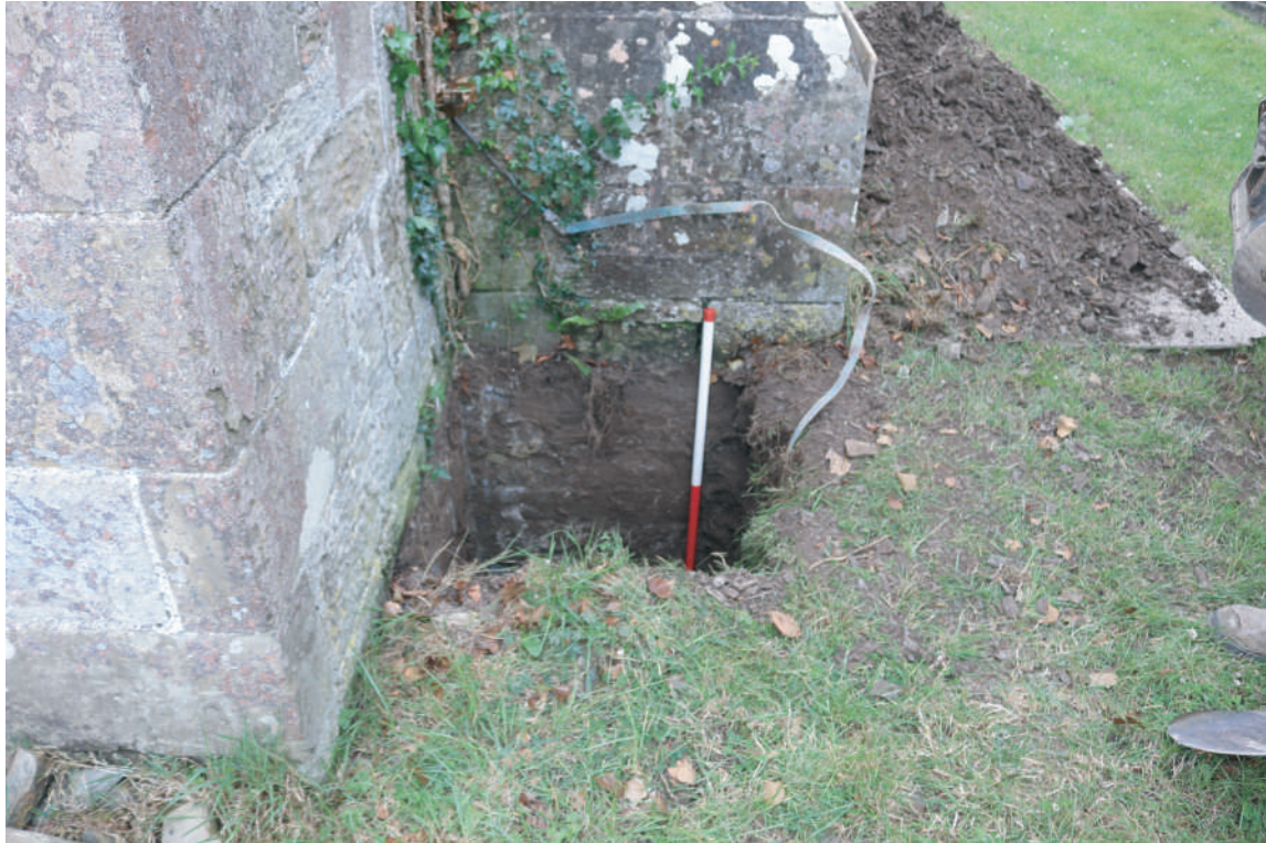
Plate 26. St. David's Church, Blaenporth - Completed Trench for Lightning Conductor Plate 1. Looking S.
