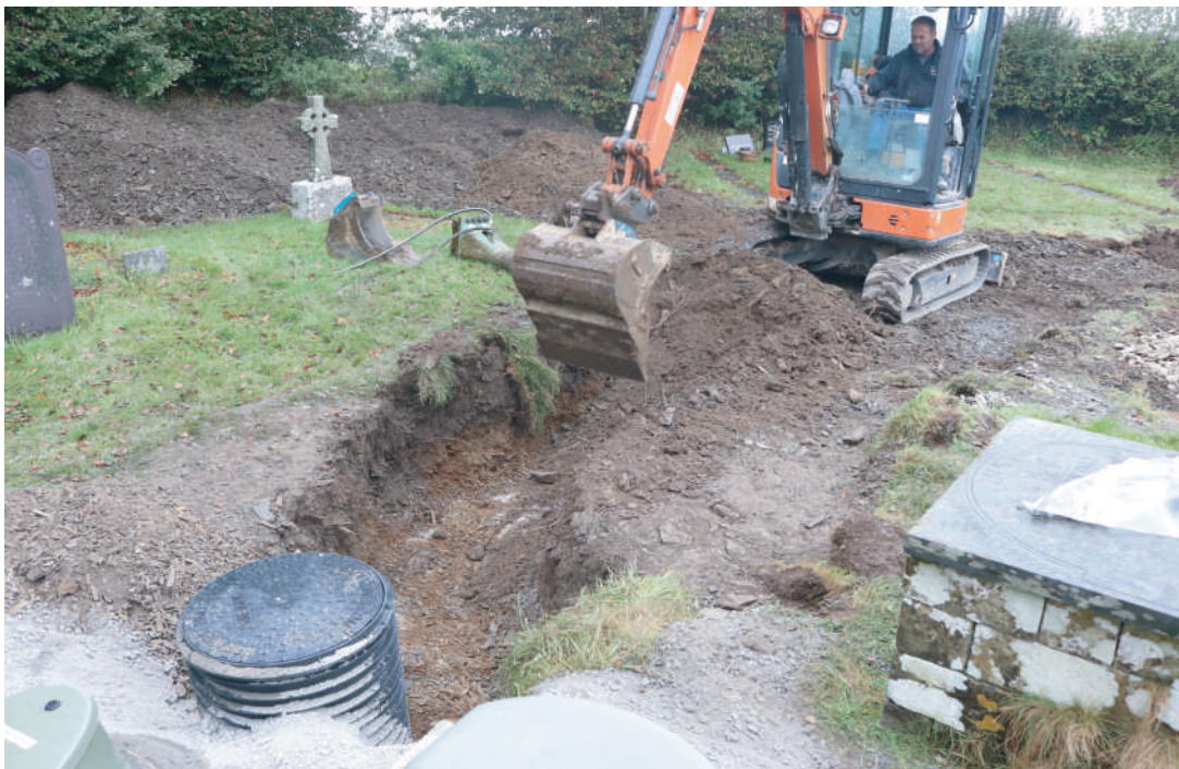
Plate 11. St. David's Church, Blaenporth - Working shot during ground work for drainage trench north of septic tank. Looking NW.
