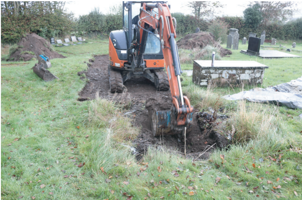
Plate 04. St. David's Church, Blaenporth - Working shot during groundwork for services. Looking North.
