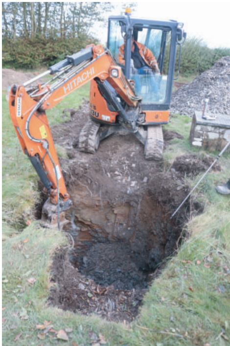
Plate 06. St. David's Church, Blaenporth - Ground work during for septic tank. Looking N.
