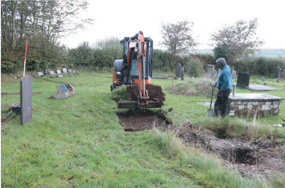
Plate 03. St. David's Church, Blaenporth - Working shot during groundwork for services. Looking North.
