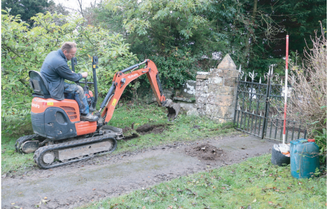
Plate 17. St. David's Church, Blaenporth - Working shot during initial cutting of water service trench at entrance of cemetery. Looking SE.
