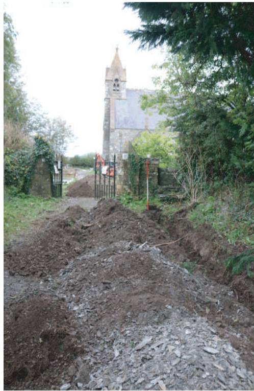
Plate 21. St. David's Church, Blaenporth - View of cut trench for proposed water pipe outside of cemetery entrance. Looking N.
