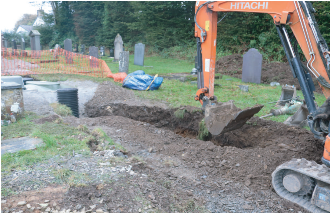
Plate 12. St. David's Church, Blaenporth - Working shot during ground work for drainage trench north of septic tank. Looking SW.
