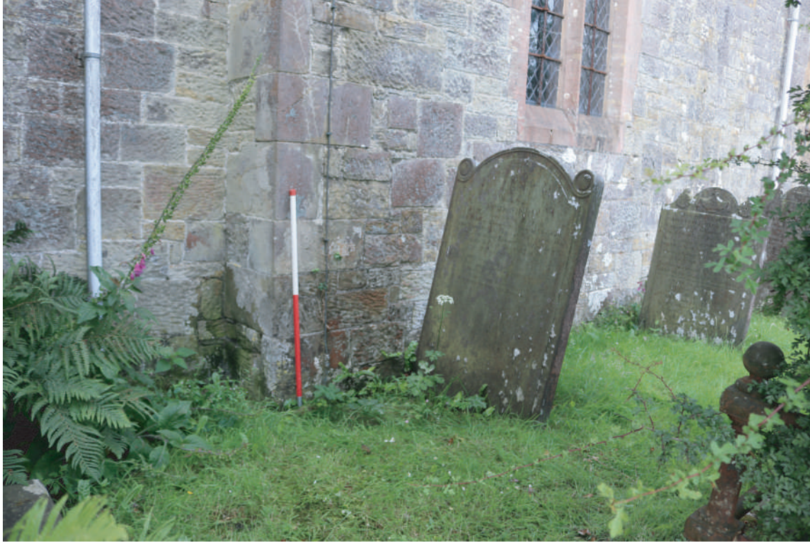
Plate 32. St. David's Church, Blaenporth - Location of Trench for Lightning Conductor Plate 3 on west side of Vestry. Looking SW..
