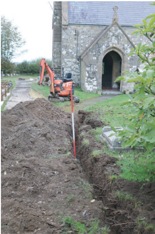
Plate 18. St. David's Church, Blaenporth - Working shot during initial cutting of water service trench at entrance of cemetery. Looking N.
