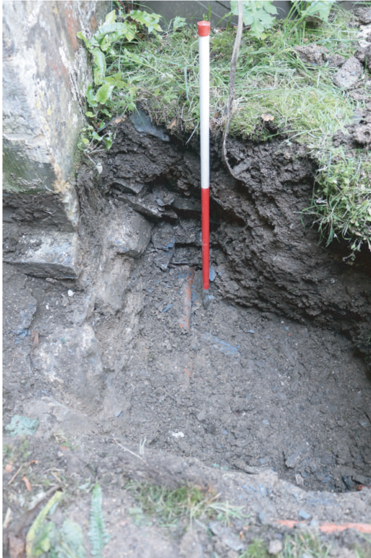
Plate 34. St. David's Church, Blaenporth - East facing section of completed Trench for Lightning Conductor Plate 3 on west side of Vestry. Looking W.
