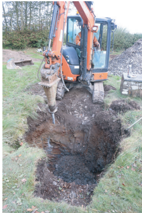
Plate 07. St. David's Church, Blaenporth - Ground work during for septic tank. Looking N.
