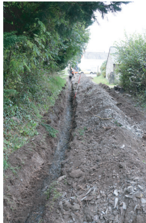
Plate 23. St. David's Church, Blaenporth - View of completed cut trench for proposed water pipe outside of cemetery entrance. Looking S.
