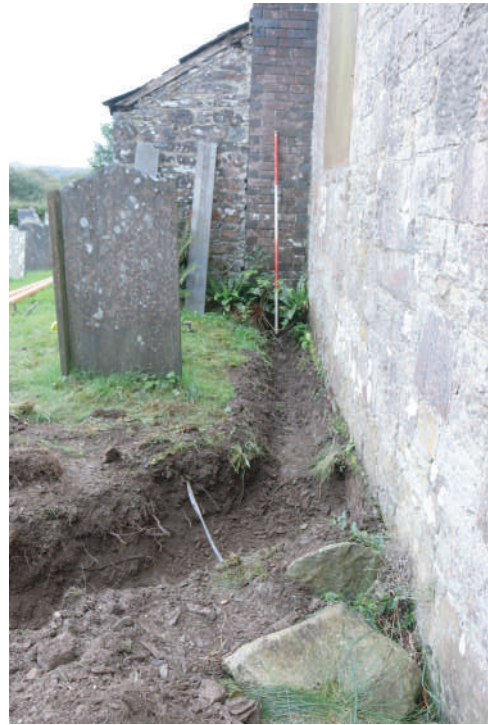
Plate 16. St. David's Church, Blaenporth - View of cut drainage trench alongside west end of church. Looking E.
