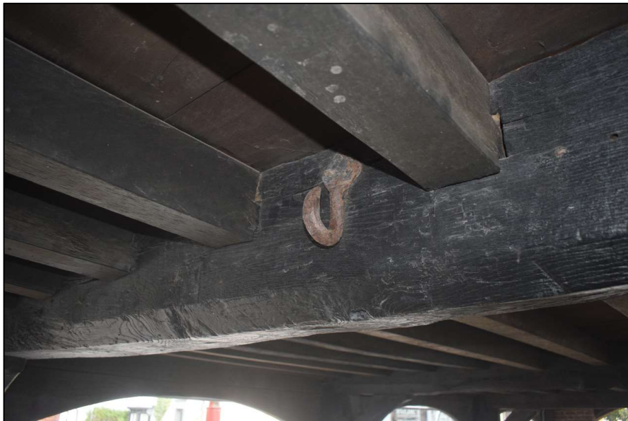
Fig. 8 Hook attached to beam at southern end of covered market. Photo CPAT 5096-019
