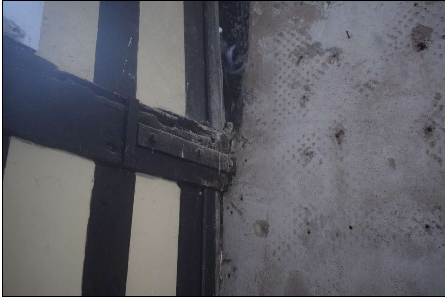
Fig. 11 Bracket attaching stonework of the south elevation to the timber frame Photo CPAT 5096-048
