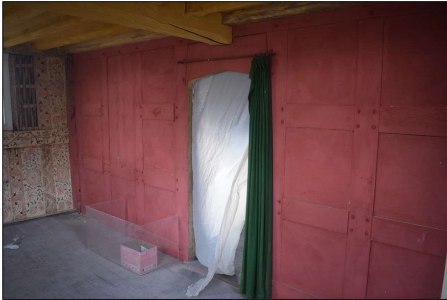
Fig. 15 View south of the doorway and timber framed partition between the room at the north end of the building and the main hall Photo CPAT 5096-033
