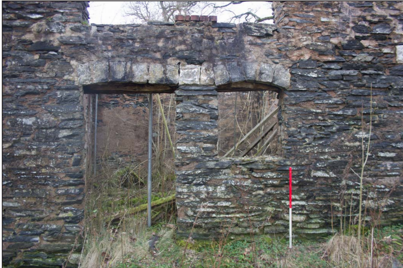
Plate 11: East facing external elevation showing doorway to Room 1, from the east. Scale 1.0m.
