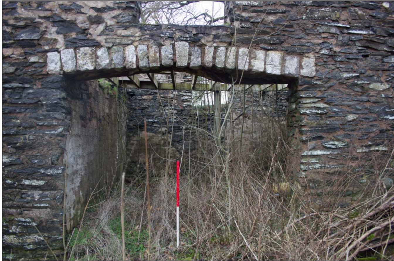
Plate 12: East facing external elevation showing cart door to Room 2, from the east. Scale 1.0m.
