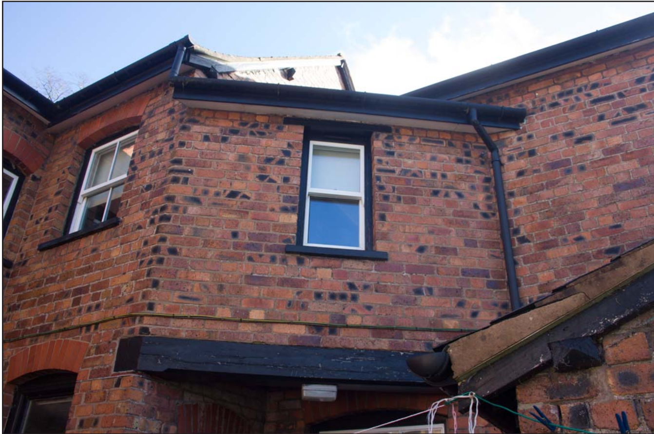
Plate 12: First Floor, side access of Compton House, 10 Station Avenue, Chirk, Wrexham - from the west - no scale
