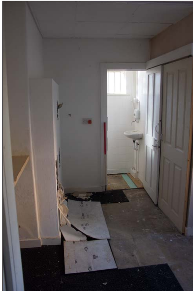
Plate 19: Rear Room of Compton House, 10 Station Avenue, Chirk, Wrexham - from the north - 1.00m scale
