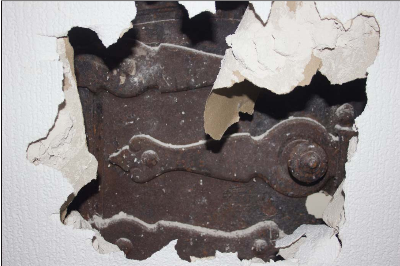
Plate 22: View through modern wall (2) showing former stove in Rear Room of Compton House, 10 Station Avenue, Chirk, Wrexham - from the west - no scale
