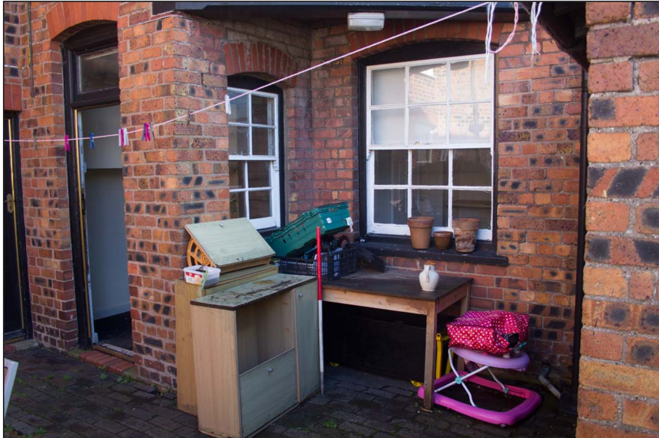
Plate 13: Side door (oblique view) of Compton House, 10 Station Avenue, Chirk, Wrexham - from the west - 1.00m scale
