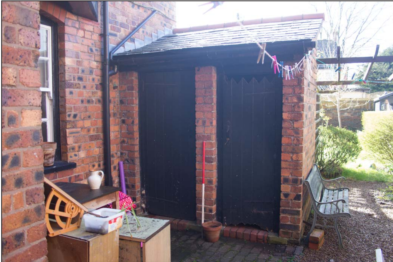
Plate 14: Outside stores (former outhouses) of Compton House, 10 Station Avenue, Chirk, Wrexham - from the northwest - 1.00m scale
