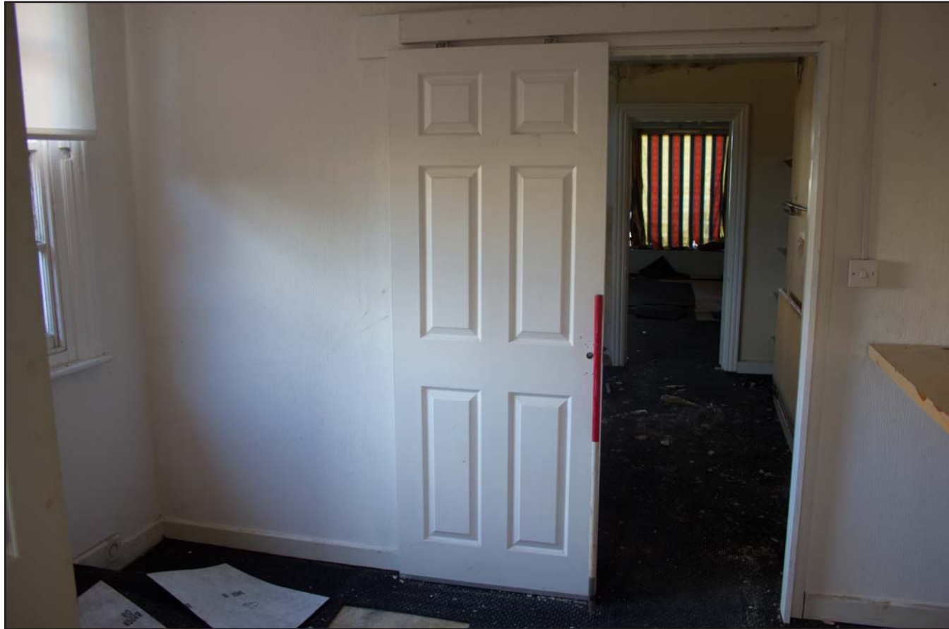
Plate 20: Rear Room (view to front) of Compton House, 10 Station Avenue, Chirk, Wrexham - from the south - 1.00m scale
