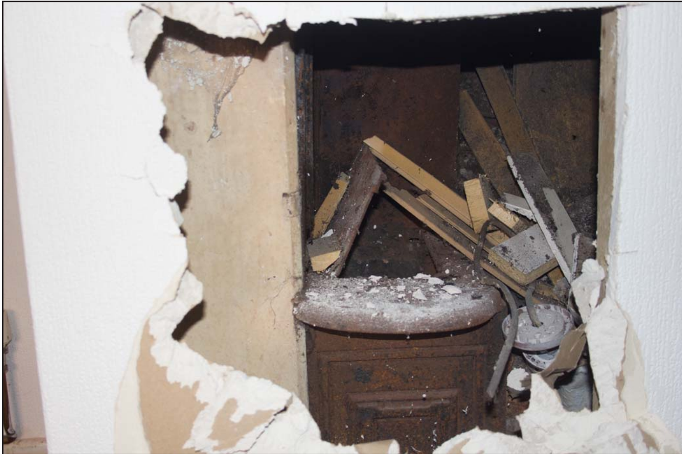
Plate 21: View through modern wall (1) showing former stove in Rear Room of Compton House, 10 Station Avenue, Chirk, Wrexham - from the west - no scale
