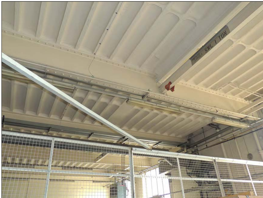
Plate 97. View of the concrete ceiling in the garage, looking upwards to the E
