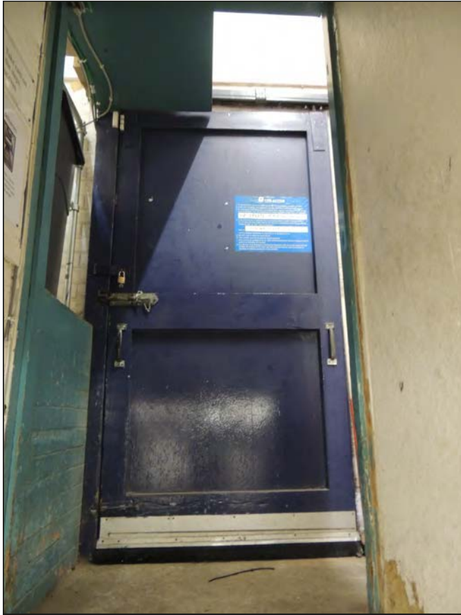
Plate 54. View from cellar towards blue wooden sliding door in the beer store looking SW
