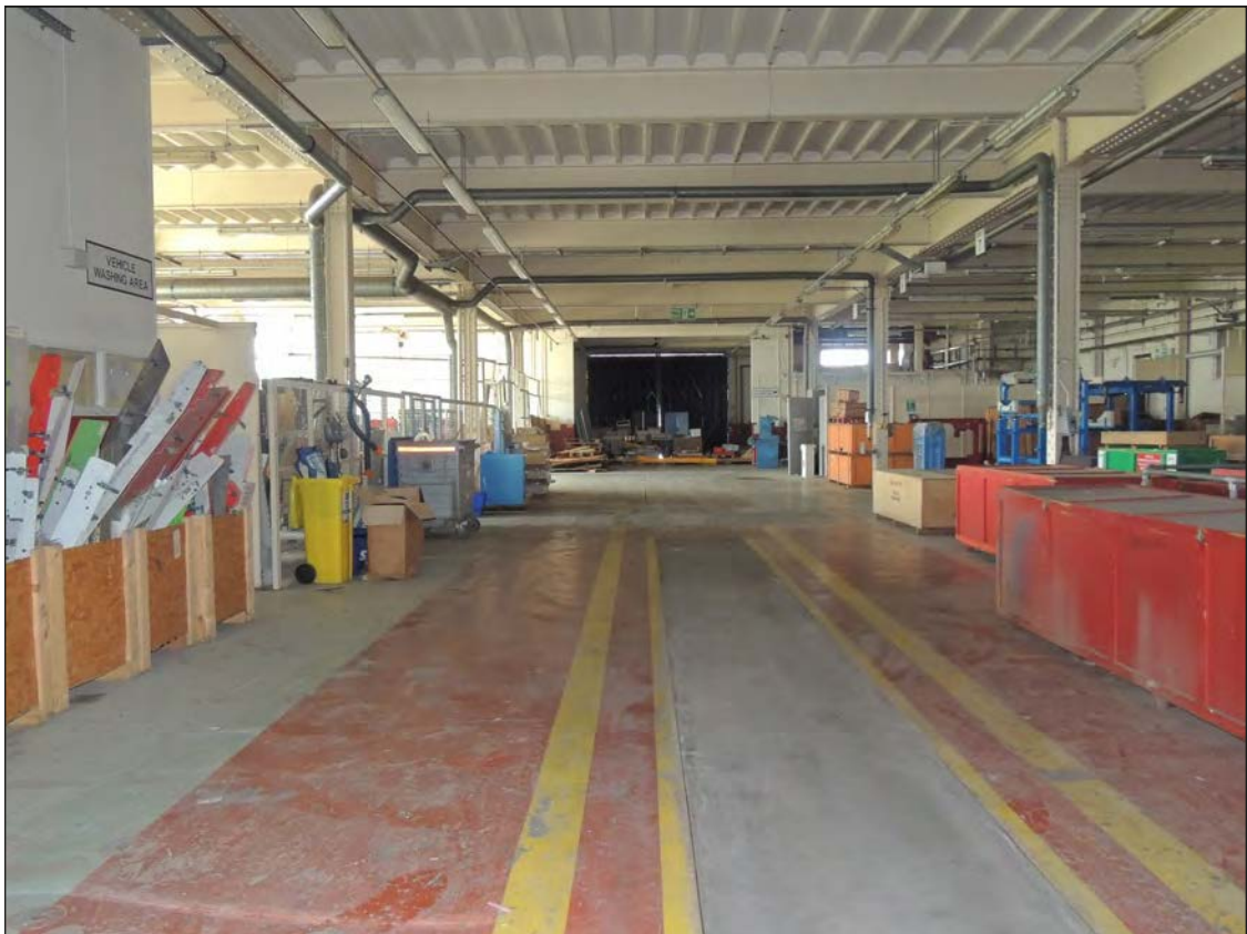
Plate 93. View of the garage with concrete infilled vehicle pit on the floor looking SSE
