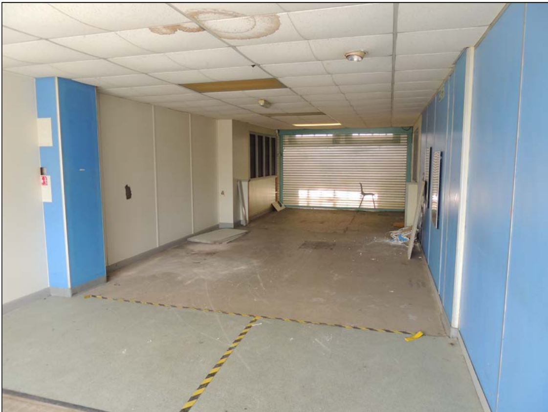
Plate 132. View of food hall that has been sub-divided into office space, looking NE
