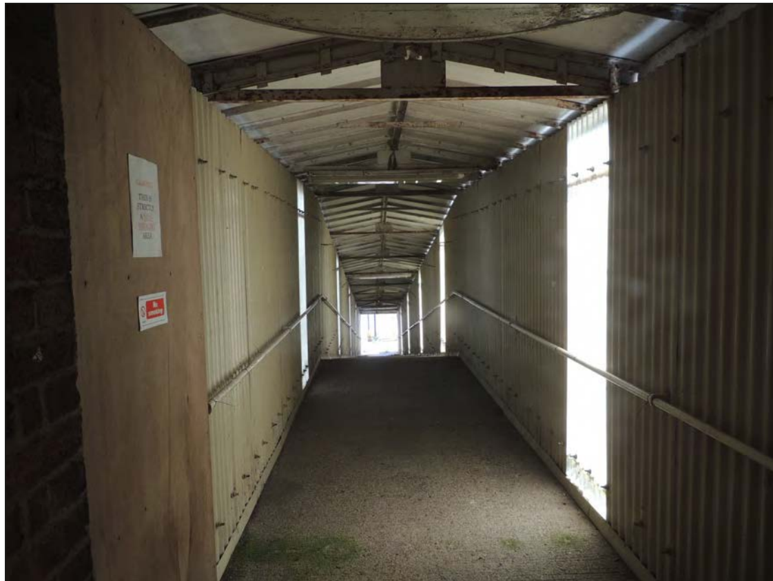
Plate 118. View of an access ramp leading to a SE entrance from the carpark, looking SE
