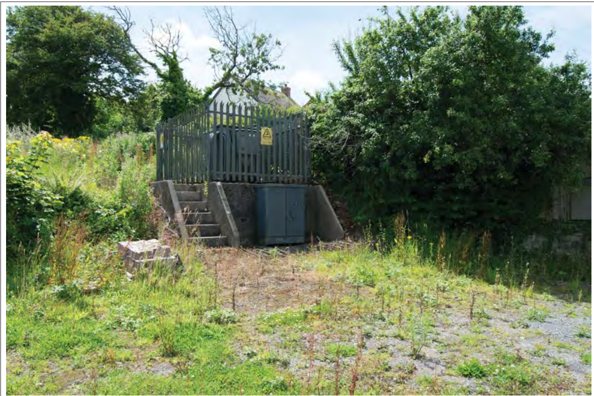
Plate 8. The electrical substation in the central area. View west.
