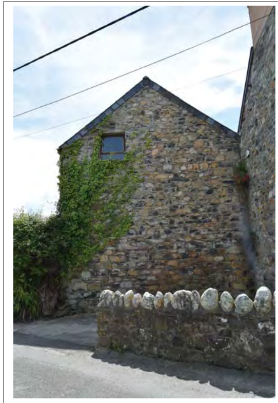
Plate 23. Northern gable wall of the The Pottery, with Grade II listed Trem y Don adjoining on the right. View south.
