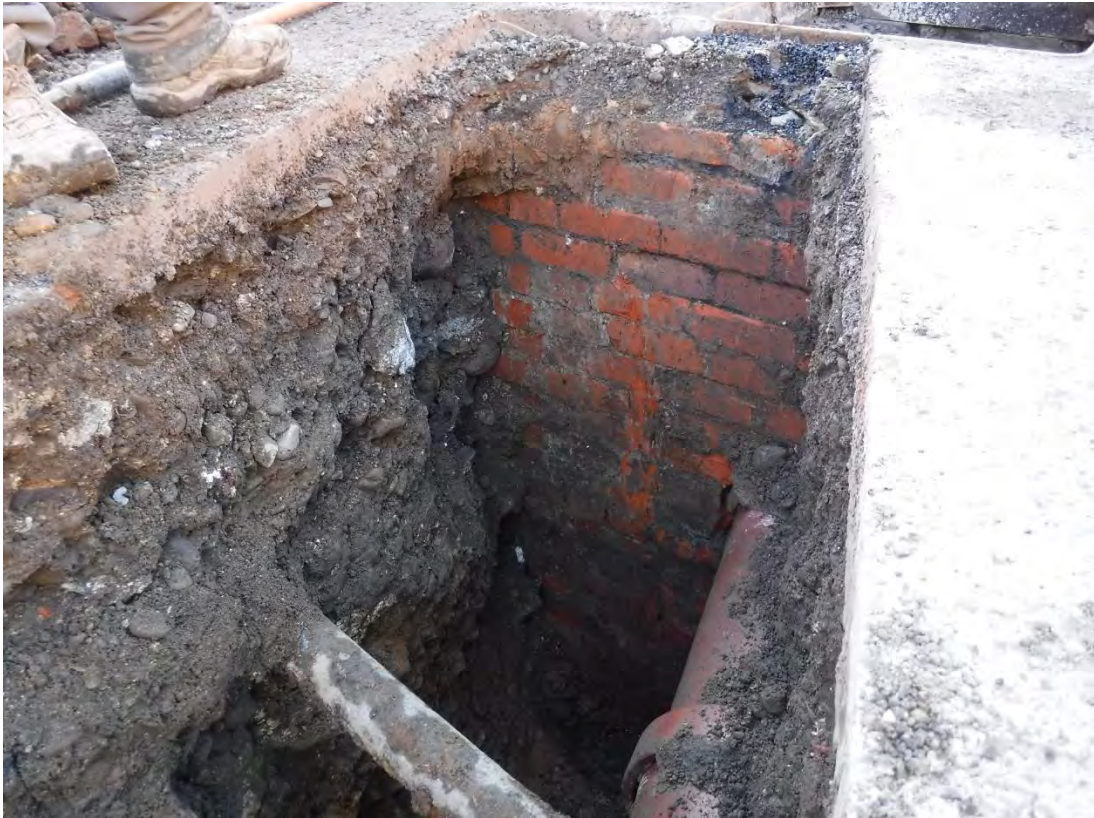
Photo 3: Shot facing southwest, showing the inspection chamber at the start of Trench 1.
