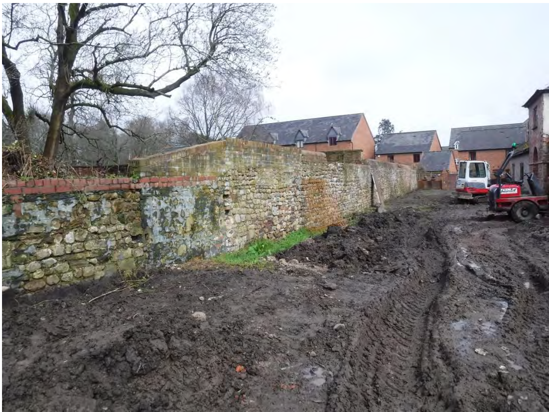
Photo 34: General shot facing east, showing the area in front (north) of the Laundry Building and the enclosure wall.
