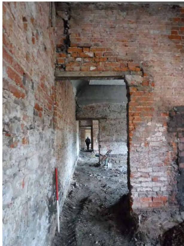
Photo 18: Phase 2 works within the Laundry Building. Shot facing west looking along the southern wall of the building. 1m scale.
