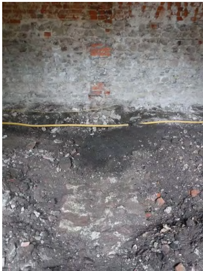
Photo 30; Laundry Building, Room 4. Shot facing south, showing wall remains (171), the former doorway gap beyond, and remnants of the internal wall attachment to the southern wall beyond.
