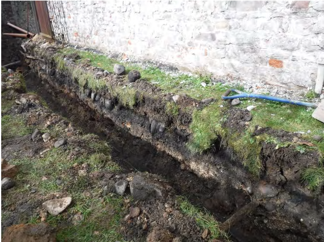
Photo 11: Trench 1 as it runs along the southern side of the Laundry Building. Shot facing northwest, showing large stone layer (142/202) below the turf to the left.
