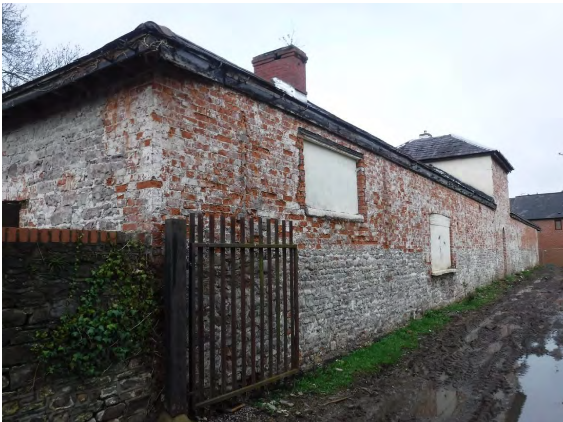
Photo 10: General shot facing northeast, showing the southern side of the Laundry Building.
