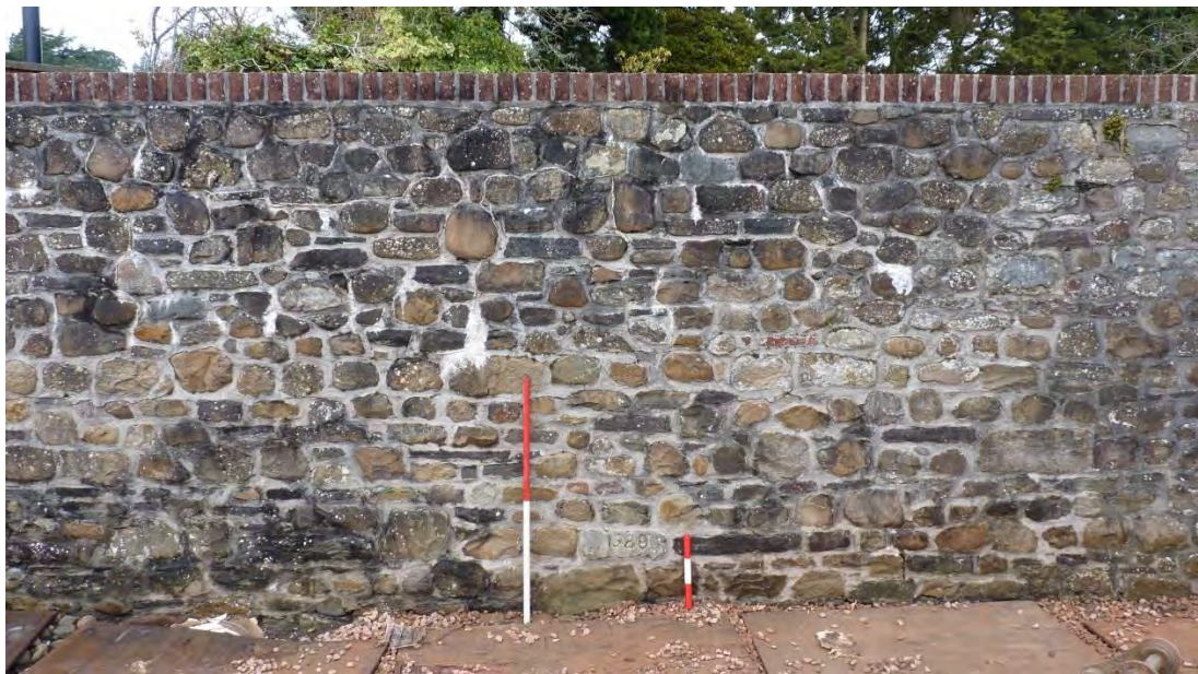
Photo 42: Boundary wall between the main yard to the south, and the Laundry Building yard to the north, shot facing north. Date stone '1928' at base of wall between scales. 1m & 0.3m scales.
