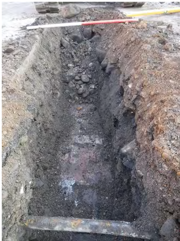
Photo 6: Trench 1, shot facing northeast showing Drain/Culvert 122 crossing the base of the trench. 1m scale.
