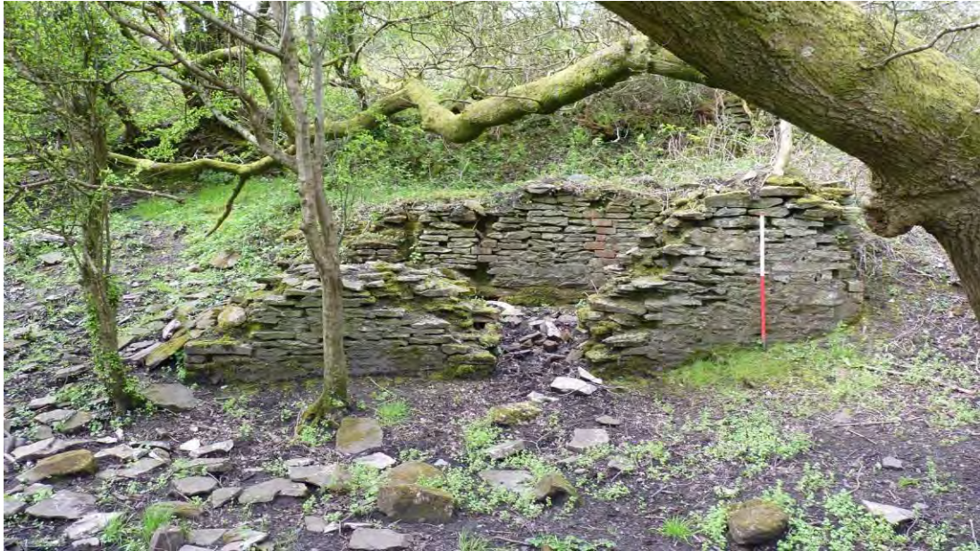
Photo 25: Remains of the lower structure associated with Trawsdy (LPN05), lying outside the area of proposed development. 1m scale.
