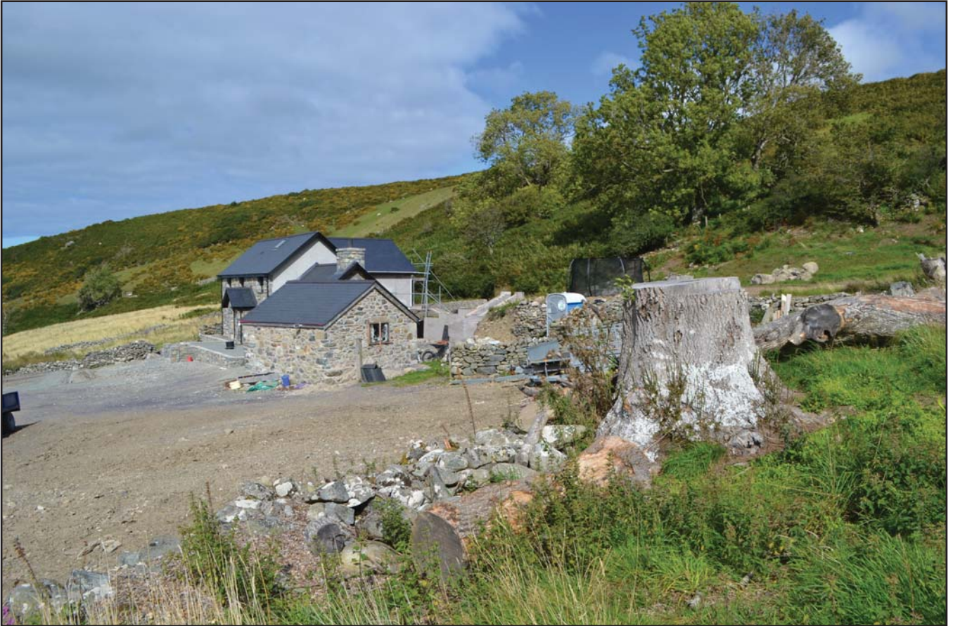
Plate 01: View of the location of the proposed barn, viewed from the SW (archive ref: G2783_HASIA_022).
