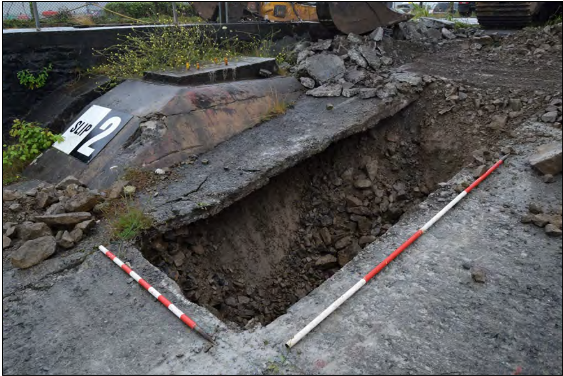
Plate 29: STP213 mid excavation, looking SE showing winch or anchor point [2135], view to SE, 1m & 2m scales.
