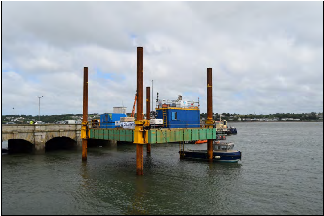
Plate 5: Offshore drilling rig at high tide with Carr Jetty behind, View to the NW.
