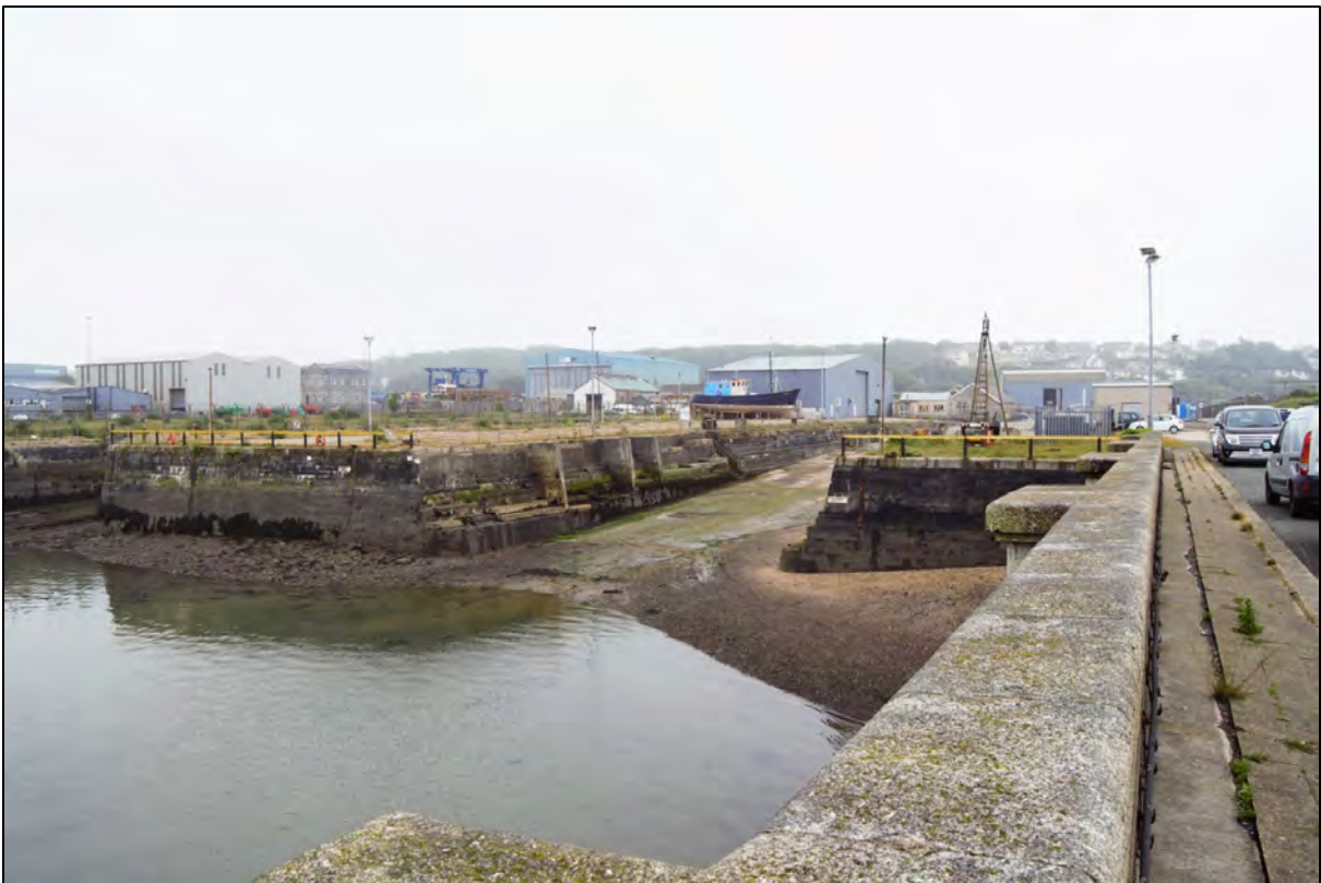
Plate 2: Overview of the site taken from Carr Jetty showing Slipway 1 (centre) and Slipway 2 (left), View to the S.
