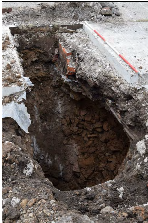
Plate 22: STP208 concrete sloping wall (2087) and brick culvert [2084], view to the North, 2m scale.
