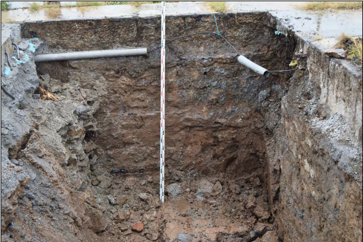
Plate 43: CPWIT East, detail of west face of western wall of Slipway 2, view to the east, 3m scale.
