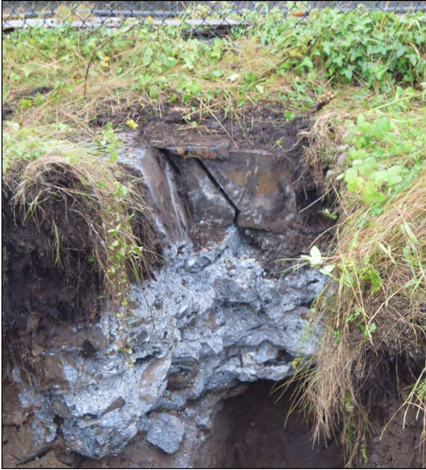
Plate 31: STP215 eastern wall of Slipway 2 [2153] detail of dressed masonry, view to the west.
