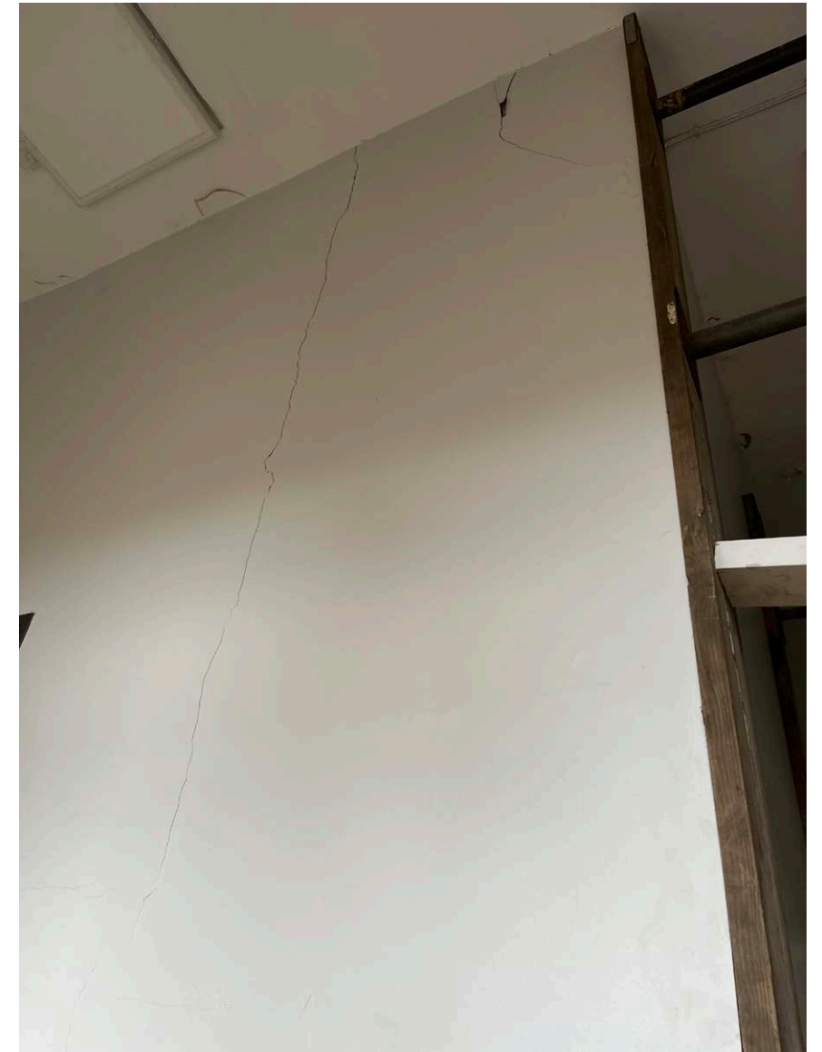
View of existing cracks to blockwork wall
