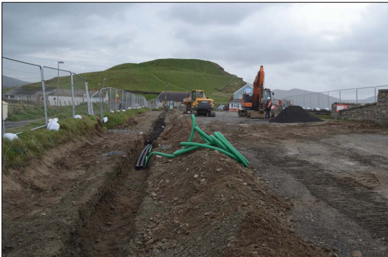
Plate 9: General shot of the cable trench being excavated; scale not used; view from N (archive reference: G2813_012).
