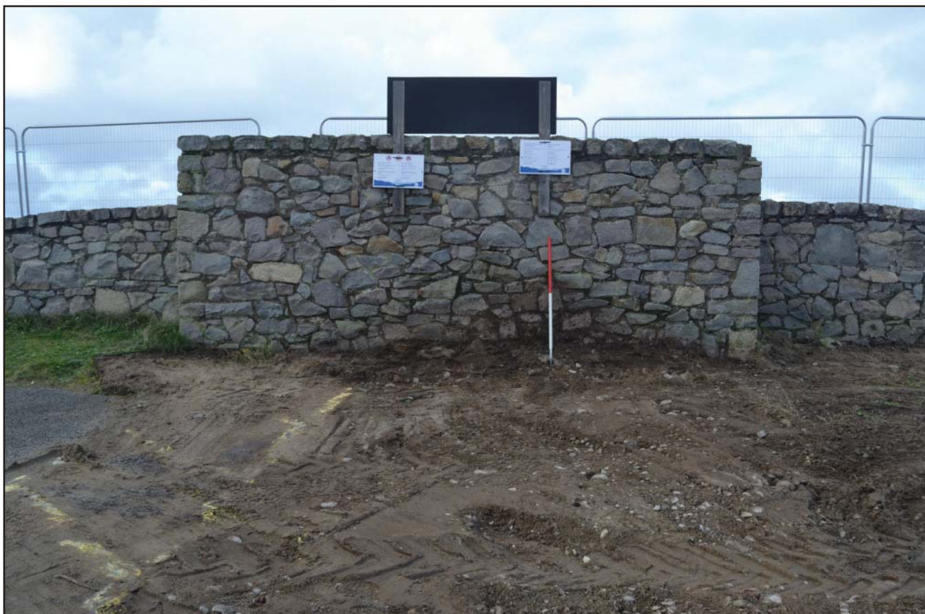
Plate 4: Shot showing wall/sea defence with mound removed. Location of new pay and display machine; scale 1m; view from E (archive reference: G2813_005).
