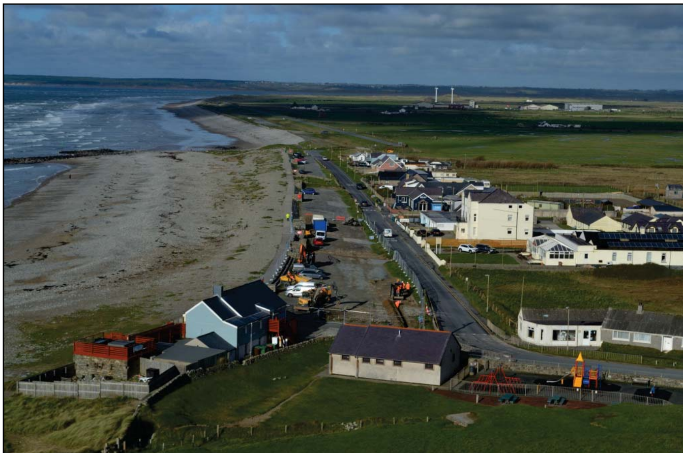
Plate 7: General shot of works area taken from elevated position from outer rampart of Dinas Dinlle hillfort (CN 048); scale not used; view from S (archive reference: G2813_010).
