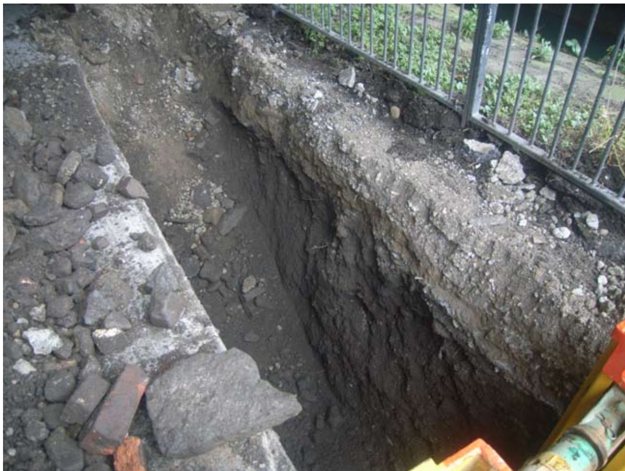
Plate 14: Deposits below road bridge
