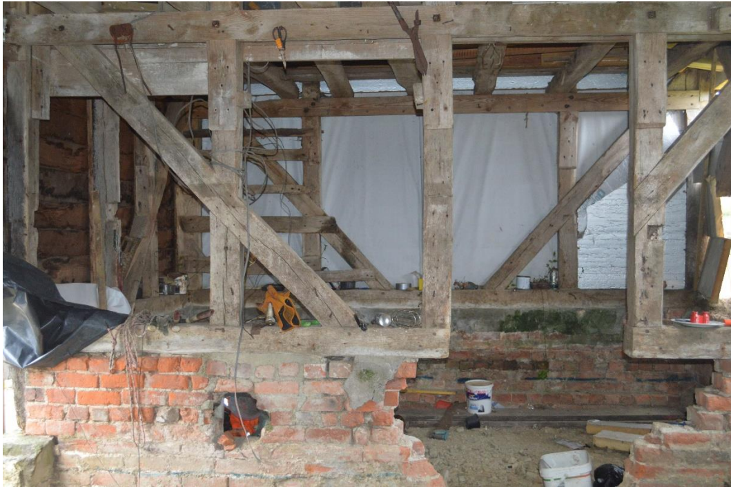
Figure 20: the wall of loose box. Doorway cut into beams with part of the wall demolished. Facing west. CPAT 5046_0028
