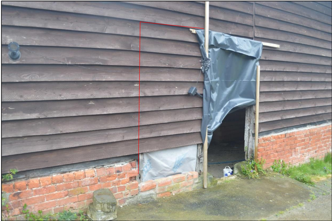
Figure 12: Doorway on south wall with blocked up doorway visible to the left (outlined in red). Facing north east. CPAT 5046_0062
