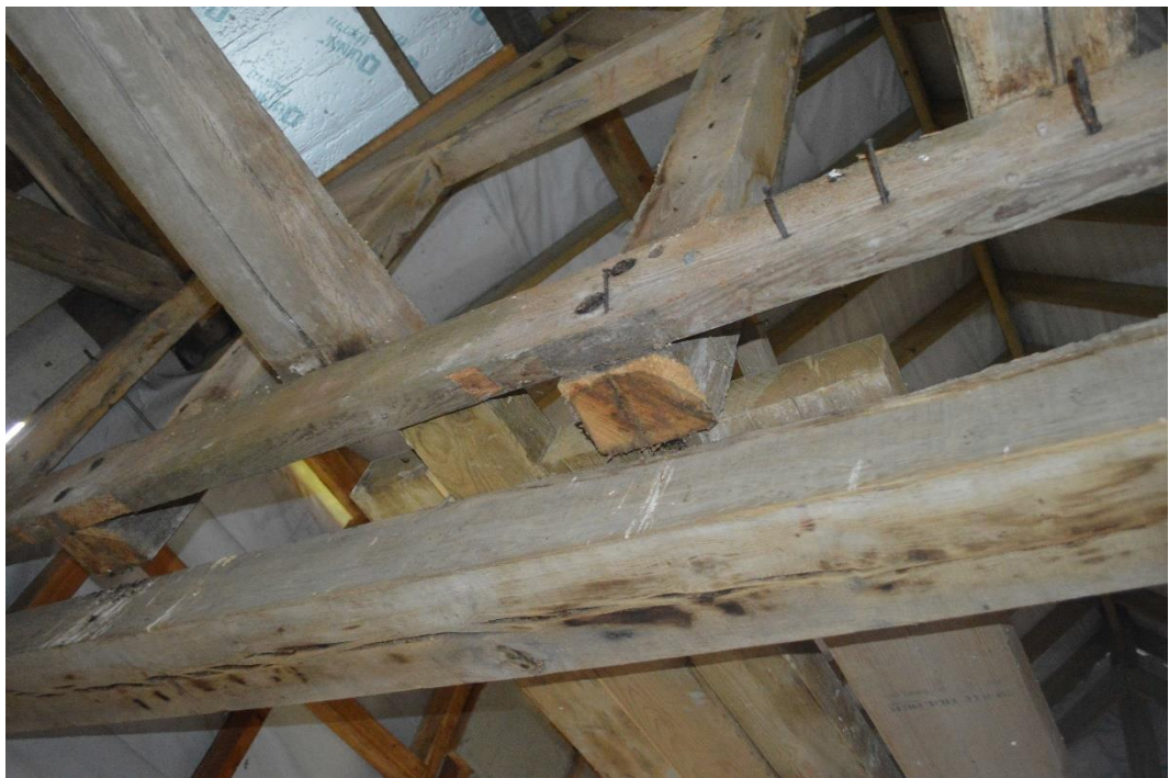
Figure 27: cut beam at base of queen post to allow for the extension to the barn. Facing north east. CPAT 5046_0098
