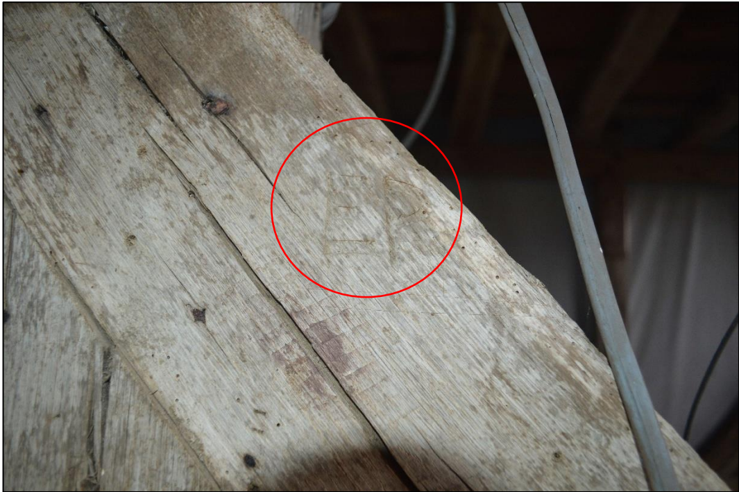
Figure 22: Initials carved into wooden frame of loose box next to exterior entrance doorway into main barn. Facing west. CPAT 5046_0091
