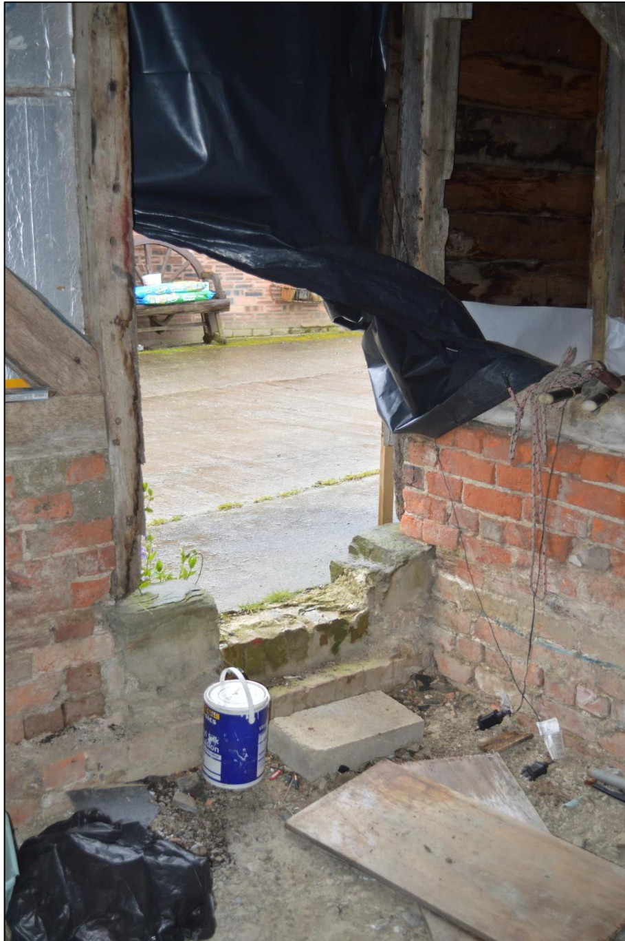
Figure 15: External doorway into barn. Brick wall with wooden frame on top visible to the right. Facing south-west. CPAT 5046_0001
