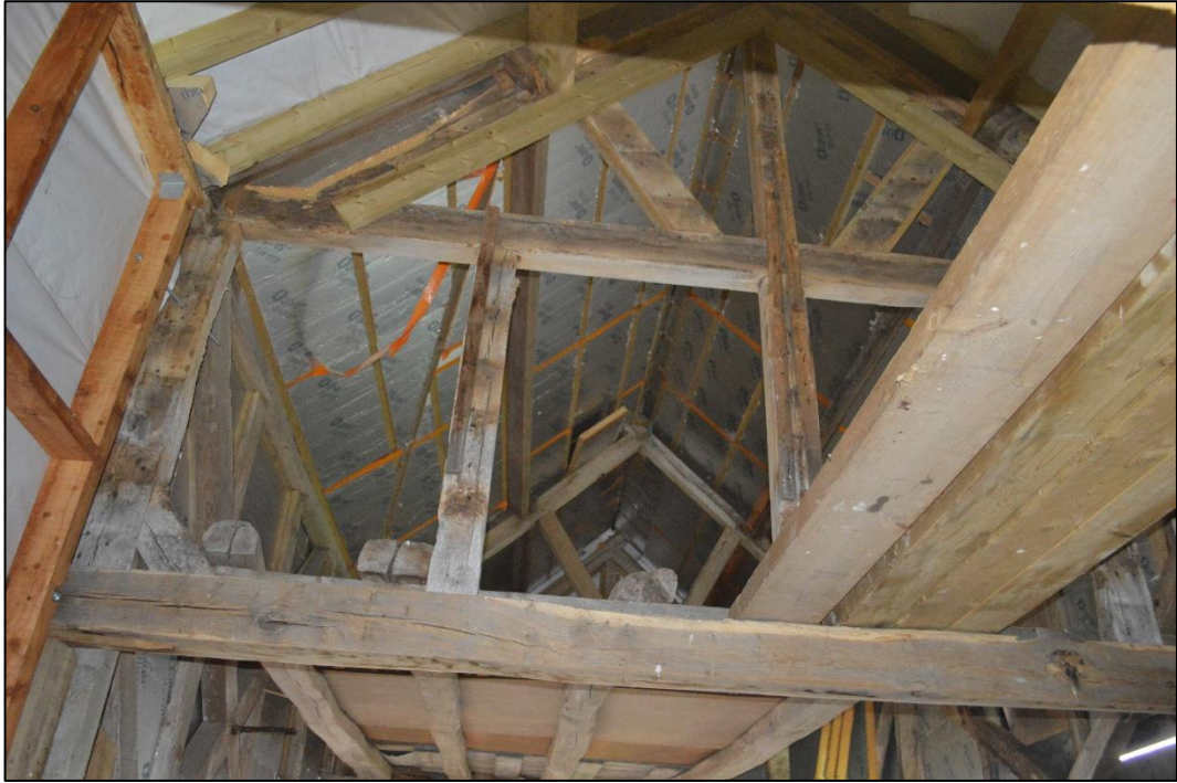
Figure 26: king post of roof towards west gable. Queen post from original east gable of barn visible in background. Facing east. CPAT 5046_0095
