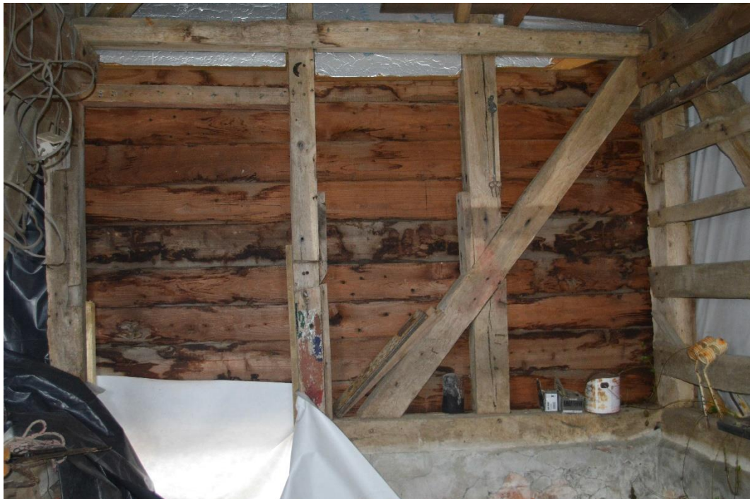
Figure 21: South wall of loose box. Wooden weatherboard panelling visible with blocked up original doorway to the left. Facing south. CPAT 5046_0040
