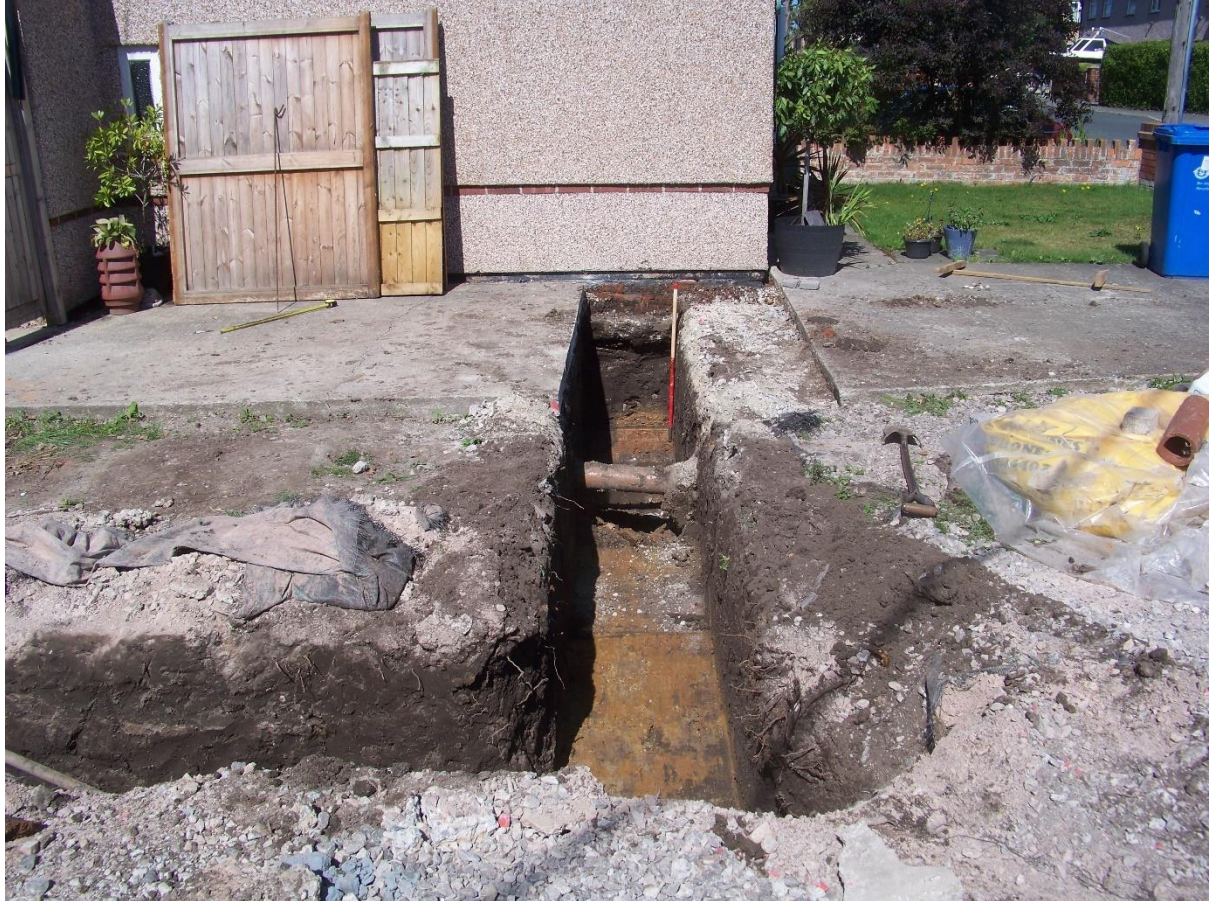
Figure 7 Pipe line visible in eastern footing (note yellow natural sand geology at base of trench)
