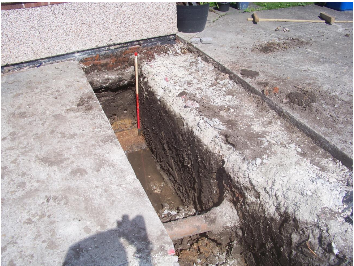
Figure 6 Potential ditch or pit in the eastern footing with water quickly filling it
