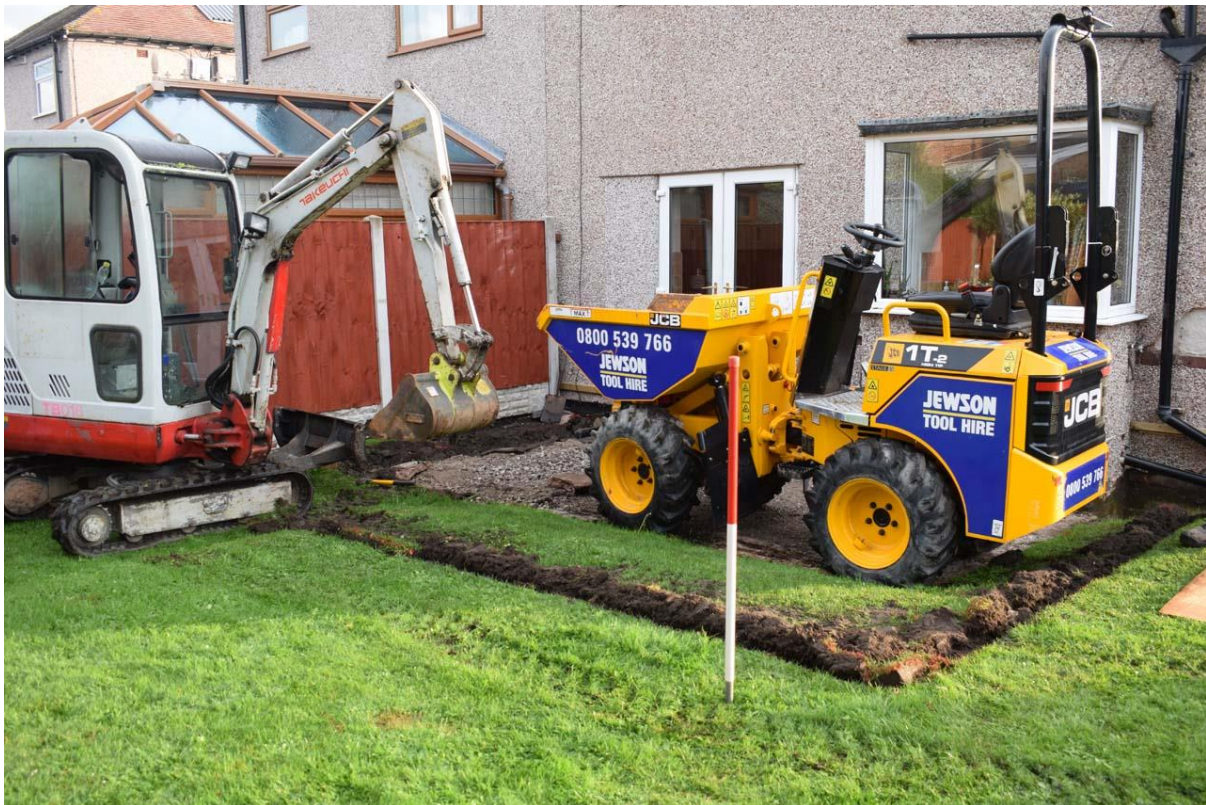
Fig. 3 Extent of excavation area (marked by turf cut/red line) viewed from the south west. CPAT photo 4953-0001
