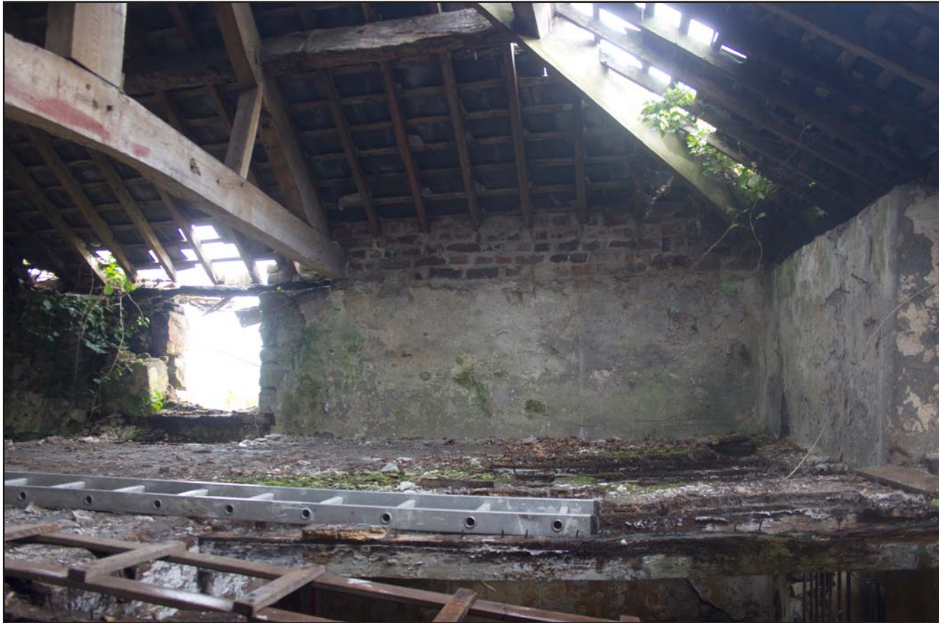
Plate 45: Internal shot of Hayloft, Estate Offices & Stables, Trevor Road, Chirk - from the east - no scale
