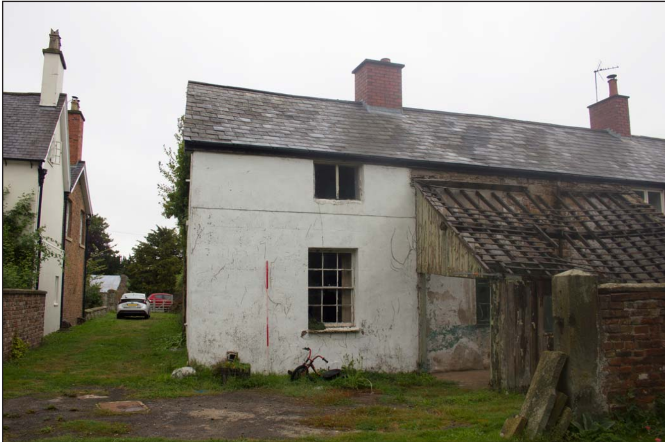
Plate 14: Southern elevation (wide), former Estate Offices & Workshop, Trevor Road, Chirk - from the south - 2.00m scale
