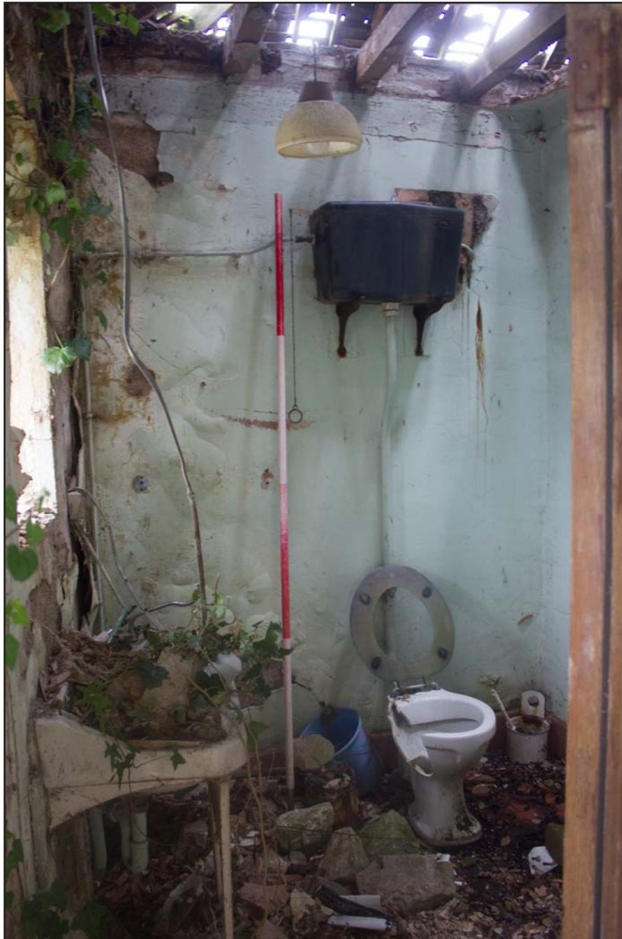
Plate 35: Office Toilet , Estate Offices & Stables, Trevor Road, Chirk - from the south - 2.00m scale
