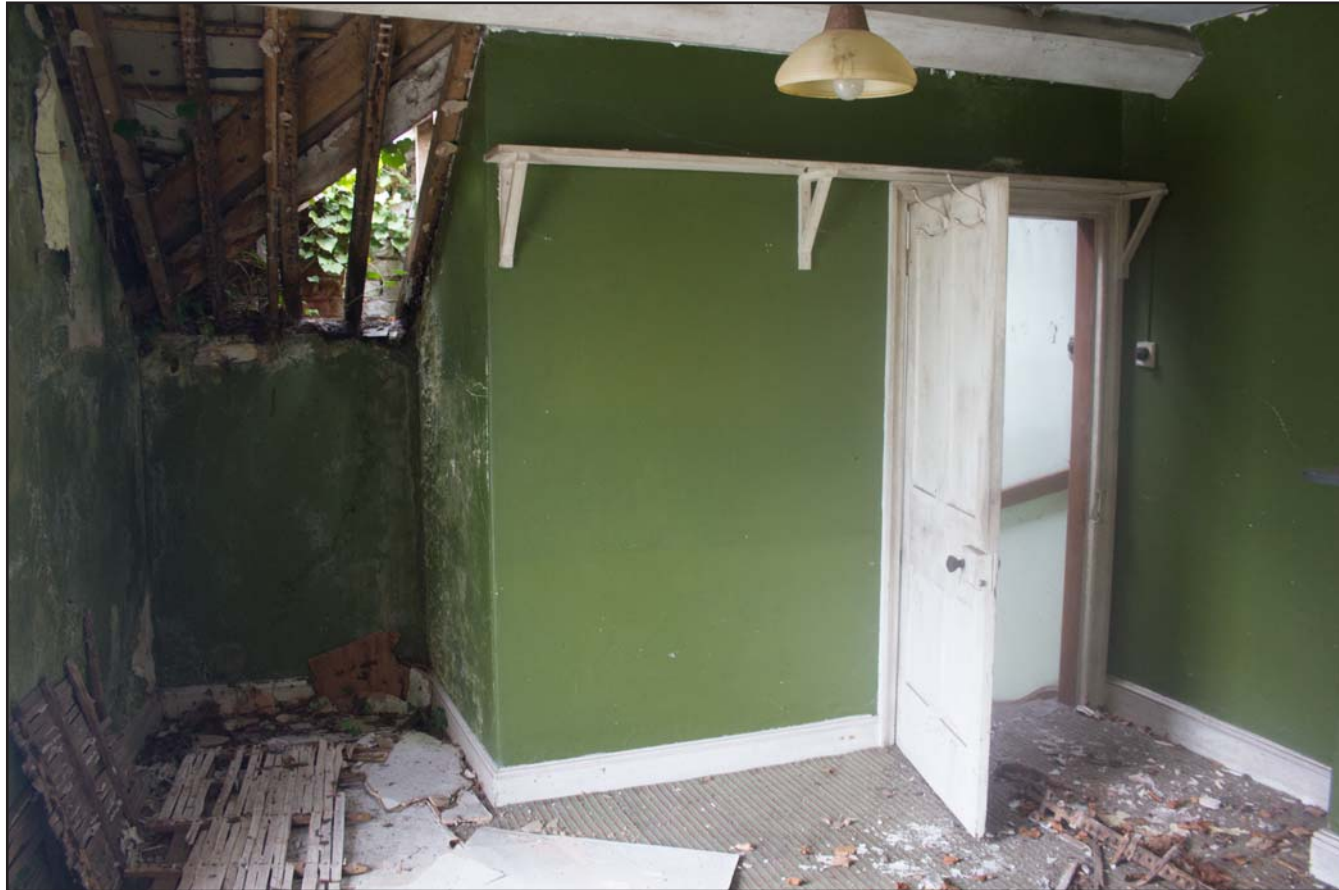
Plate 40: Internal shot of First Floor Office, Estate Offices & Stables, Trevor Road, Chirk - from the southwest - no scale
