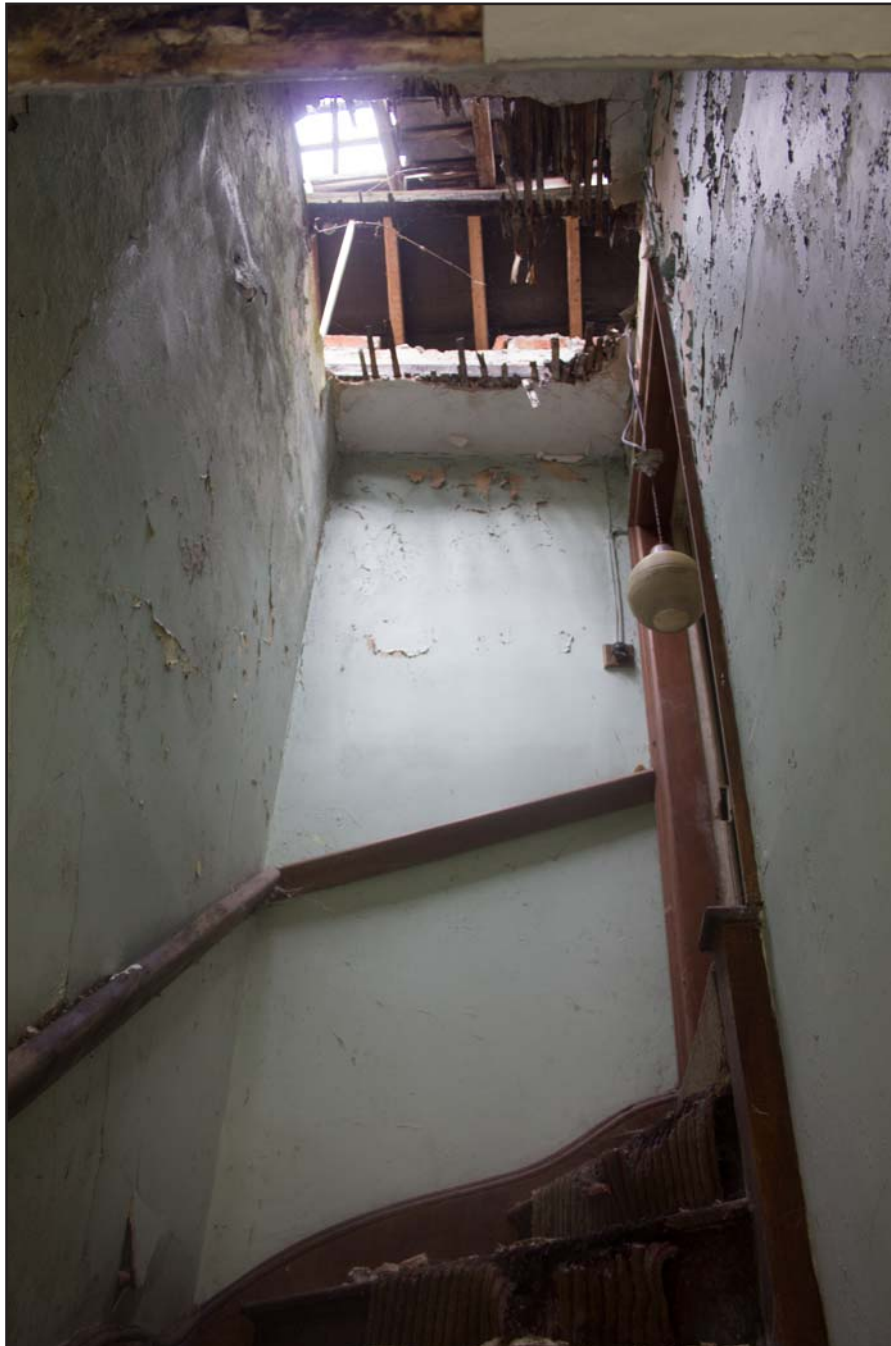
Plate 42: Staircase to First Floor Office - Fireplace, Estate Offices & Stables, Trevor Road, Chirk - from the west - no scale
