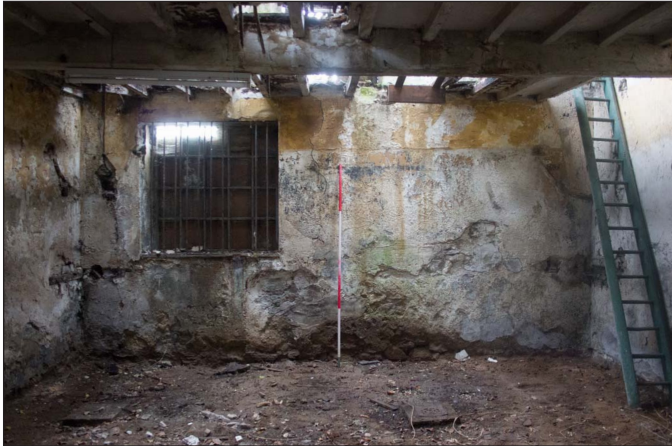
Plate 26: Internal shot of stables, Estate Offices & Stables, Trevor Road, Chirk - from the south - 2.00m scale
