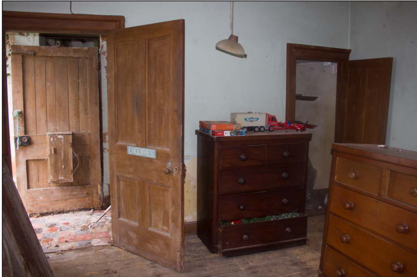
Plate 37: Internal shot of Enquiries Office, Estate Offices & Stables, Trevor Road, Chirk - from the southwest - no scale
