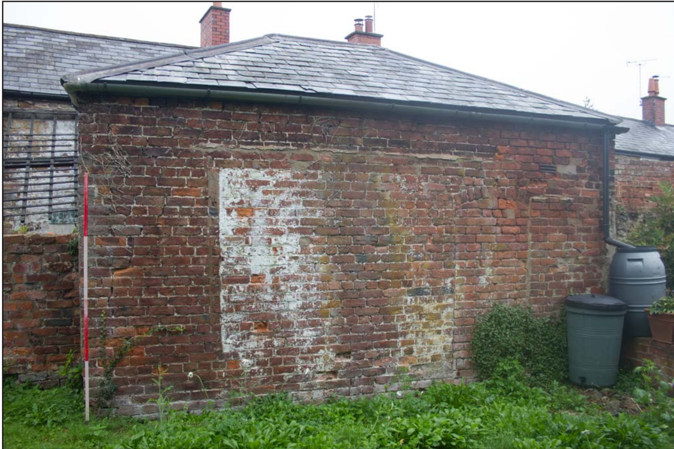
Plate 22: Southern elevation Garage, former Estate Offices & Stables, Trevor Road, Chirk - from the south - 2.00m scale
