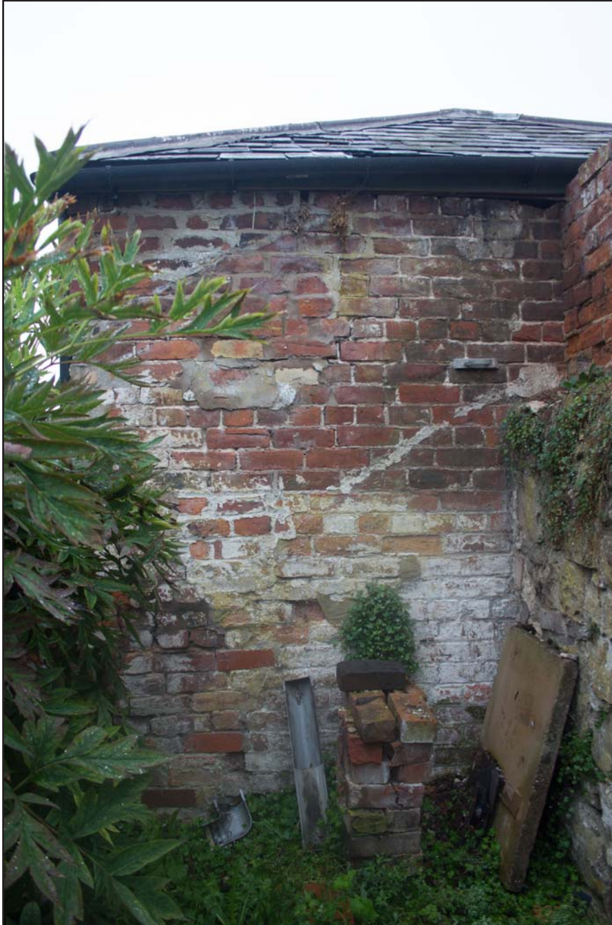
Plate 23: Eastern elevation Garage, former Estate Offices & Stables, Trevor Road, Chirk - from the east - 2.00m scale
