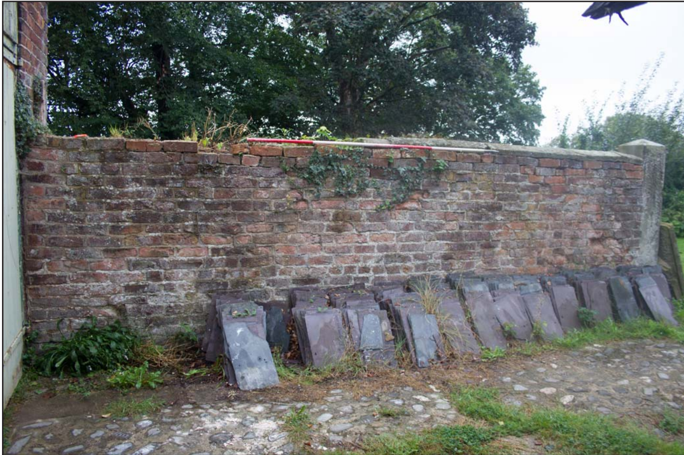
Plate 18: Garden Wall, former Estate Offices & Stables, Trevor Road, Chirk - from the northeast - 2.00m scale
