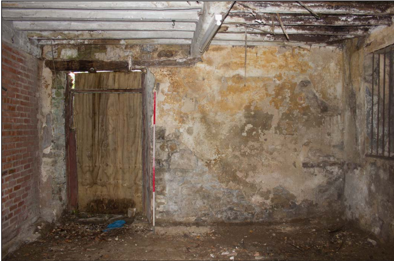
Plate 28: Internal shot of stables, Estate Offices & Stables, Trevor Road, Chirk - from the east - 2.00m scale
