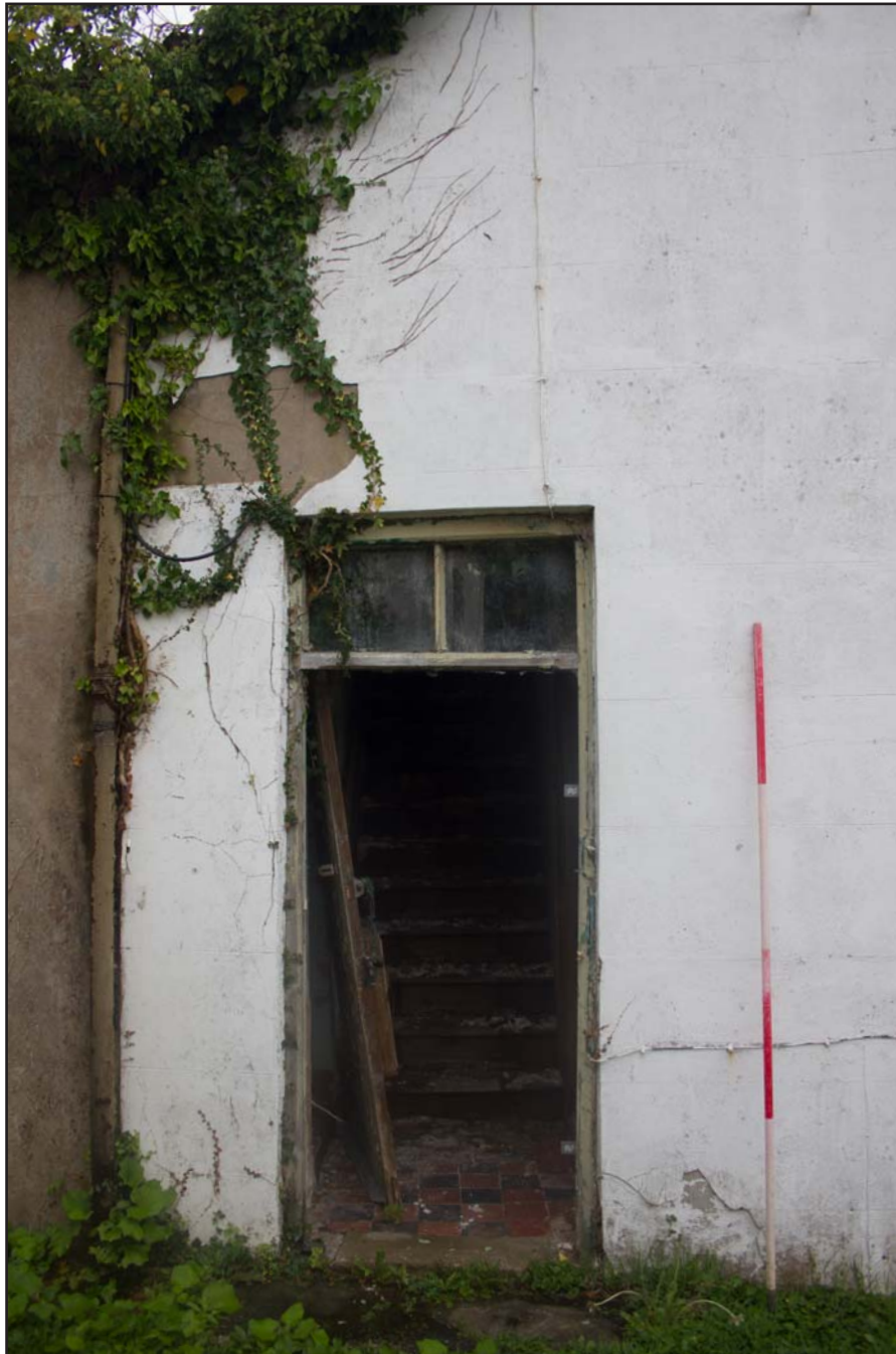
Plate 08: Western elevation (left), Office Entrance, former Estate Offices & Stables, Trevor Road, Chirk - from the west - 2.00m scale
