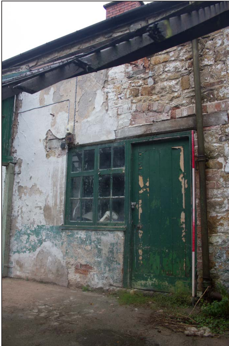
Plate 16: Workshop elevation (left), former Estate Offices & Stables, Trevor Road, Chirk - from the southeast - 2.00m scale
