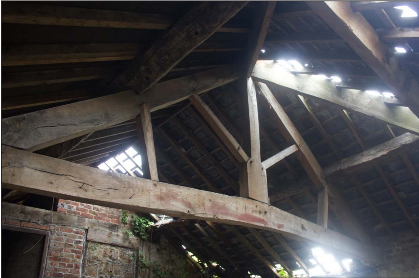
Plate 46: Internal shot of Hayloft, King's Post Truss, Estate Offices & Stables, Trevor Road, Chirk - from the northeast - no scale
