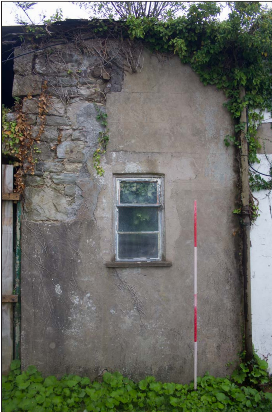
Plate 07: Western elevation (right), stables, former Estate Offices & Stables, Trevor Road, Chirk - from the west - 2.00m scale
