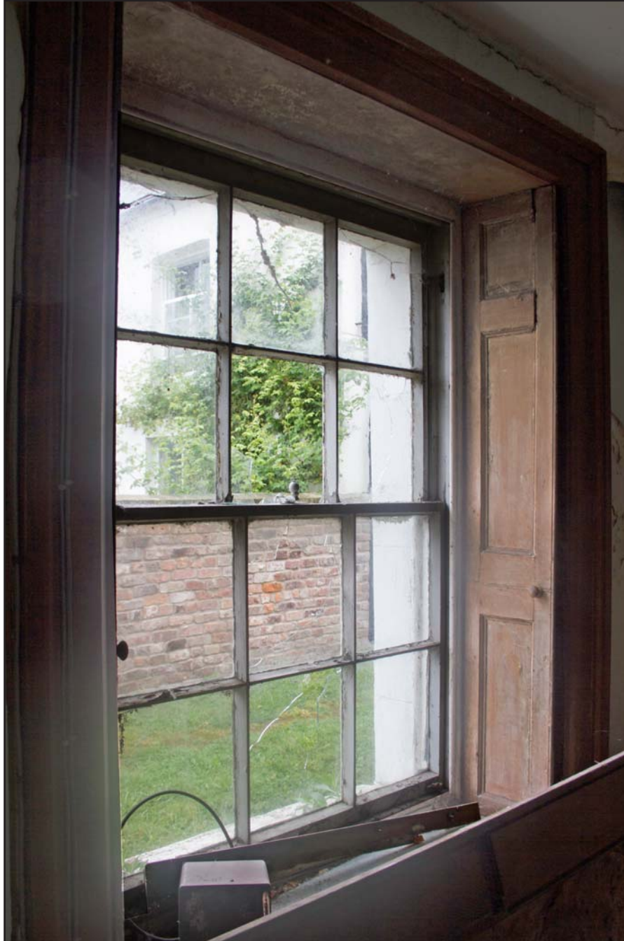
Plate 38: Internal shot of Enquiries Office - sash window, Estate Offices & Stables, Trevor Road, Chirk - from the southeast - no scale
