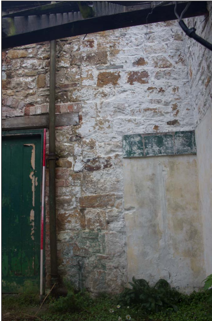
Plate 17: Workshop elevation (right), former Estate Offices & Stables, Trevor Road, Chirk - from the south - 2.00m scale
