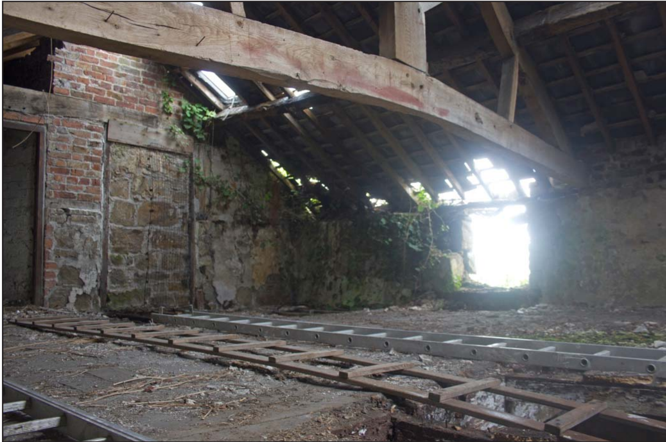
Plate 44: Internal shot of Hayloft, Estate Offices & Stables, Trevor Road, Chirk - from the northeast - no scale
