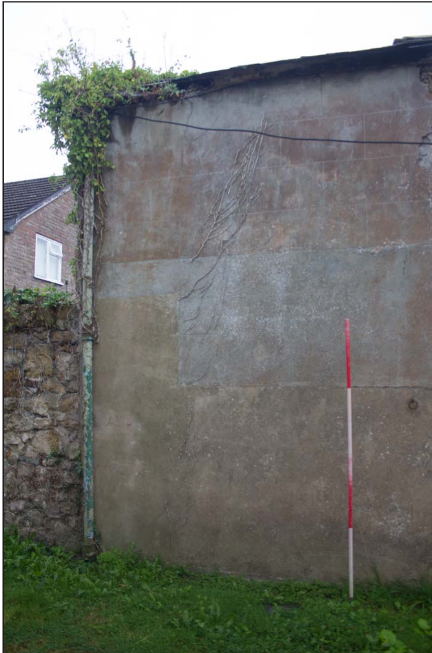
Plate 05: Western elevation (left), stables, former Estate Offices & Stables, Trevor Road, Chirk - from the west - 2.00m scale
