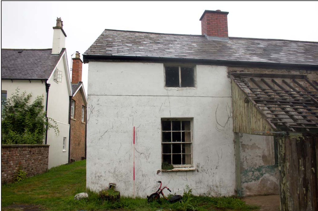
Plate 13: Southern elevation (left), Estate Office, former Estate Offices & Stables, Trevor Road, Chirk - from the south - 2.00m scale
