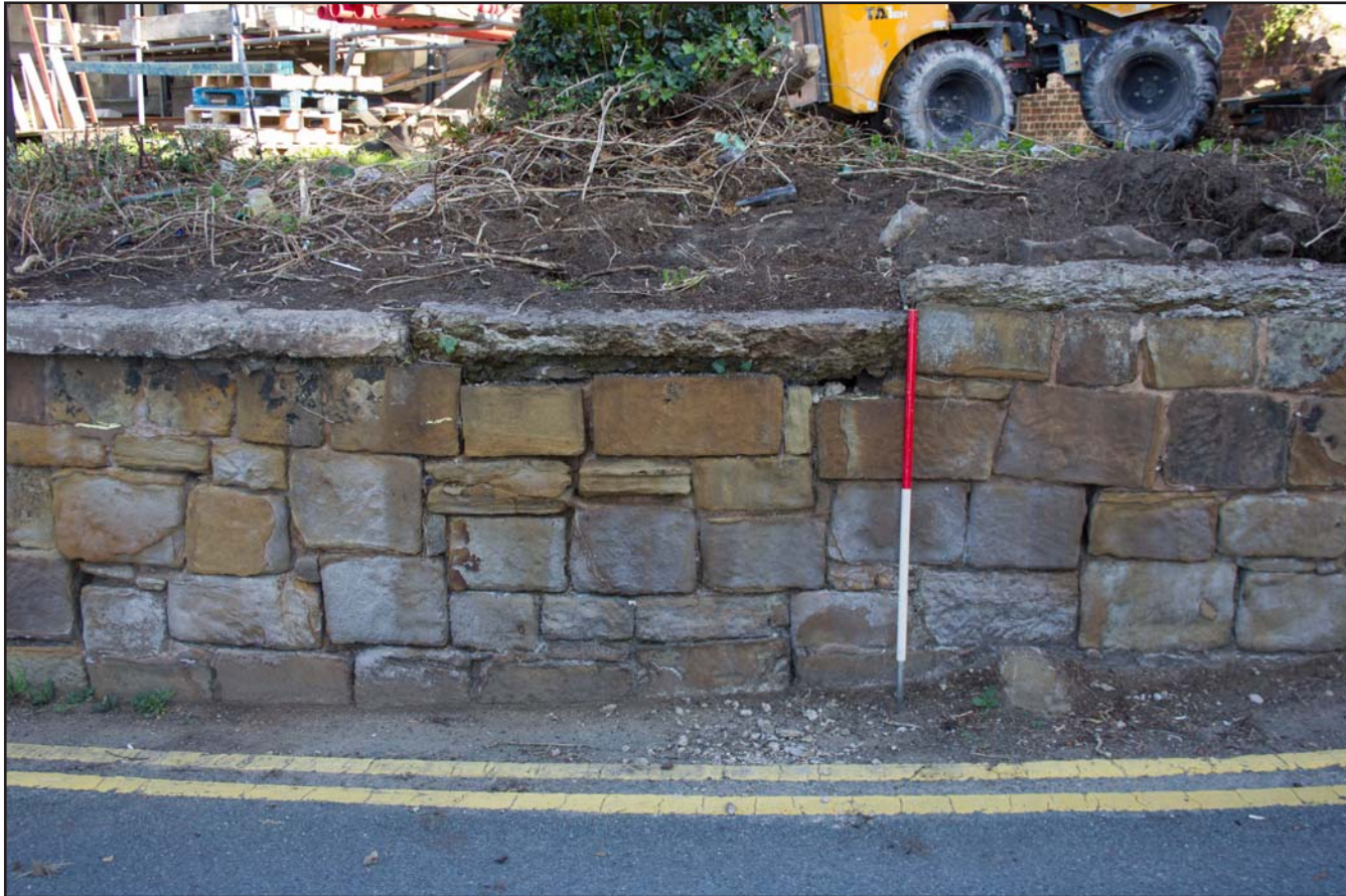
Plate 10: Fron Deg boundary wall showing blocked entrance, from the south. Scale 1.0m.
