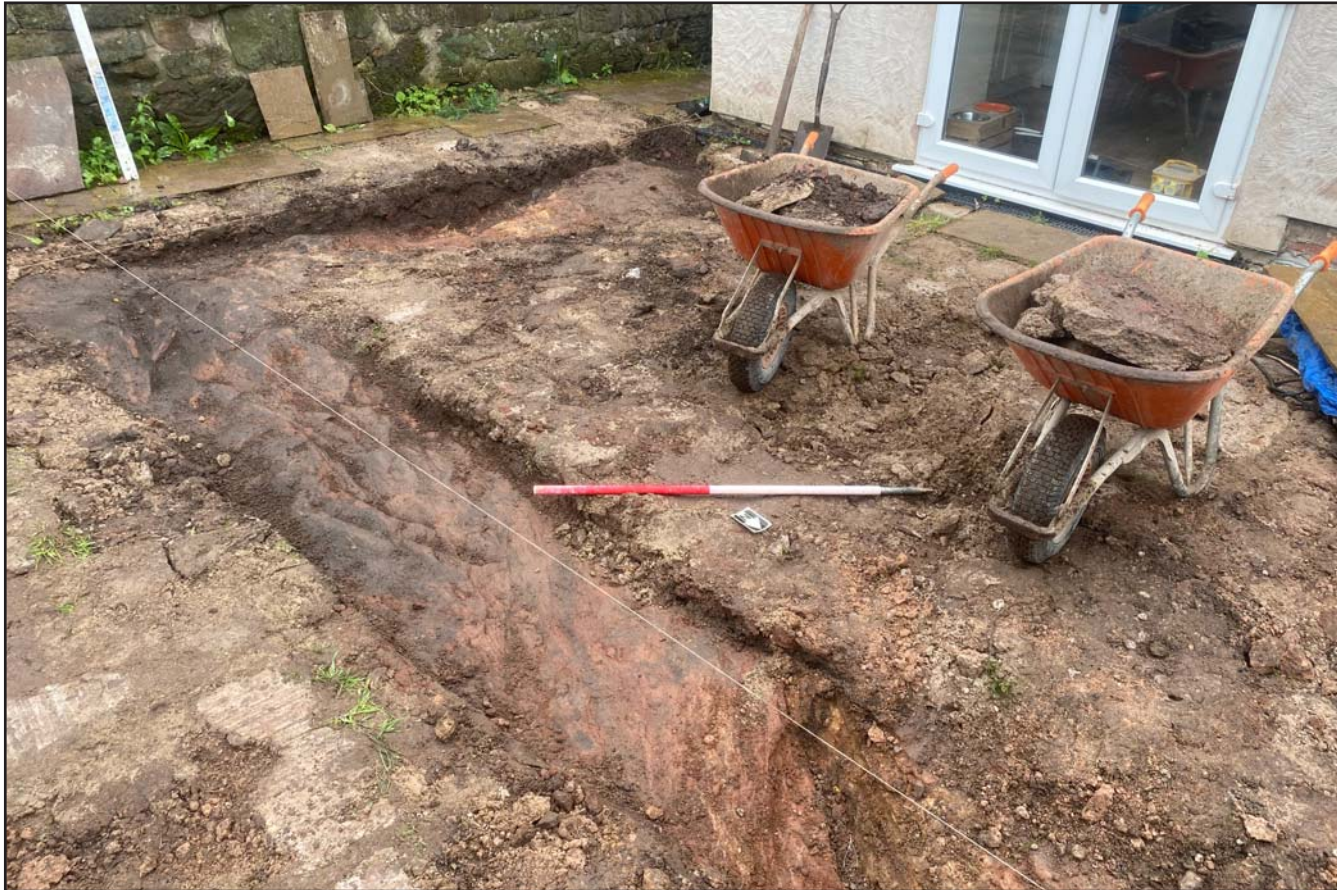
Plate 10: Post excavation shot of site, on land to rear of Rose Avon, Bridge Street, Holt, Wrexham - from the northeast - 1.00m scale
