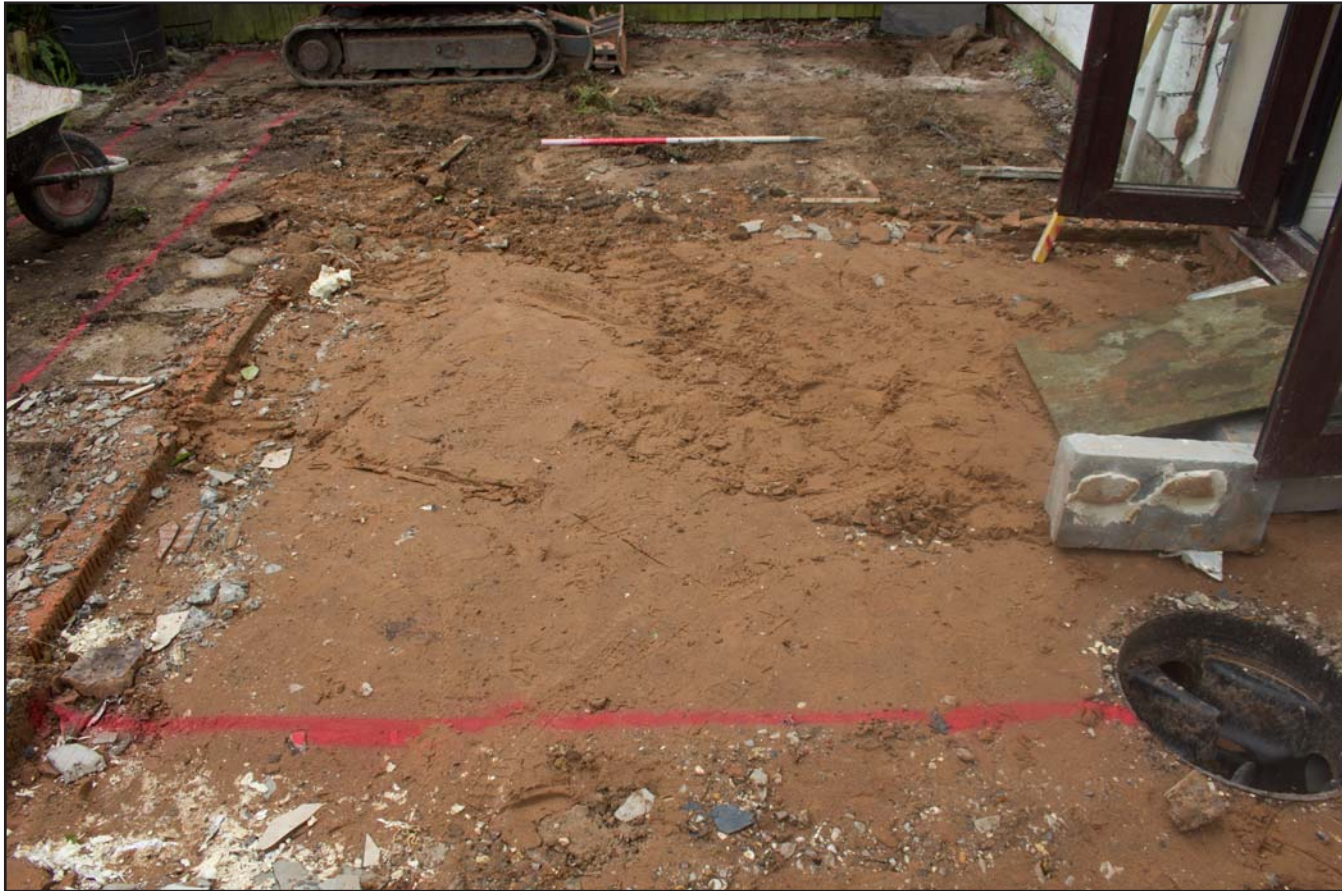
Plate 01: Pre excavation shot of site, Holm Lea, Church Street, Holt, Wrexham - from the north - 1.00m scale
