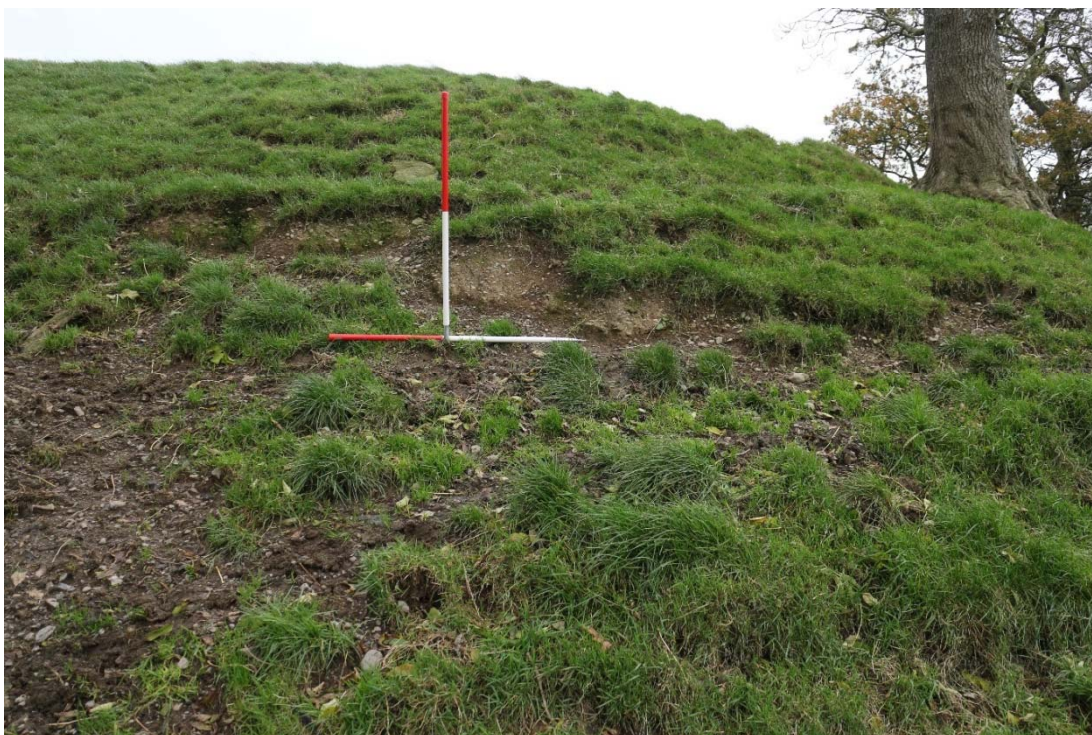
Prior to repair, IMG_2523, 22.10.2014
