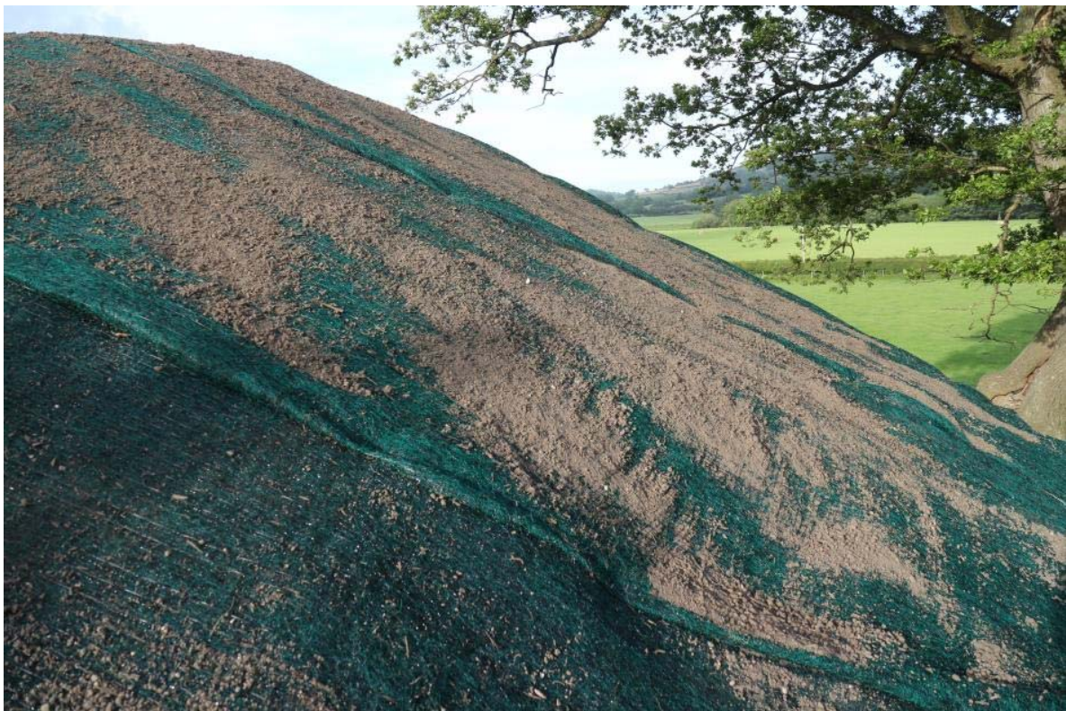
Western Excelsior Excel PP5-12 Turf Reinforcement Matting installed, top dressing with topsoil in progress, IMG_7288, 26.06,2015
