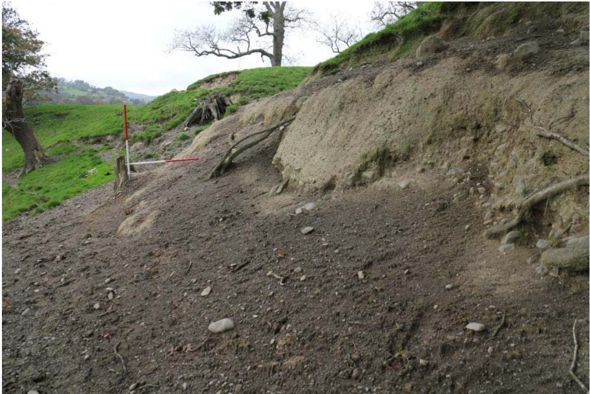
Prior to repair, IMG_2538, 22.10.2014
