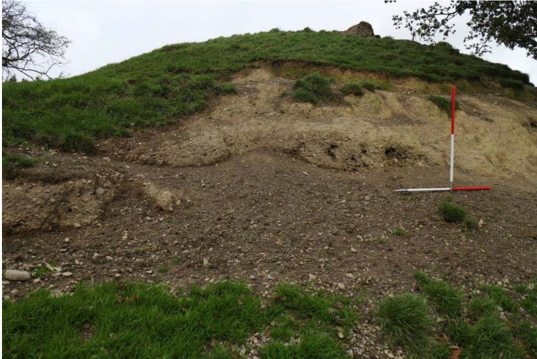
Prior to repair, IMG_2534, 22.10.2014
