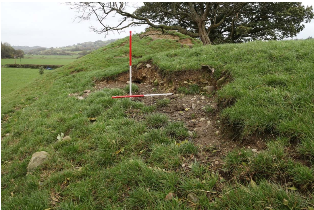
Prior to repair, IMG_2520, 22.10.2014
