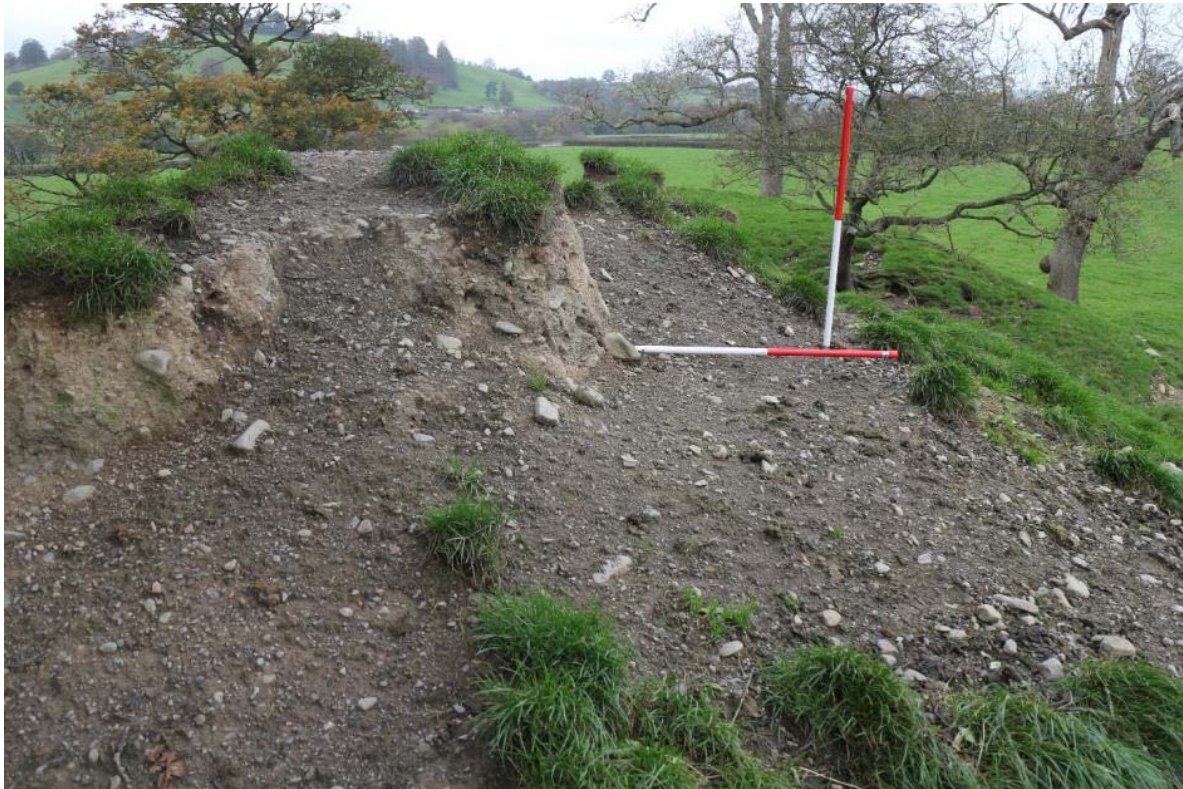
The motte summit, prior to repair, IMG_2526, 22.10.2014
