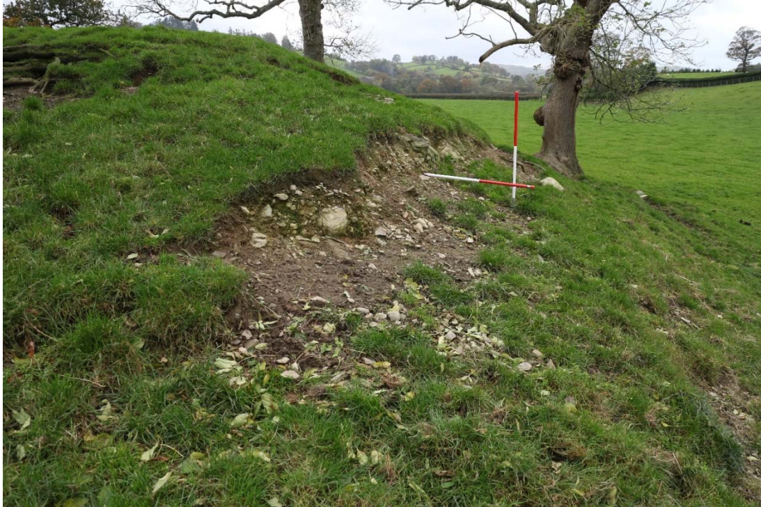
Prior to repair, IMG_2517, 22.10.2014
