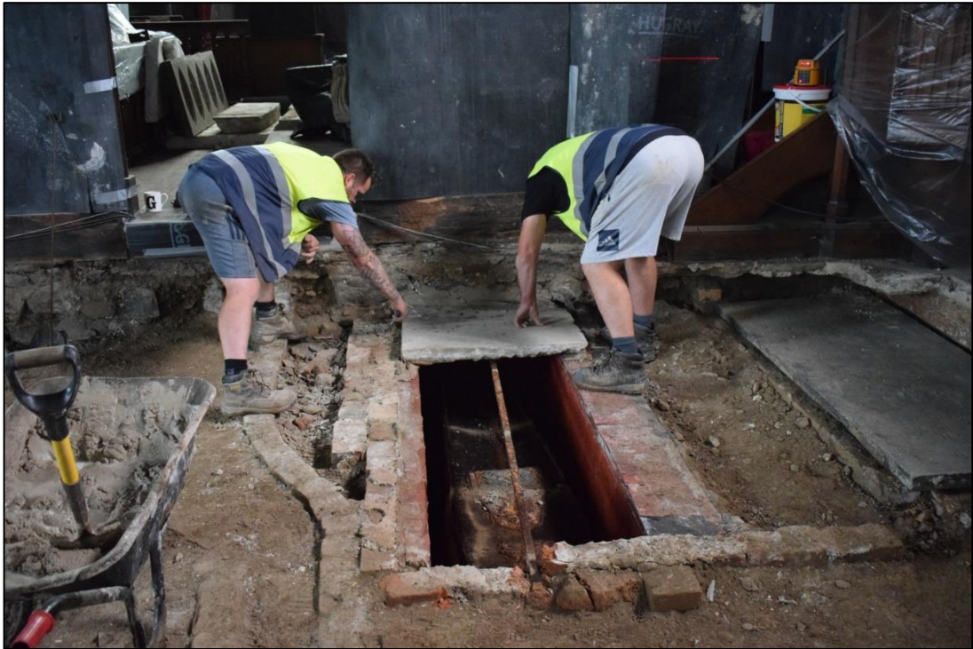
Fig. 12: The placement of the new capping stones over the north part of the vault. The ledger is in its lowered position. CPAT 4679-0105
