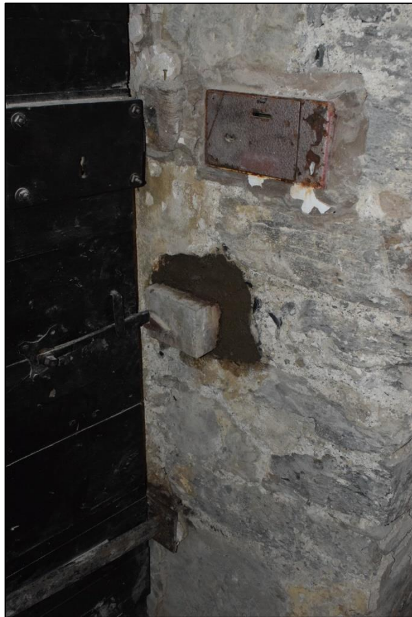
Fig. 23: The location of the (repointed) wooden drawbar slot on the external door of the chapel. CPAT 4679-0171
