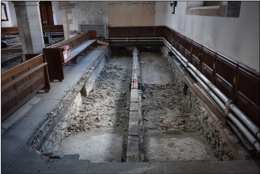
Fig. 2: The north aisle floor, showing the sleeper walls, from the east. CPAT 4679-0001
