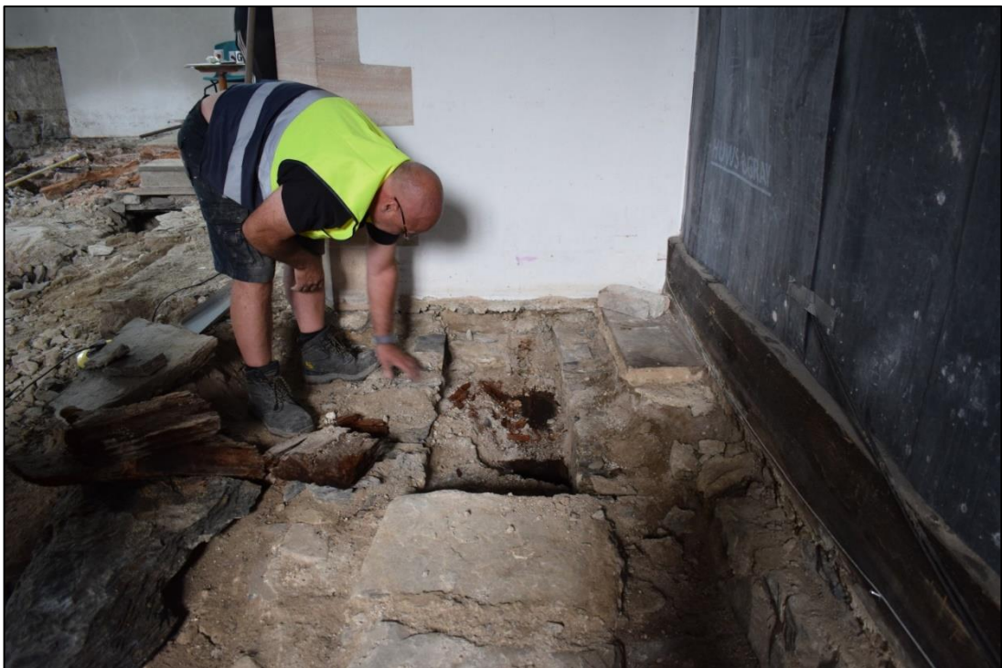
Fig. 9: The reduction in the height of the sleeper walls of Vault 2, prior to the setting in place of new covering slabs, from the south. CPAT 4679-0082
