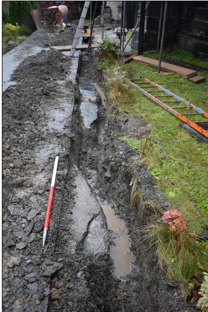
Fig. 25: Ledgers visible in the side of the trench for the waste pipe leading from the sewage treatment plant and following the line of the church path. CPAT 4679-0138
