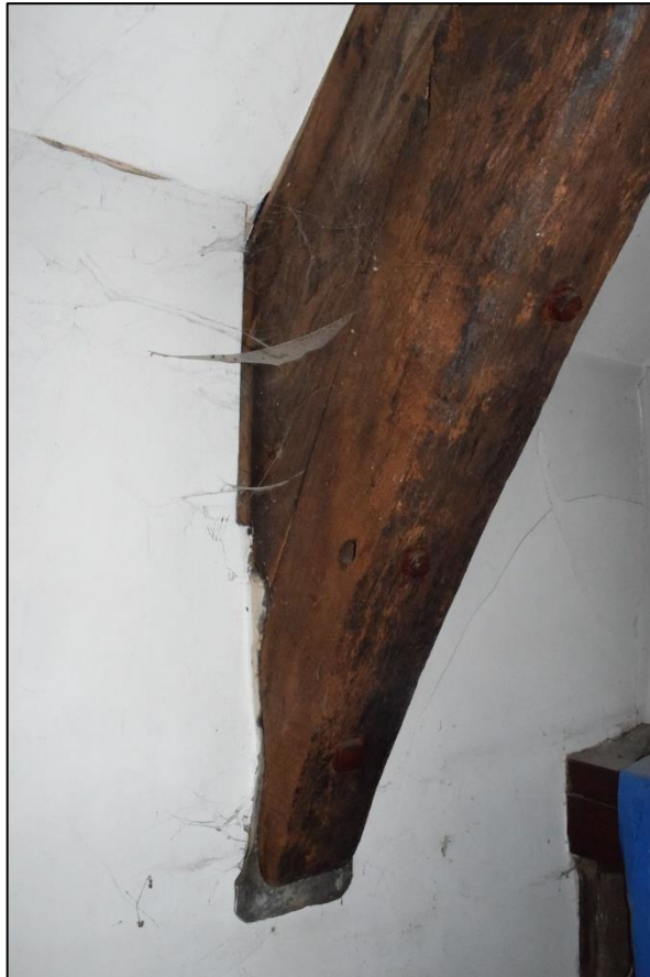
Fig. 17: The south side of the roof truss crossing the rood screen, showing bolted repair, from the north-east. CPAT 4679-0183
