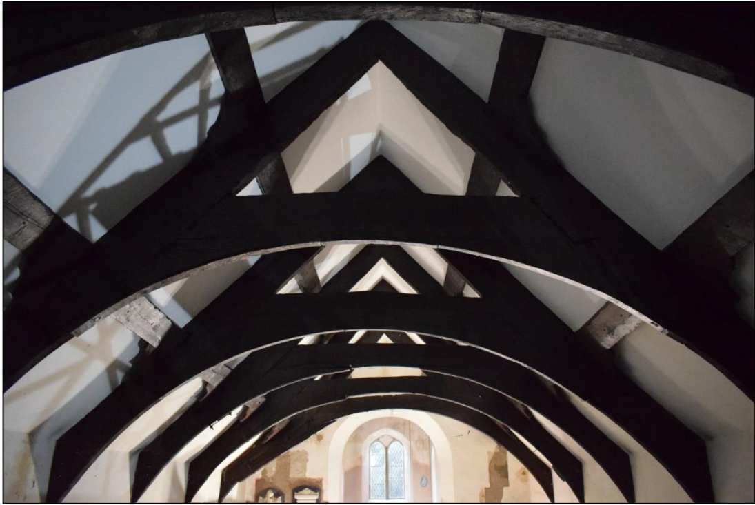
Fig. 16: The roof trusses in the nave taken from the top of the rood screen, from the east. CPAT 4679-0181
