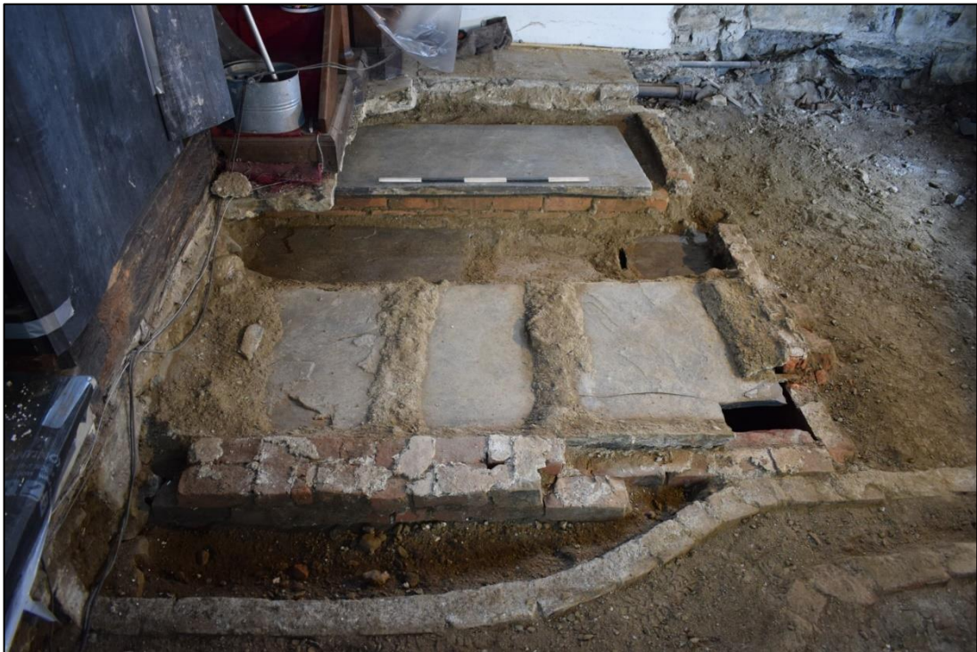
Fig. 10: Vault 3, adjoining the rood screen on the left, from the north. The ledger at the rear was as found, before it was lowered to allow the new floor to be installed. Note also the curved brick wall in the foreground, which is part of a duct associated with a 19 th -century heating system (see Fig. 13 and para 3.15). CPAT 4679-0091
